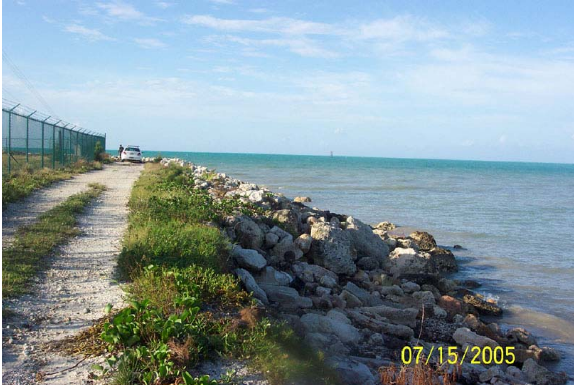
Photo 35. Revetment damage at U.S. Naval Station, Truman Annex (photo by Danielle Rogers, D.E.P.).
