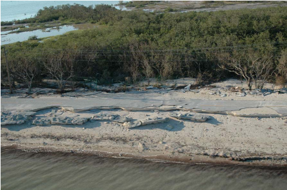
Photo 51. Boca Chica Beach Road damaged.
