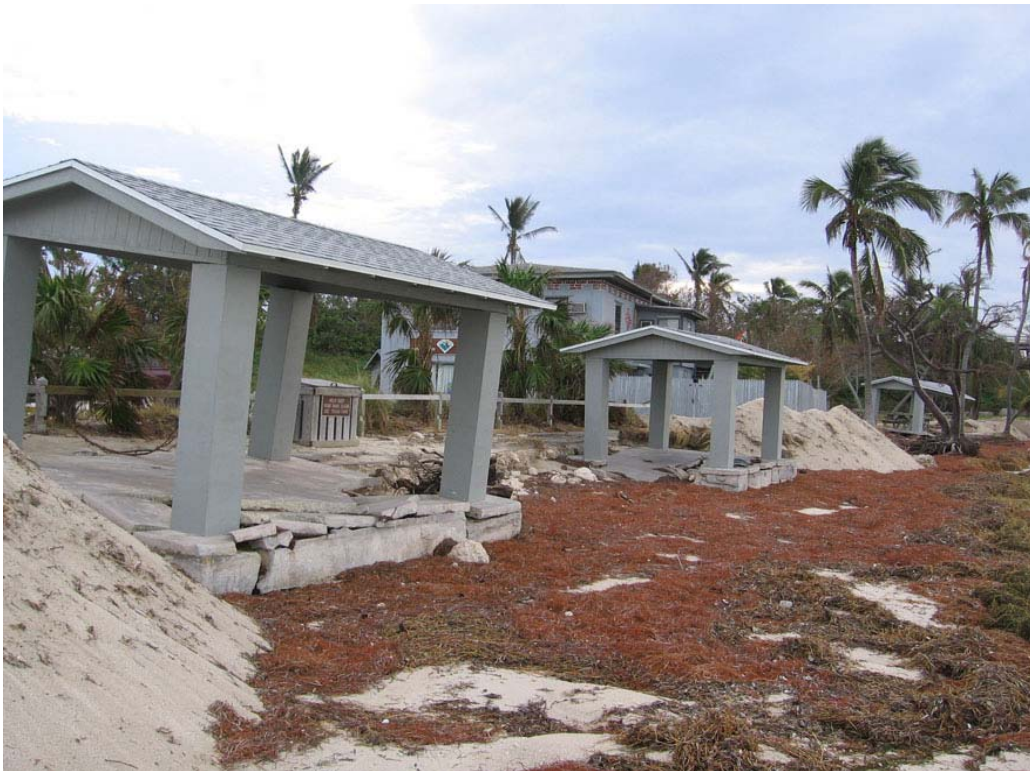
Photo 46. Destroyed picnic shelters, Calusa Beach (Hurricane Wilma).
