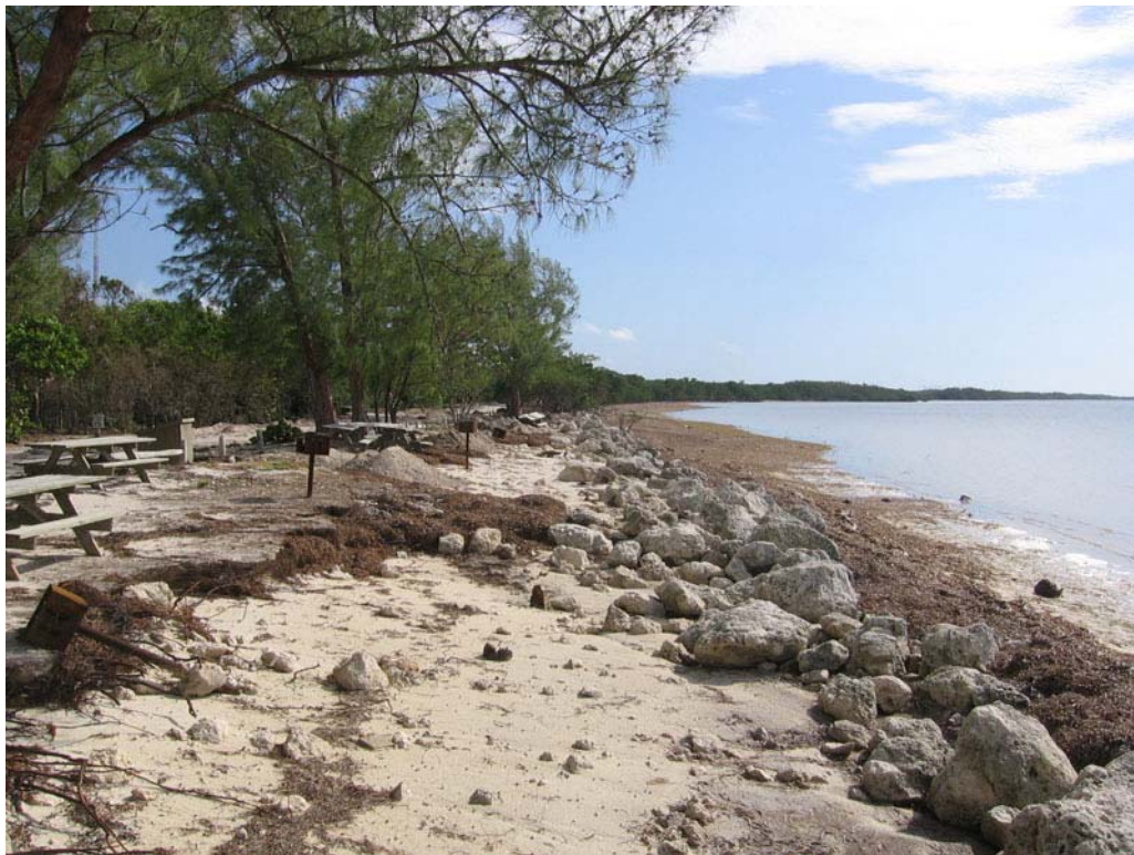
Photo 37. Revetment damaged by Rita at Long Key State Park.
