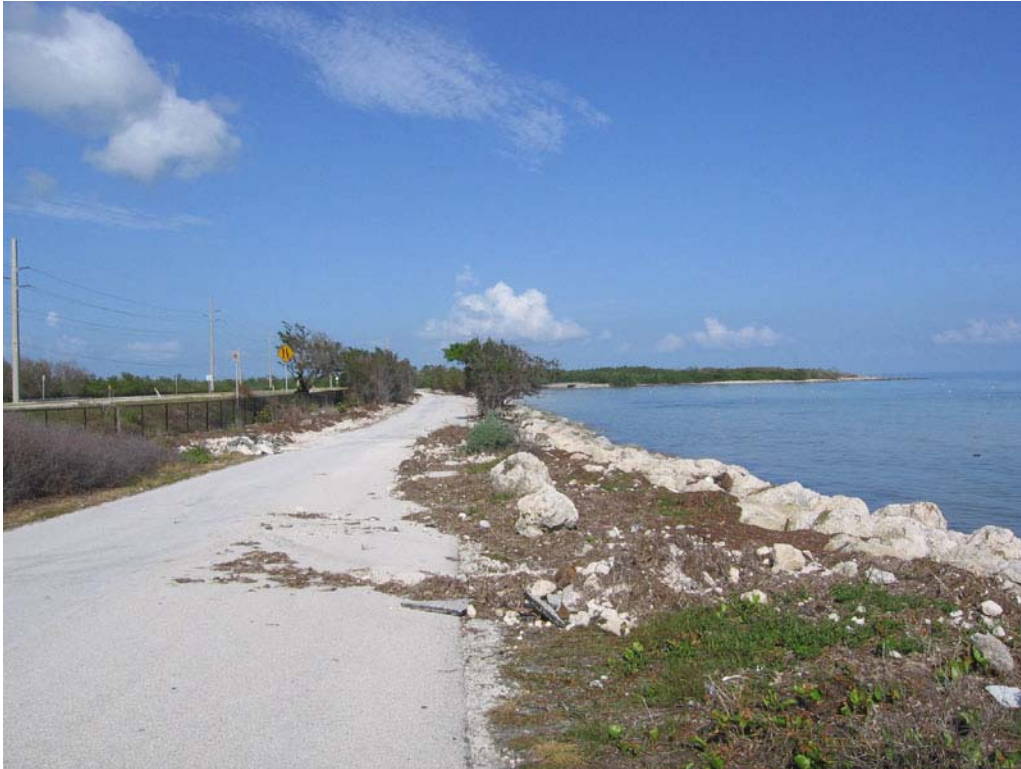
Photo 38. Revetment overtopped and damaged by Rita at Bahia Honda State Park.
