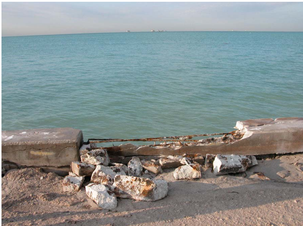
Photo 5. Concrete cap damage, Cape Florida.
