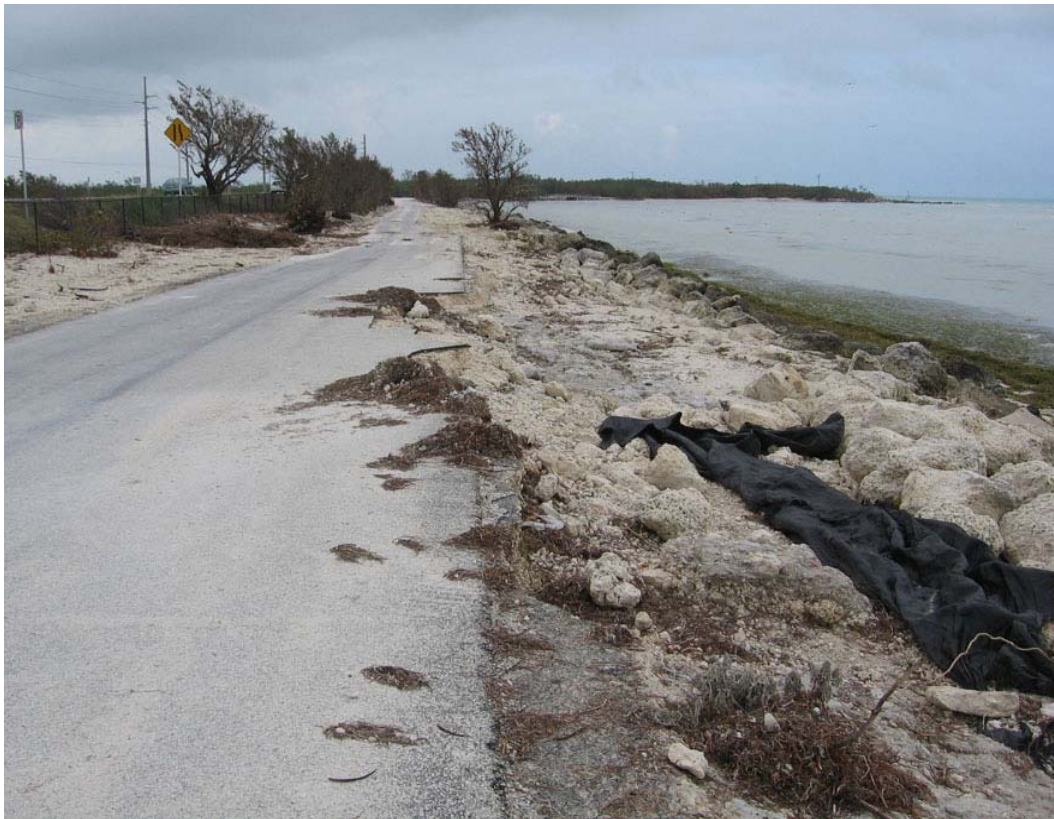
Photo 47. Road and revetment damage, Bahia Honda State Park (compare with Photo 38).
