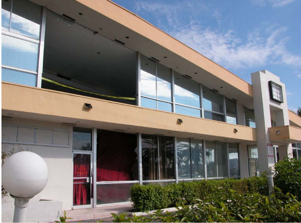
Photo 4. Broken windows, Golden Nugget Motel, Sunny Isles Beach.
