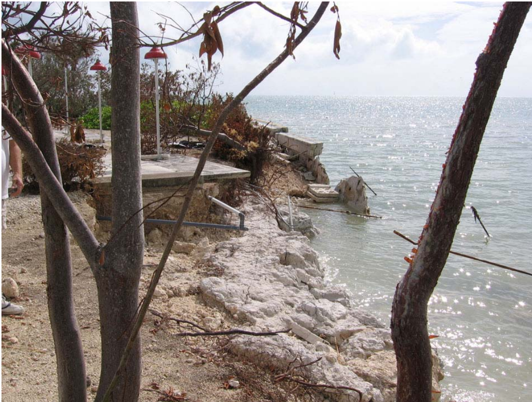
Photo 44. Seawall destroyed by Wilma, Tingler Island.
