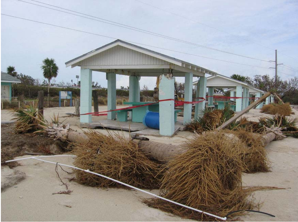
Photo 45. Damaged picnic shelter, Little Duck Key (Hurricane Wilma).
