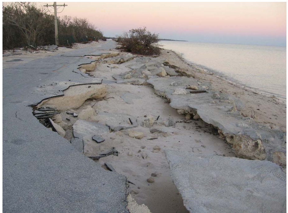
Photo 52. Boca Chica Beach Road damaged.
