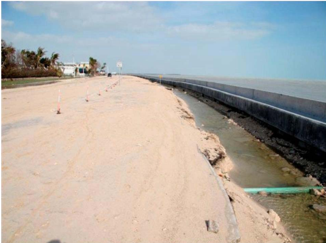
Photo 27. Scour behind seawall along South Roosevelt Boulevard (credit: City of Key West)
