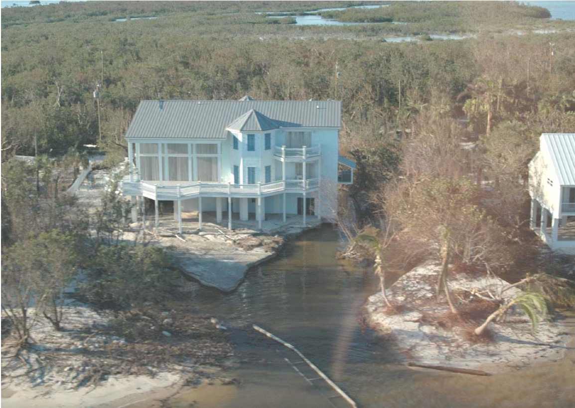
Photo 50. Imminently threatened dwelling, Sugarloaf Key (Hurricane Wilma).
