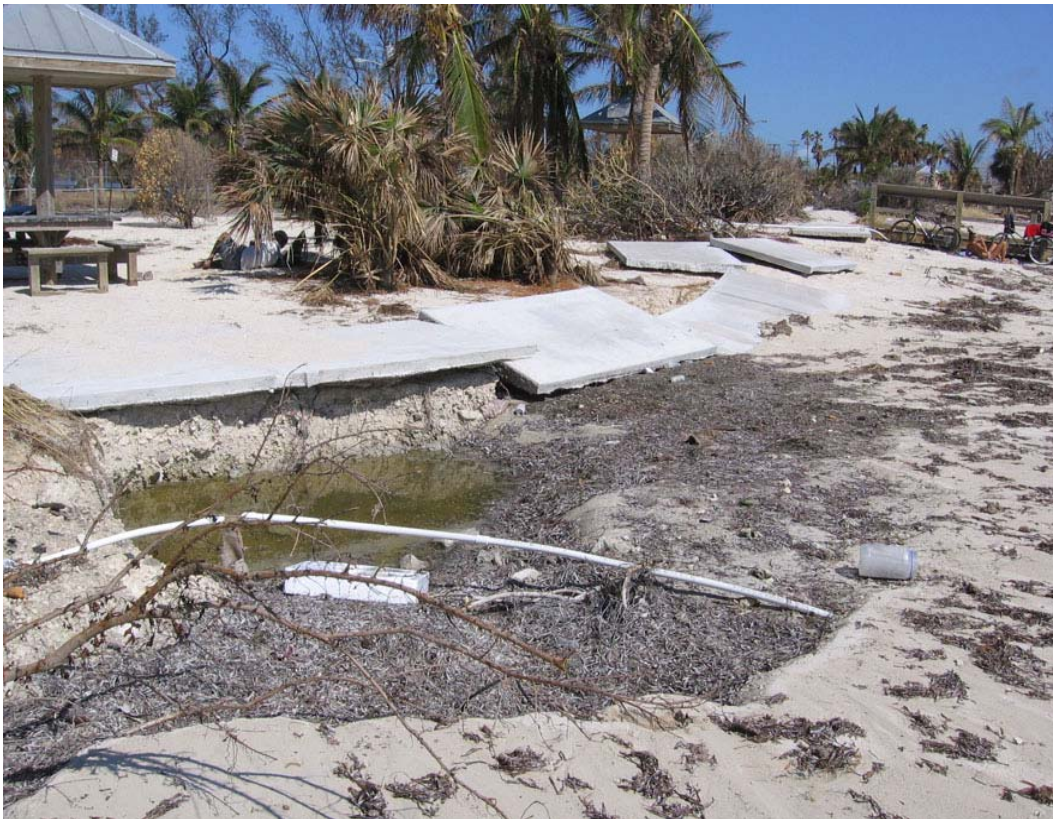
Photo 57. Damage to Rest Beach infrastructure by Hurricane Wilma.
