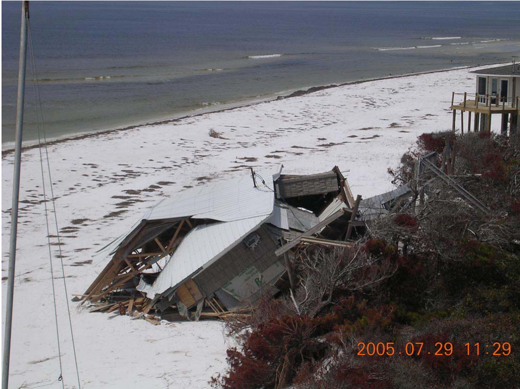
Photo 54. Dwelling destroyed, Dog Island (R169.7).
