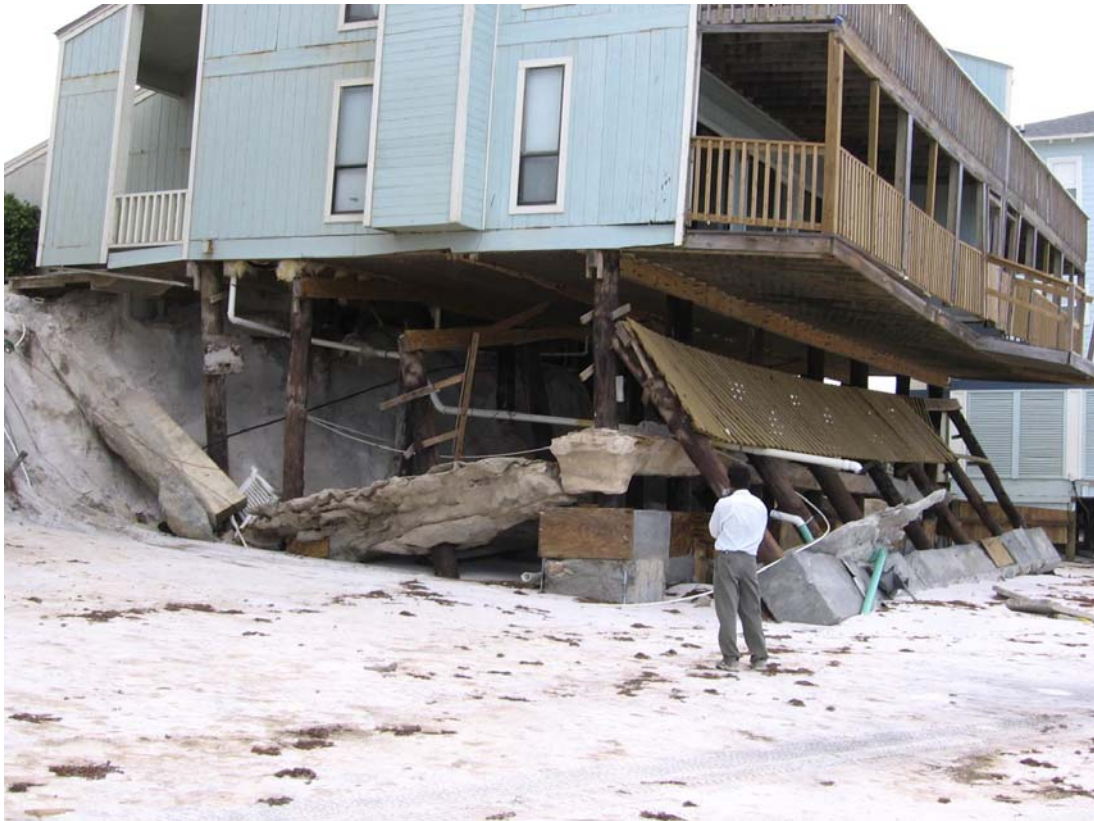
Photo 25. Damaged structure, Gulf Trace (R68).
