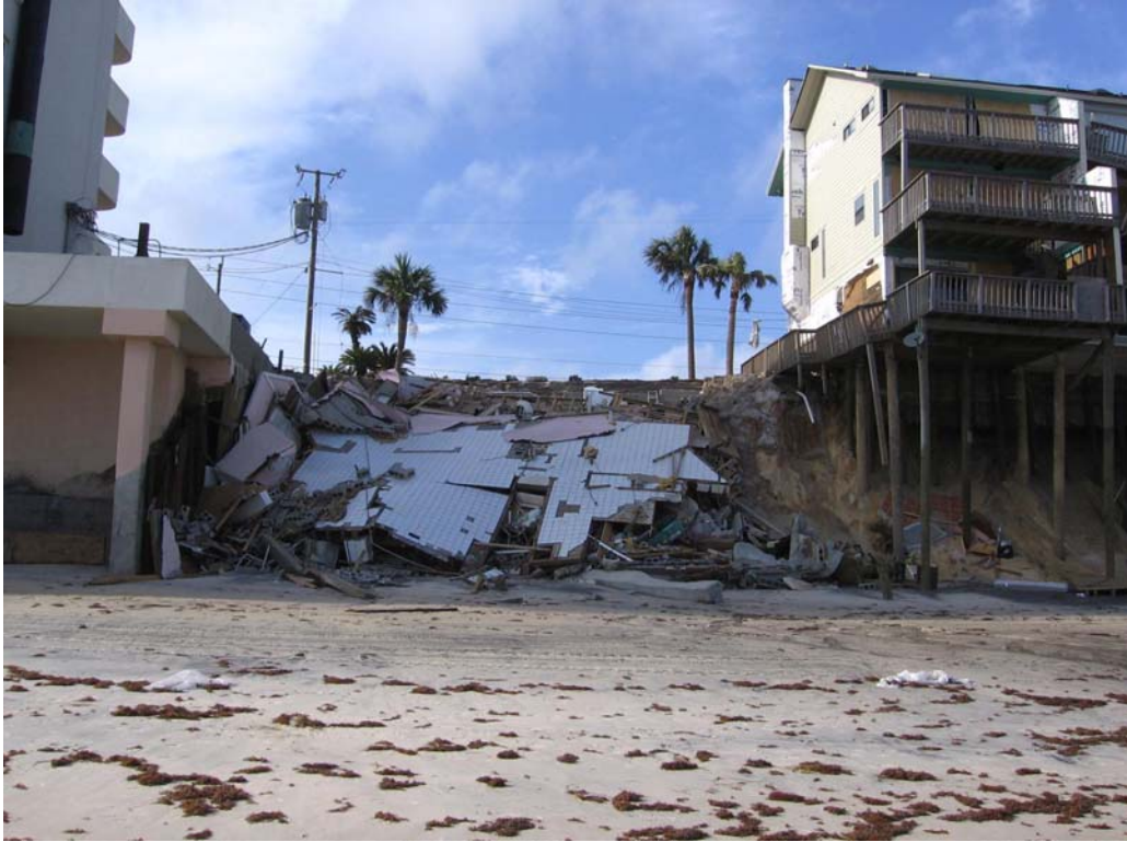
Photo 22. Single-family dwelling destroyed, Miramar Beach (R9).
