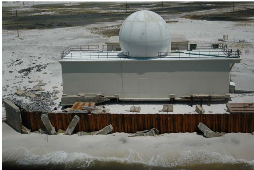
Photo 14. Destroyed seawall and damaged building foundation.
