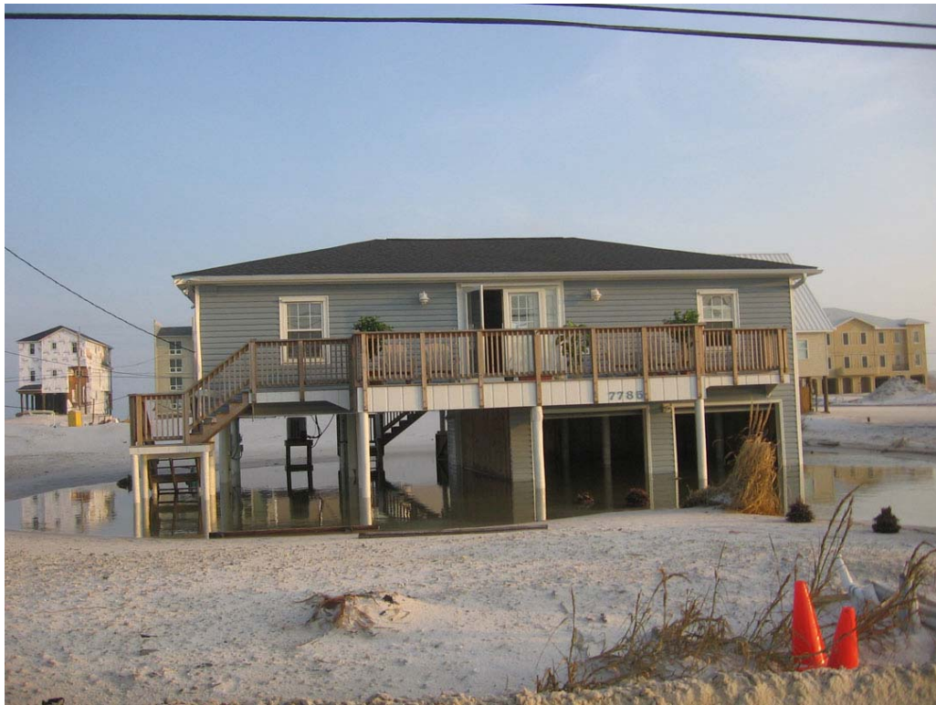
Photo 13. Dwelling with understructure flooding, Navarre Beach (R201.4).
