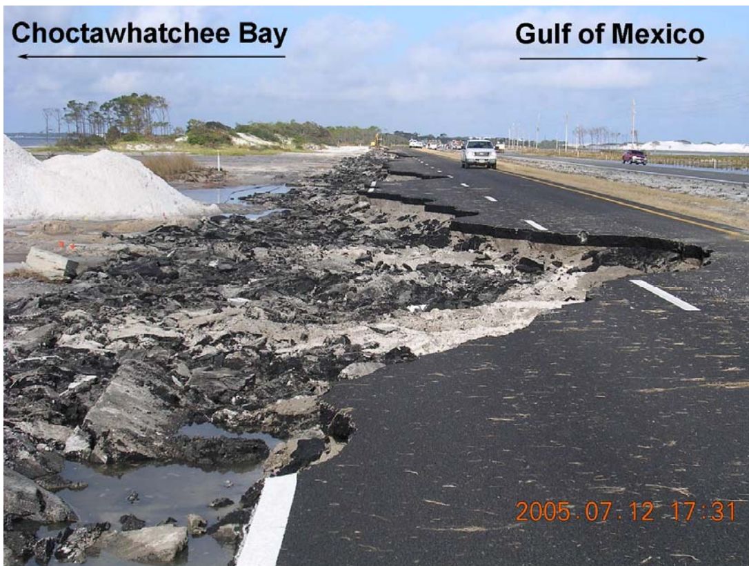
Photo 17. Damage to U.S. Highway 98 between Ft. Walton Beach and Destin (V606).
