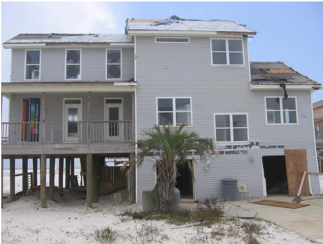
Photo 4. Dwelling with understructure damage, Pensacola Beach (R126.3).
