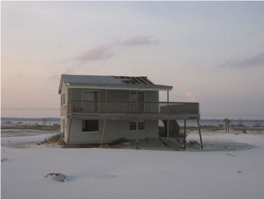
Photo 11. Dwelling destroyed, Navarre Beach (R196.2).
