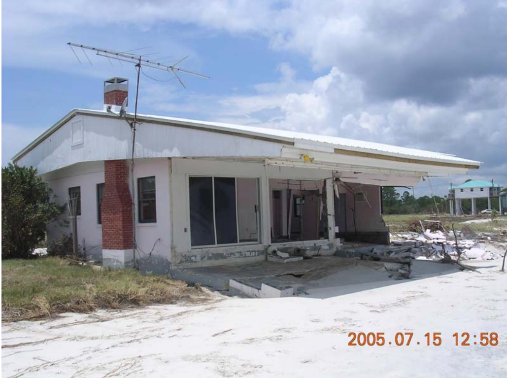
Photo 59. Dwelling destroyed near Bald Point (R132).
