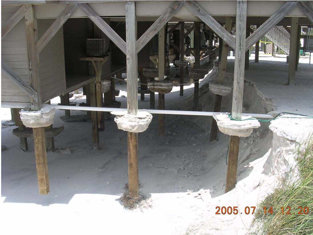
Photo 46. Undermined building with piles suspended, St. Joseph Peninsula (R90.8).
