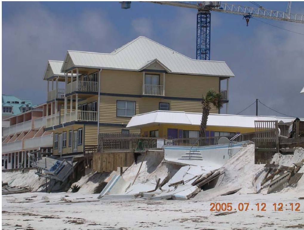
Photo 15. Destin erosion damage (R43.5).
