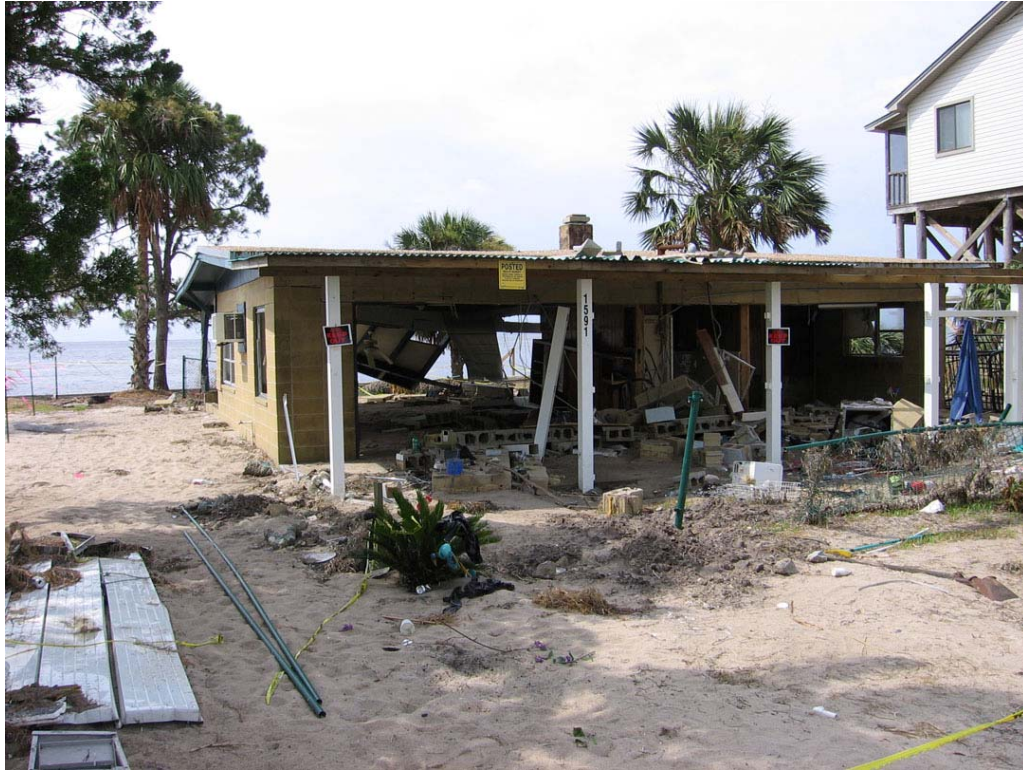
Photo 63. Dwelling destroyed, Shell Point (URS, 2005).
