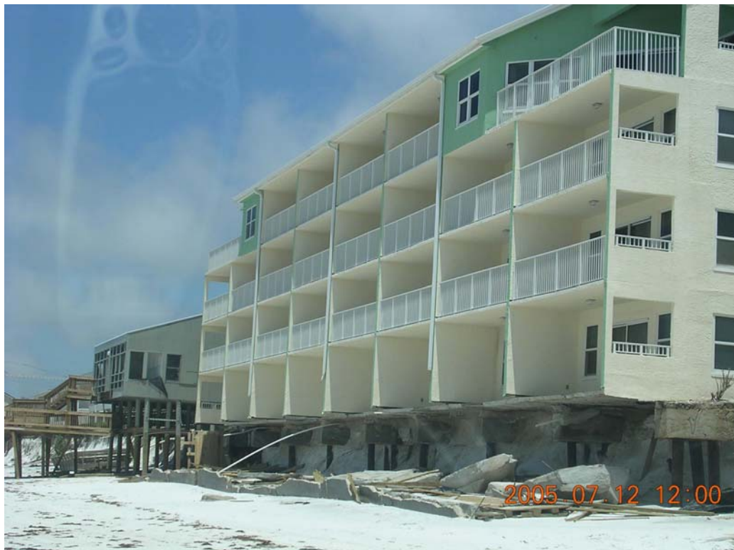
Photo 20. Concrete wall failure and building undermined, Destin (R45).
