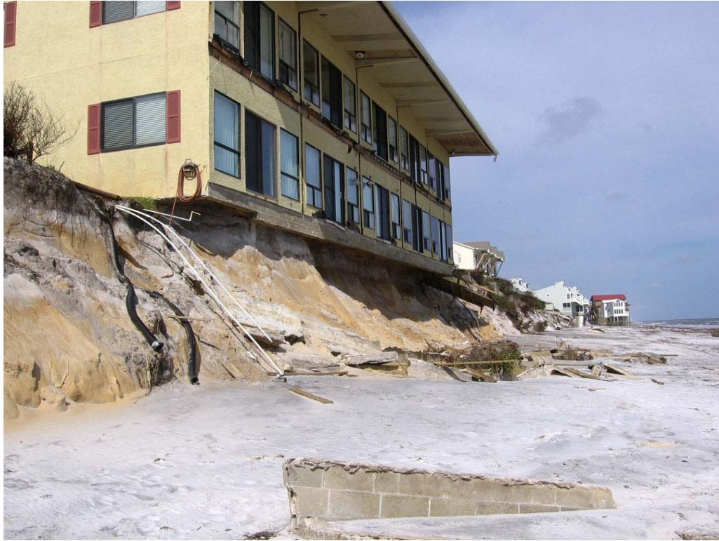
Photo 28. Condominium undermined by Dennis, Beach Highlands (R43.2).
