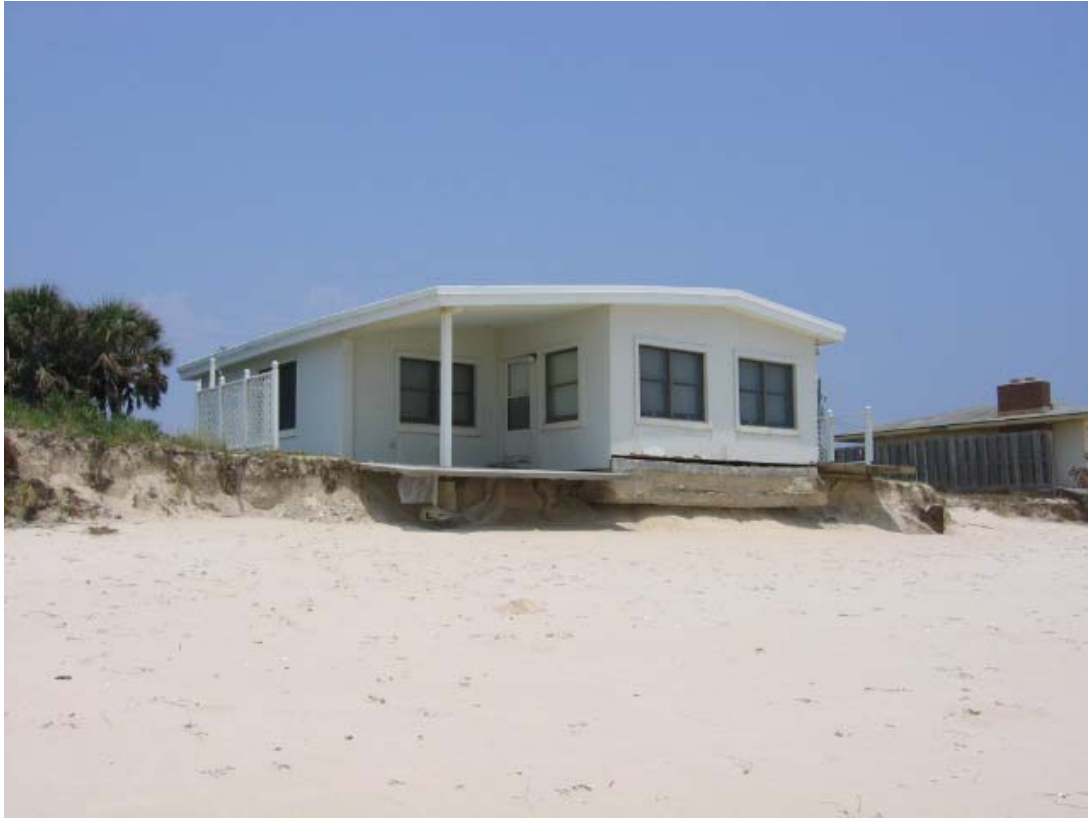
Photo 53. Foundation damage to dwelling, St. George Island (R80.3).
