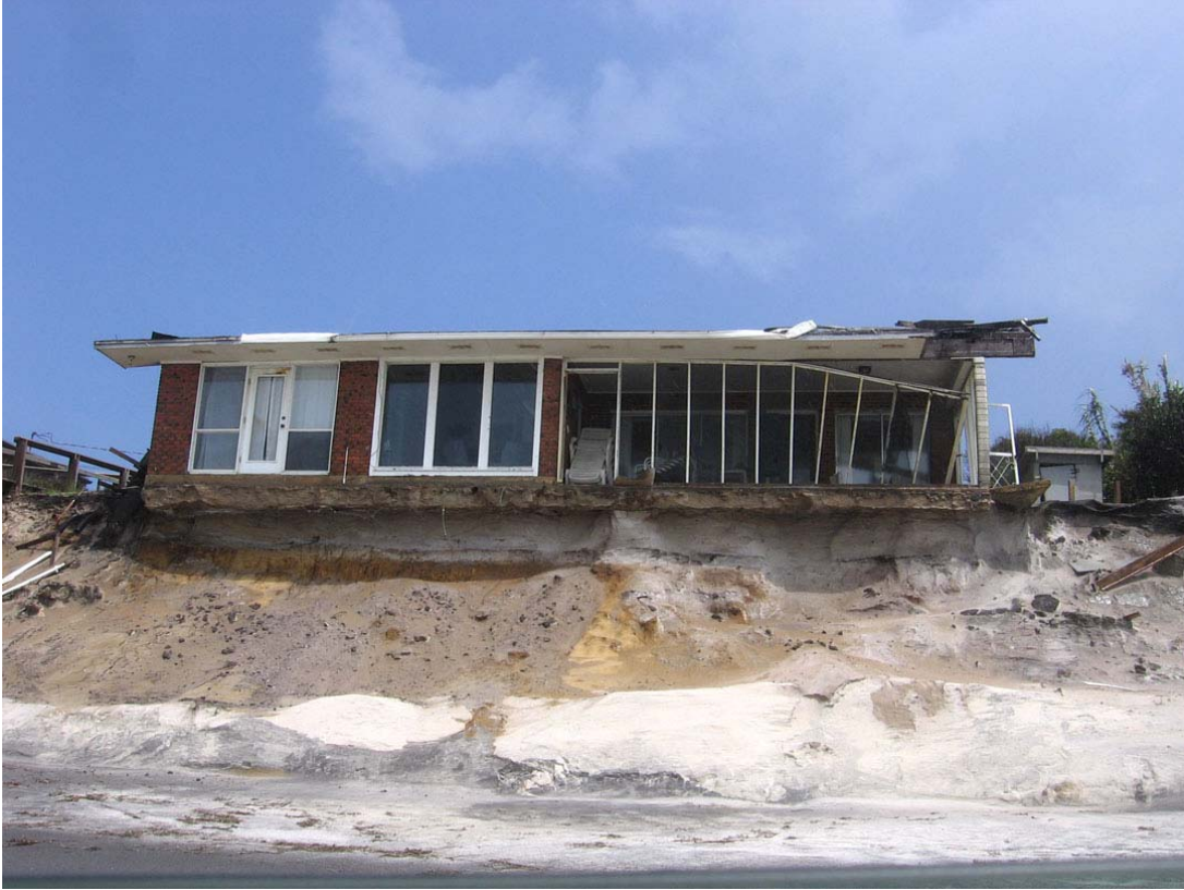
Photo 30. Dwelling undermined by Katrina, Dune Allen Beach (R49.9).
