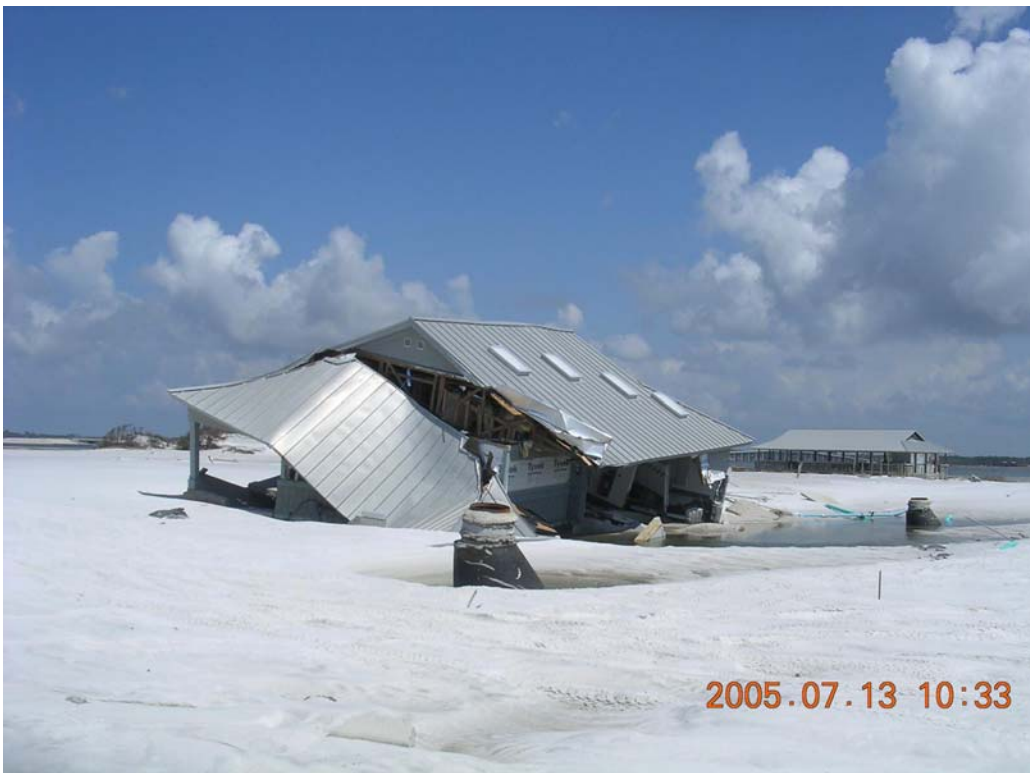
Photo 10. Bathhouse destroyed at Navarre Beach State Park (R213).
