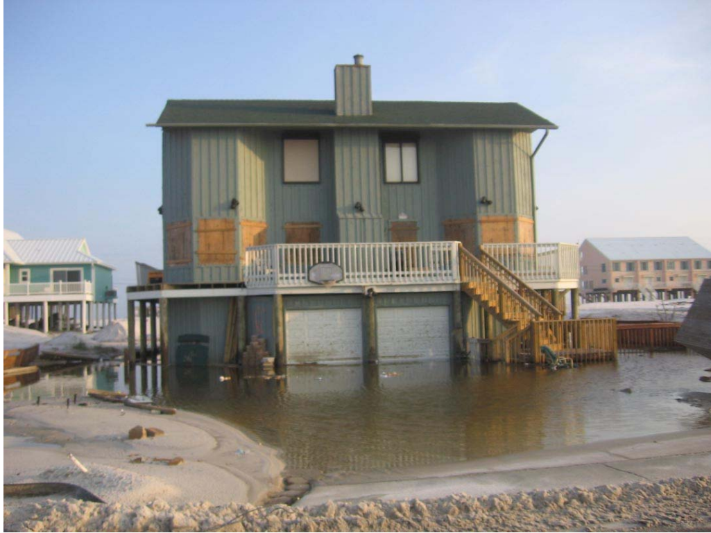
Photo 12. Dwelling with understructure flooding, Navarre Beach (R198.9).
