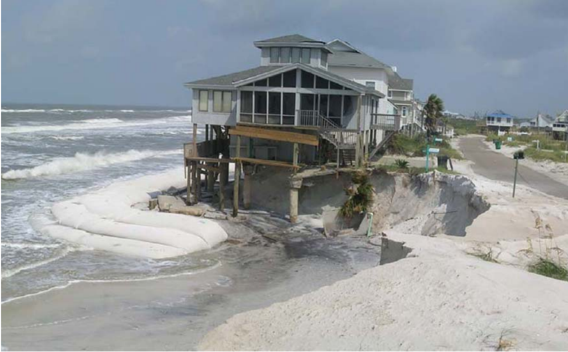
Photo 44. Dune erosion threatening Dunes Drive, St. Joseph Peninsula (R83.6).
