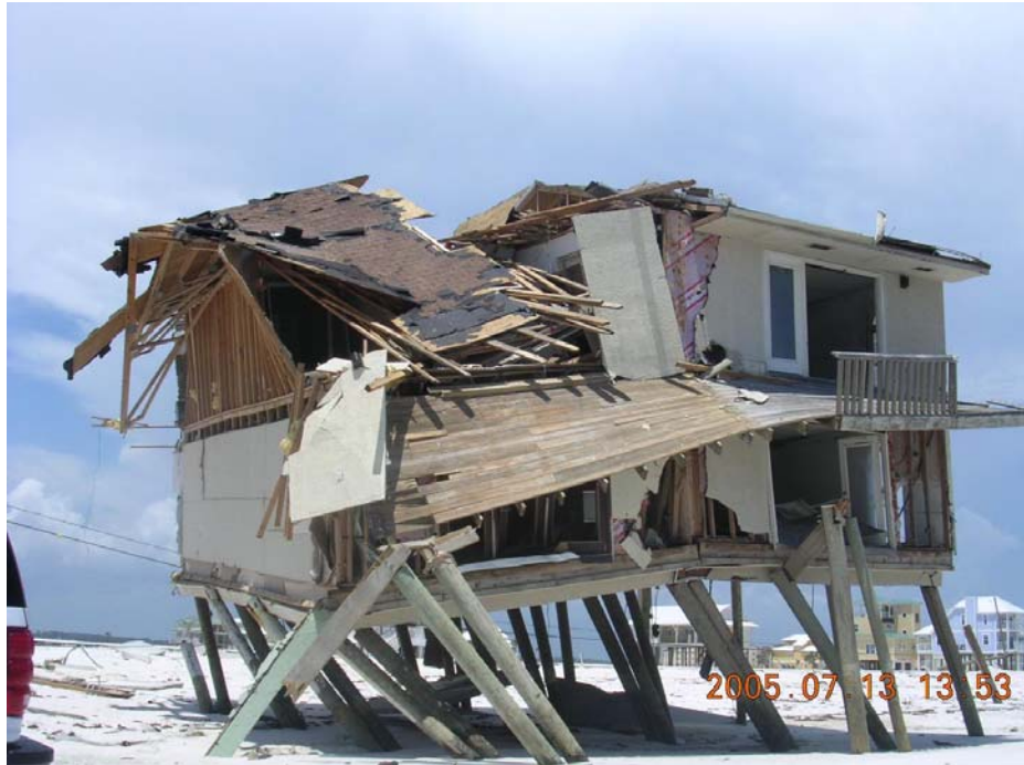
Photo 6. Non-conforming pile supported dwelling destroyed, Navarre Beach (R193).
