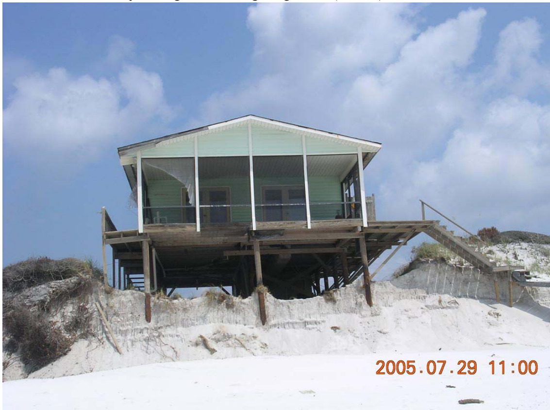
Photo 57. Imminently endangered pile-supported dwelling, Dog Island (R175).
