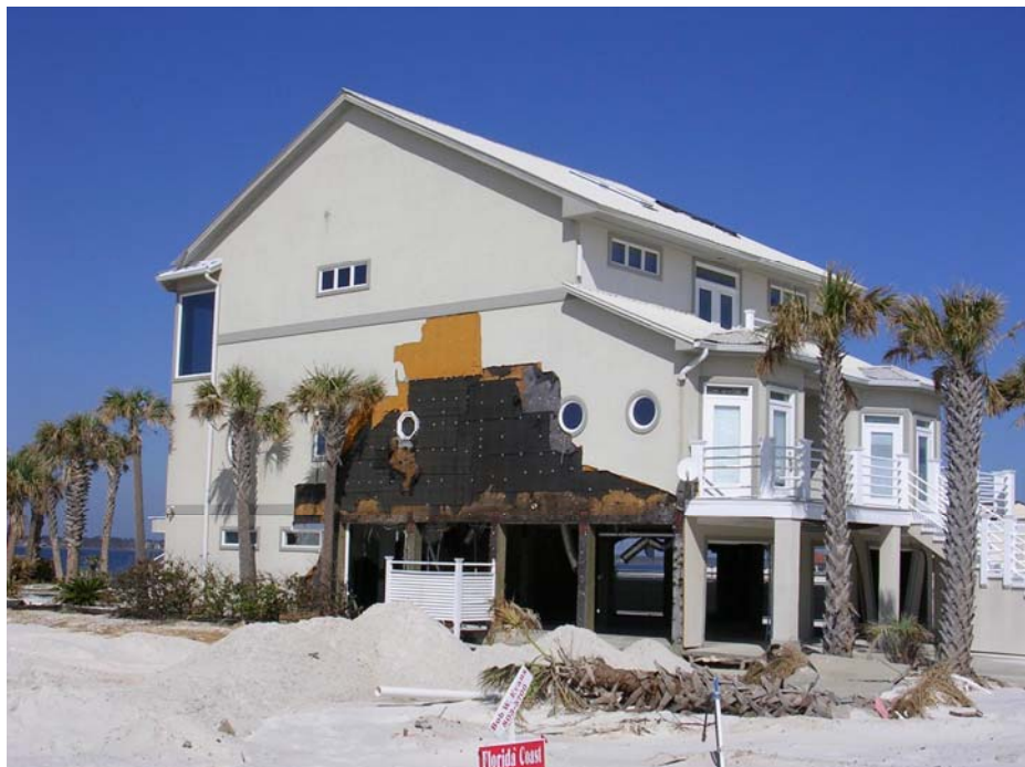
Photo 7. Understructure and siding damage, Navarre Beach (R194).
