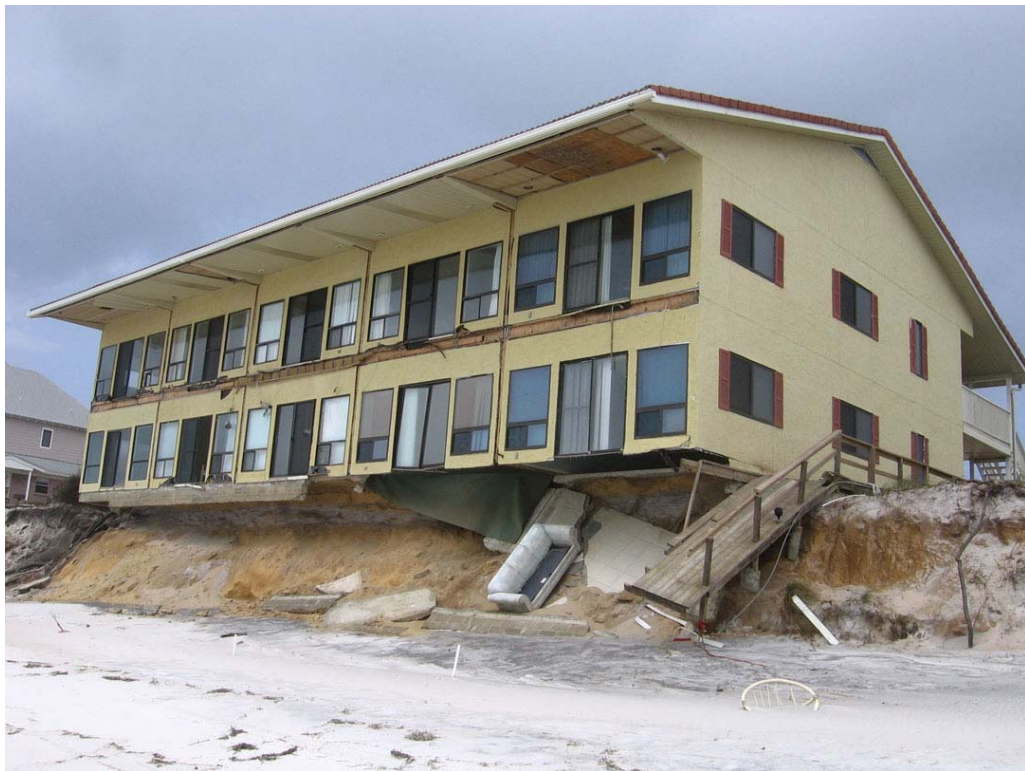
Photo 29. Condominium further undermined by Katrina (R43.2).
