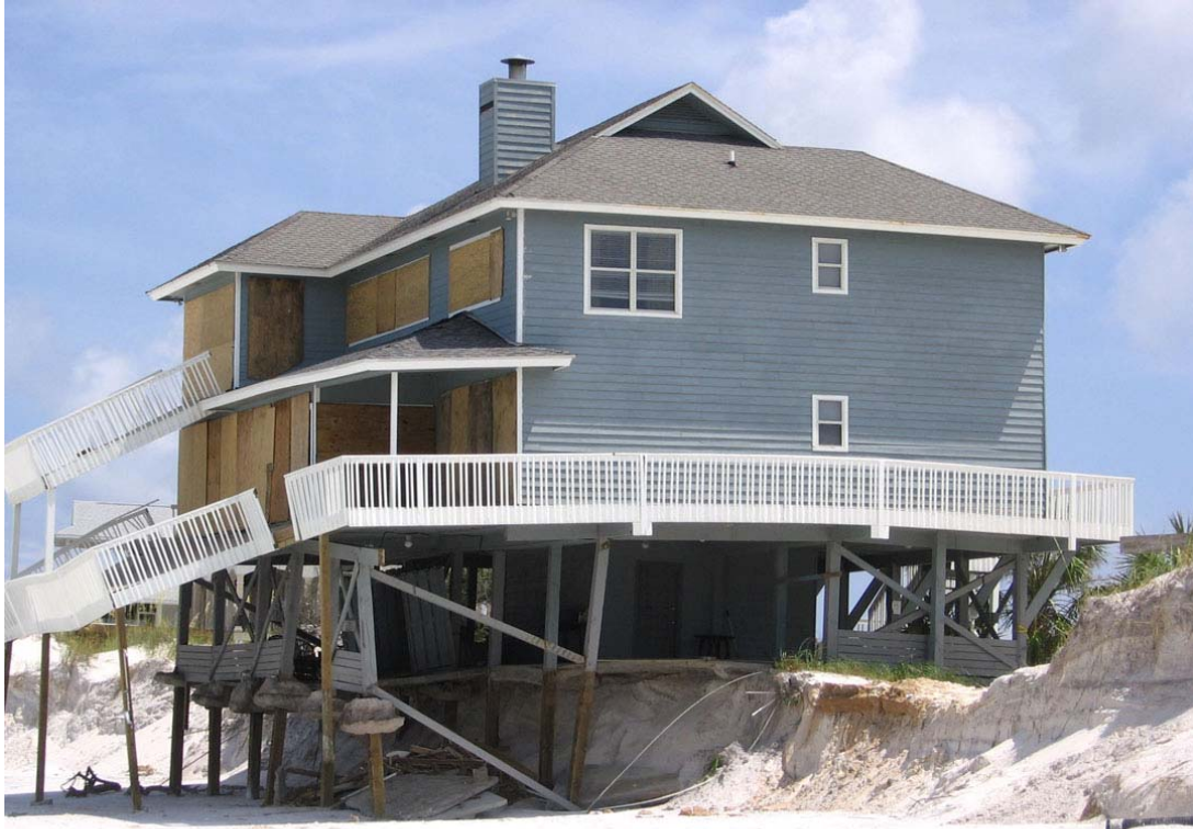
Photo 45. Foundation damage to dwelling, St. Joseph Peninsula (R75.2).
