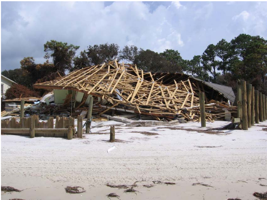
Photo 58. Dwelling destroyed, Southwest Cape (R210.2).
