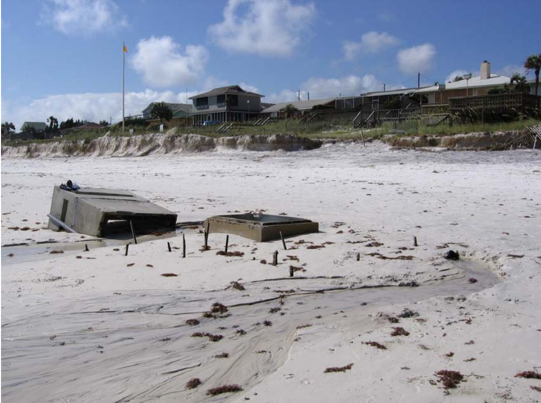
Photo 37. Outfall system damaged (R11).
