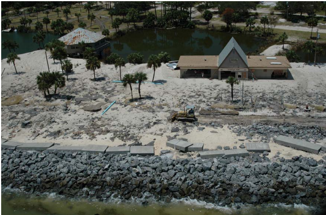
Photo 60. Revetment damaged; road and commercial building destroyed, Southwest Cape (R212.4).
