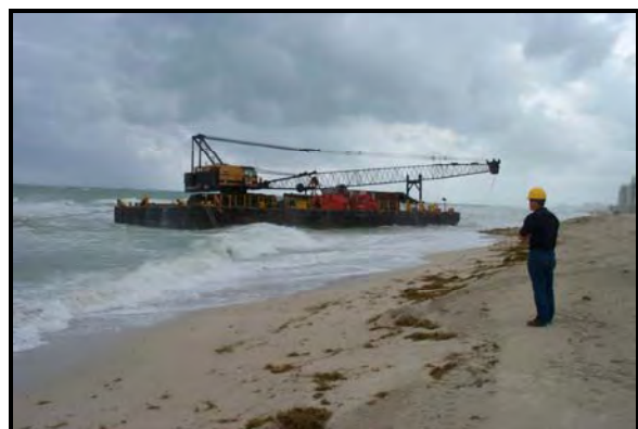
Barge and crane employed to construct mitigation in very nearshore habitat, Miami Dade County. Source: FDEP.
