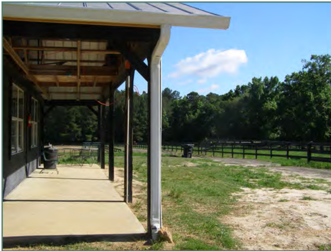
Gutters can help control stormwater runoff.
