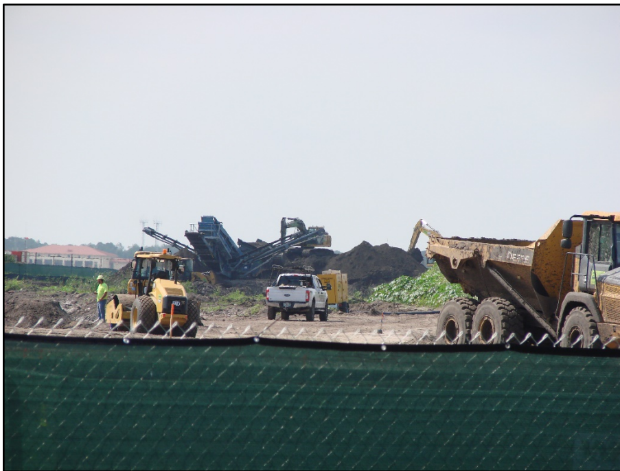
Removing solid waste and screening the waste from the soil to test soils for possible reuse.
