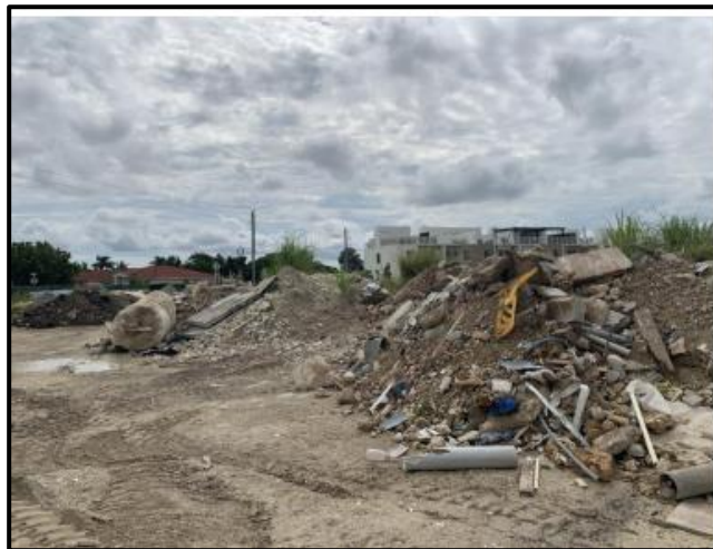
Debris piles during construction
