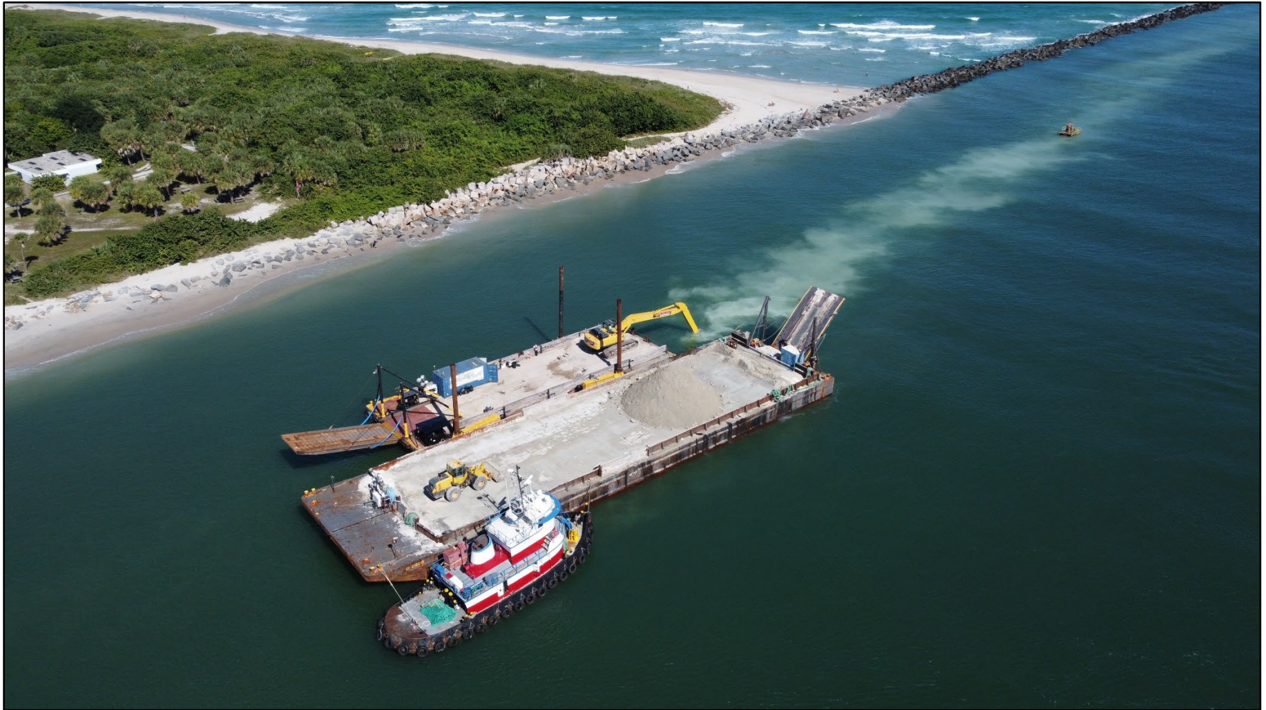
Figure 7: Ahtna Marine and Construction with a barge and backhoe within Ft. Pierce Inlet constructing the inlet sand trap. Photo courtesy of Joshua Revord project manager and P.E with St. Lucie County, November 2021.
