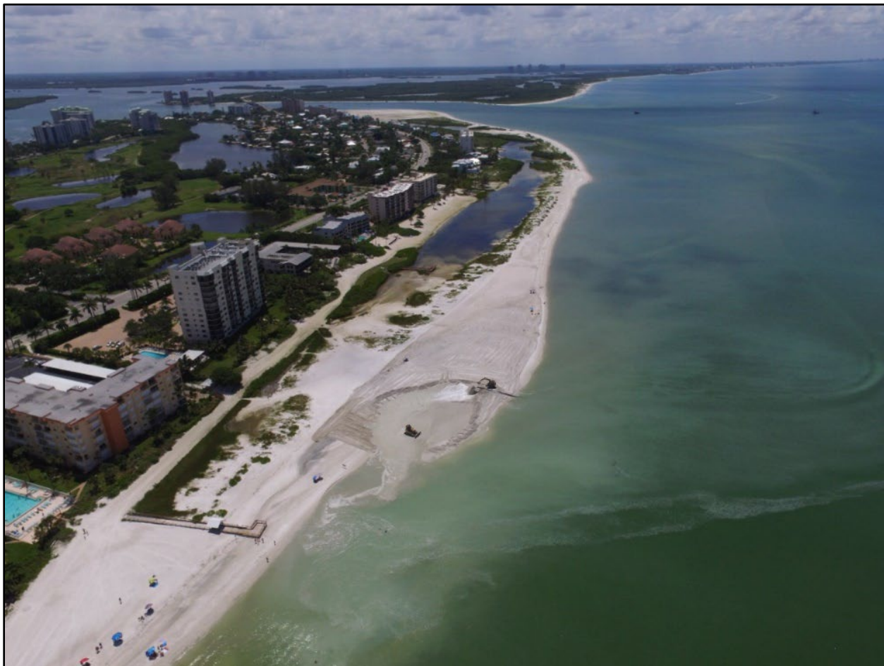
Figure 5. The 2017 fill placement at R-204 during Big Carlos Pass channel maintenance project (photo provided by Humiston & Moore, Inc.).
