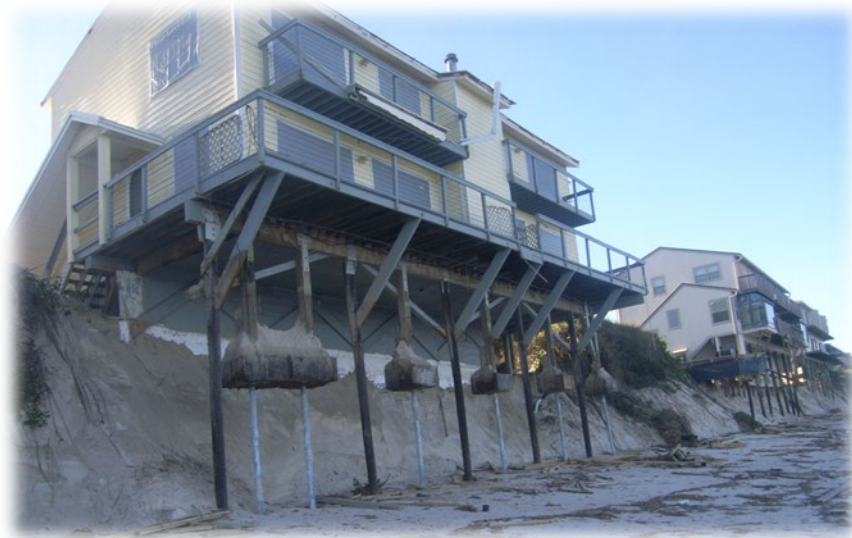
Figure 1 House foundation exposed on a beach eroded by storm waves. Reinforcement of threatened foundations is eligible for local government or CCCL emergency permits under the Department of Environmental Protection’s Emergency Final Order.
