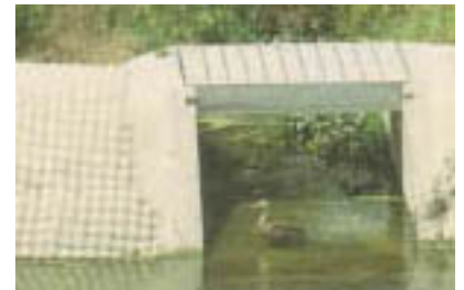
Weirs located along berms covered with grout-filled fabric revetments distribute flow into the cells 2 and 3.
