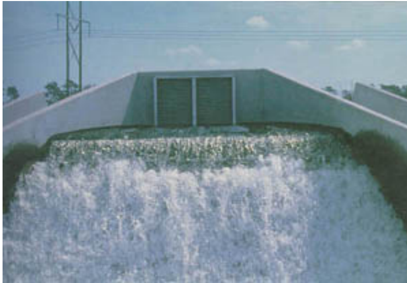
Figure 2. The influent structure aerates the water as it enters the wetland.
