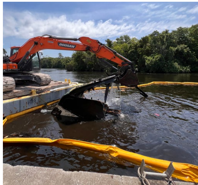
Turbidity curtains deployed for sedimentation containment during marine debris removal in Levy County, Florida (Source: Avery Bristol, FWC)
