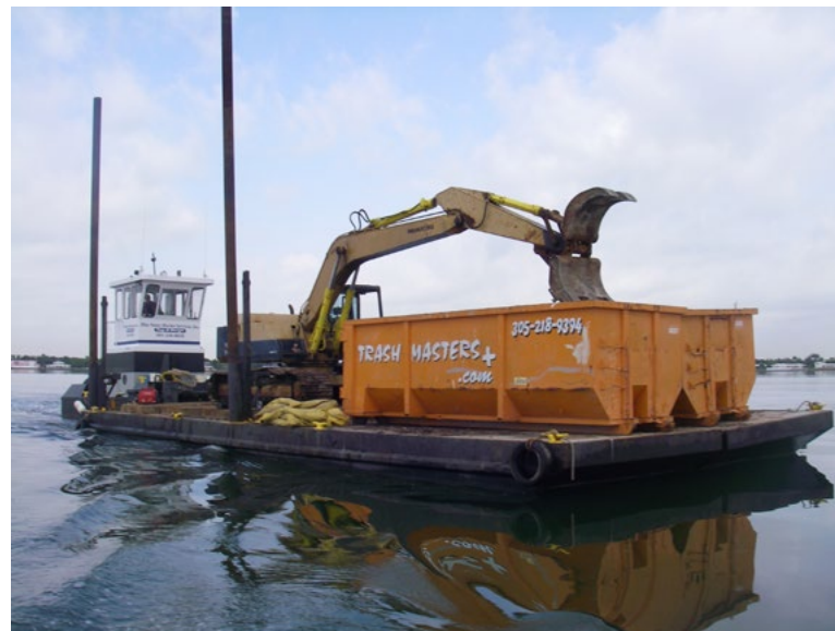
Barge-mounted excavator used to deposit debris directly into waste receptacle. (Source: FWC)
