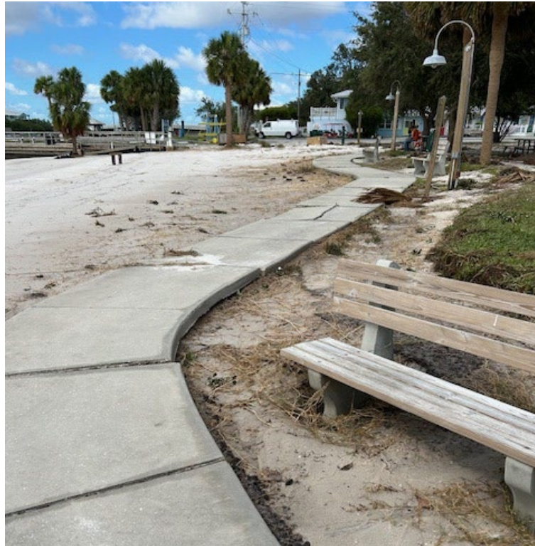
Figure 57. Scoured upland and damaged sidewalk at public beach, Cedar Key.
