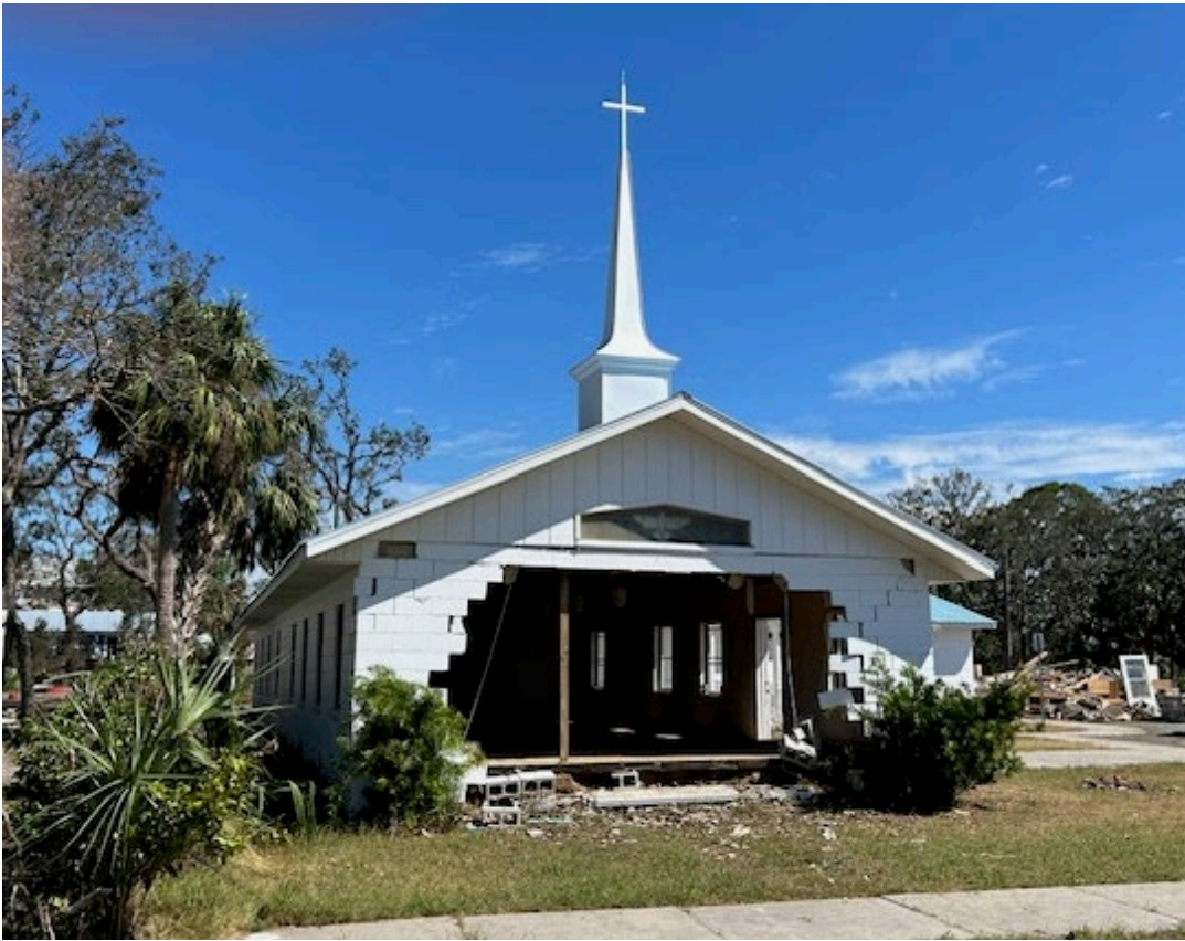
Figure 44. Grade level church was destroyed in Horseshoe Beach.
