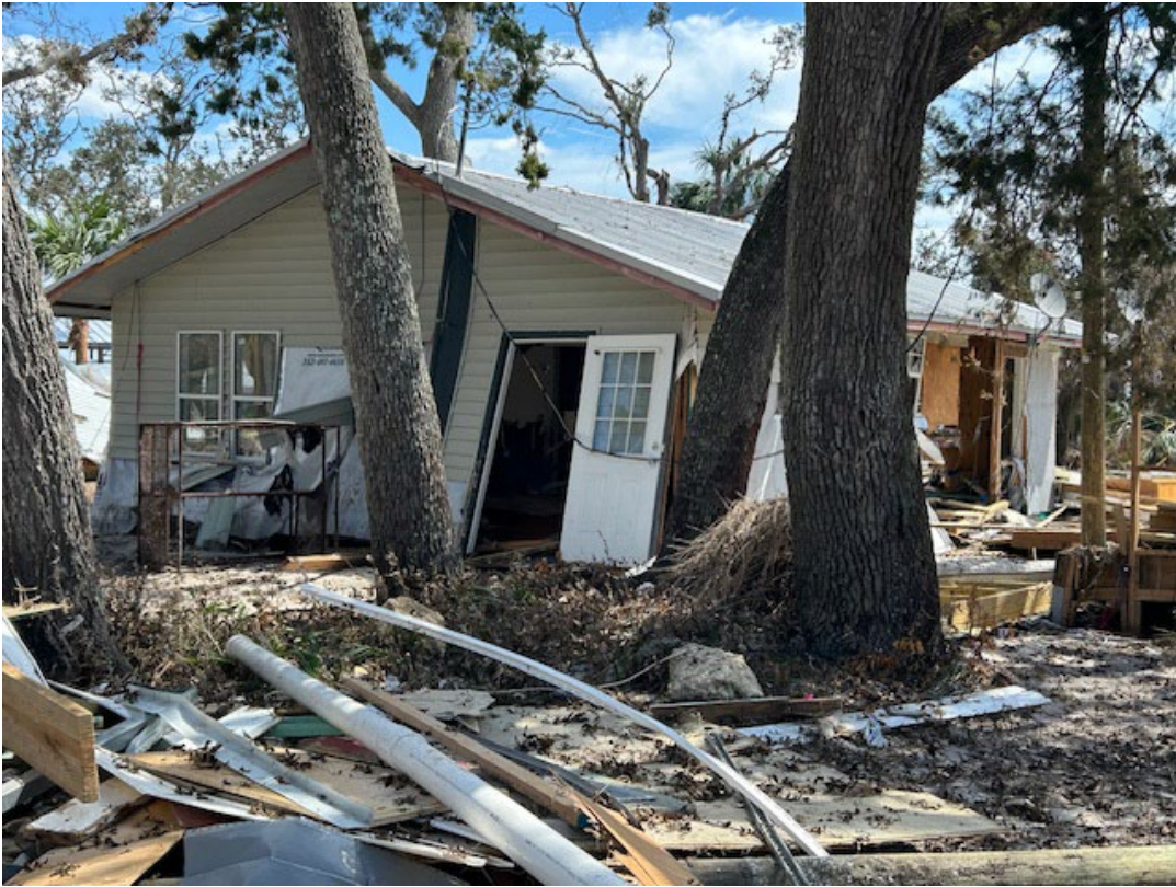
Figure 43. Grade level dwelling was destroyed in Horseshoe Beach.
