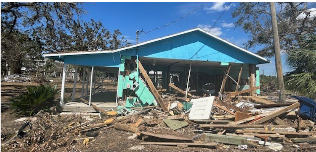
Figure 41. Grade level dwelling destroyed in Horseshoe Beach.
