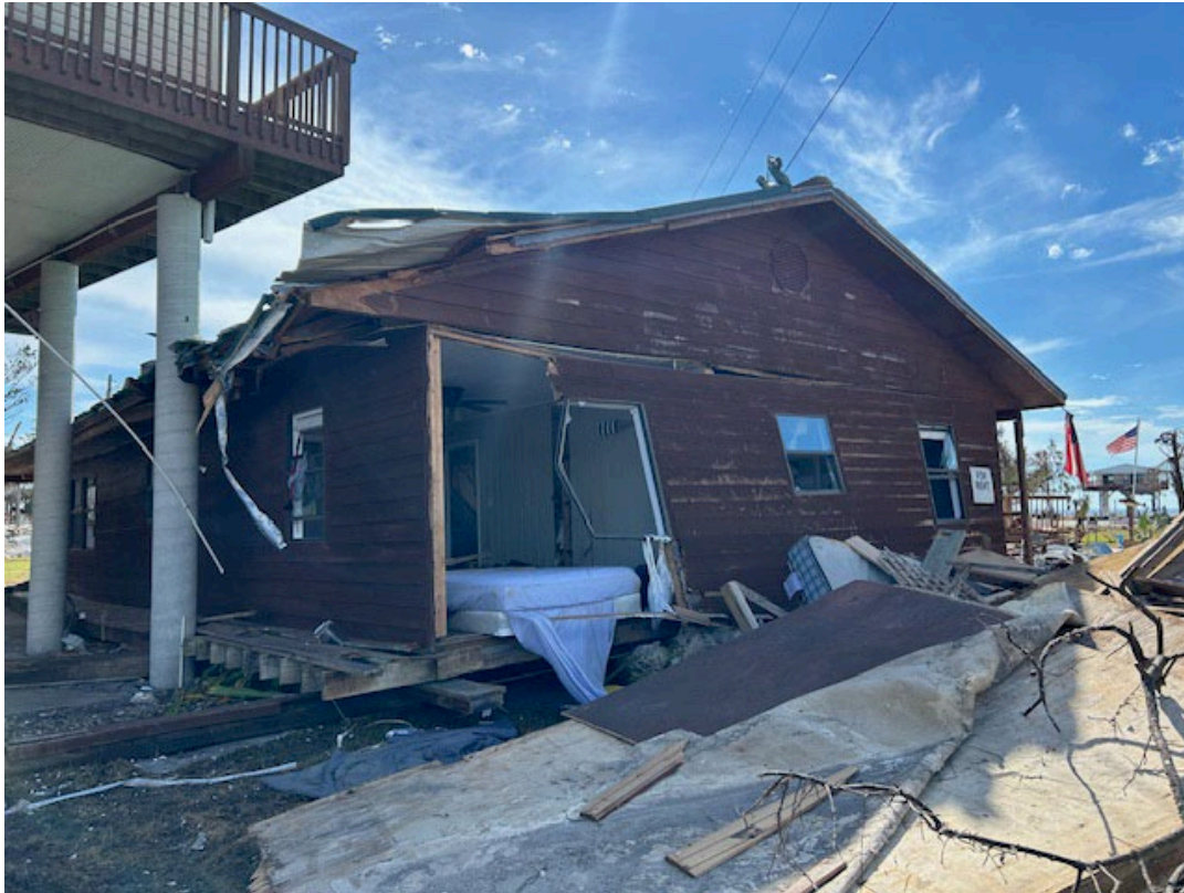
Figure 20. Keaton Beach dwelling carried across a canal and deposited on a neighbor's driveway.
