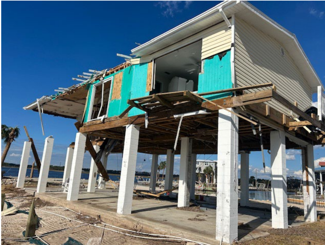
Figure 27. Three fourths of the houses on Dark Island were destroyed or sustained major structural damage.
