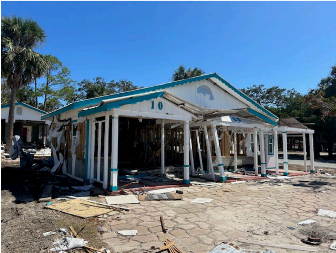
Figure 59. One of 5 destroyed motel buildings on G Street, Cedar Key.
