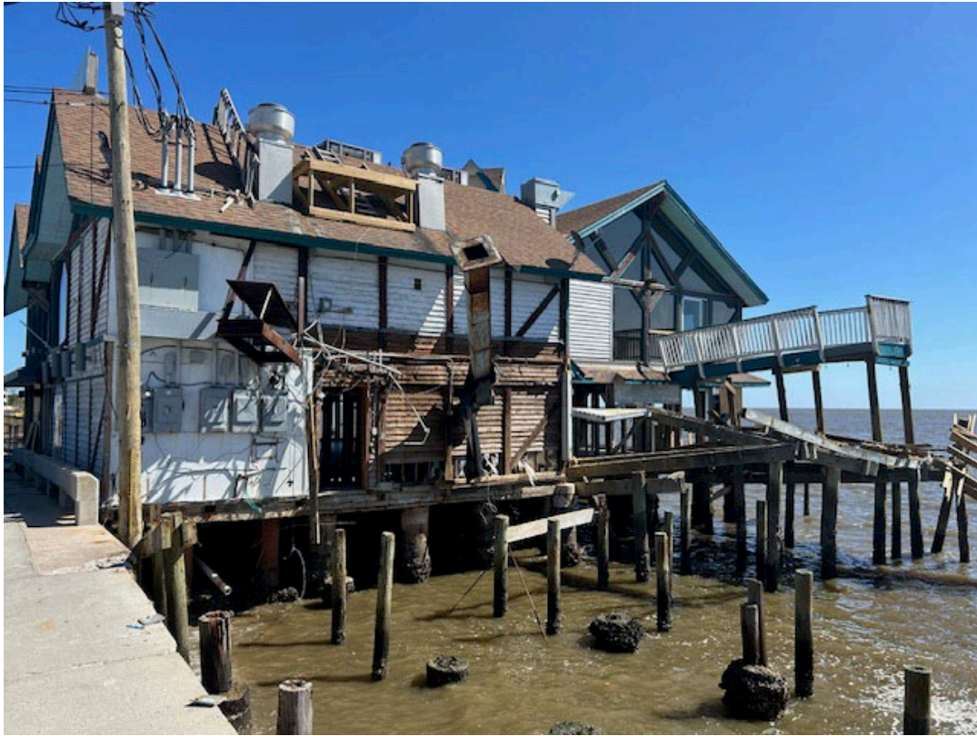
Figure 63. Commercial building damaged on Water Street, Cedar Key.
