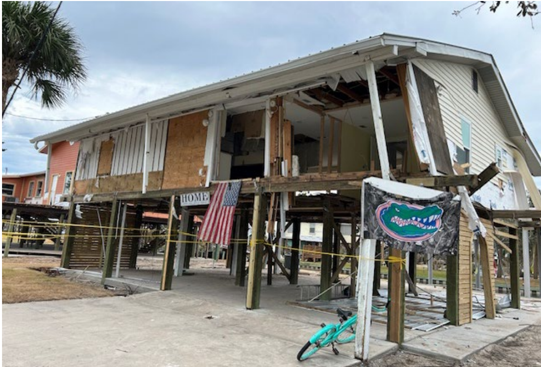
Figure 46. Pile supported dwelling damaged due to insufficient elevation.
