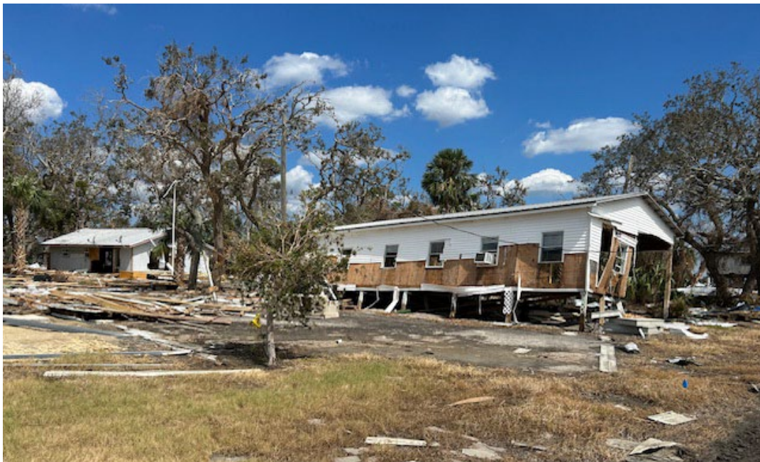
Figure 47. Buildings destroyed with insufficient elevations.
