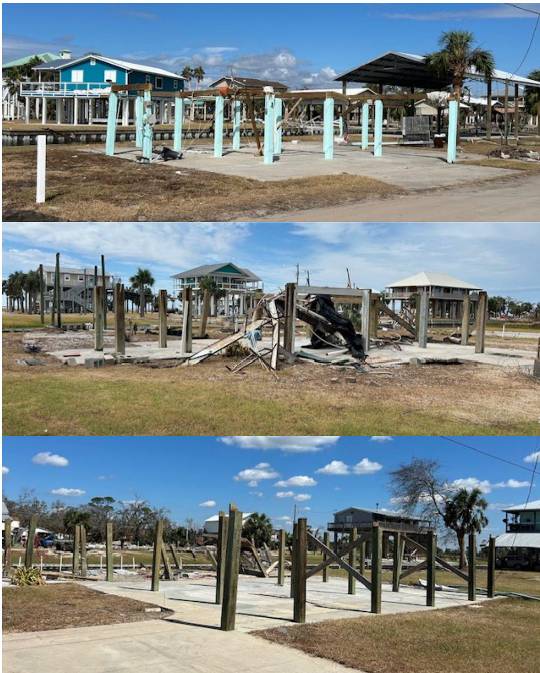
Figure 45. Three pile supported dwellings in Horseshoe Beach destroyed due to insufficient elevation for Helene's storm surge and waves.
