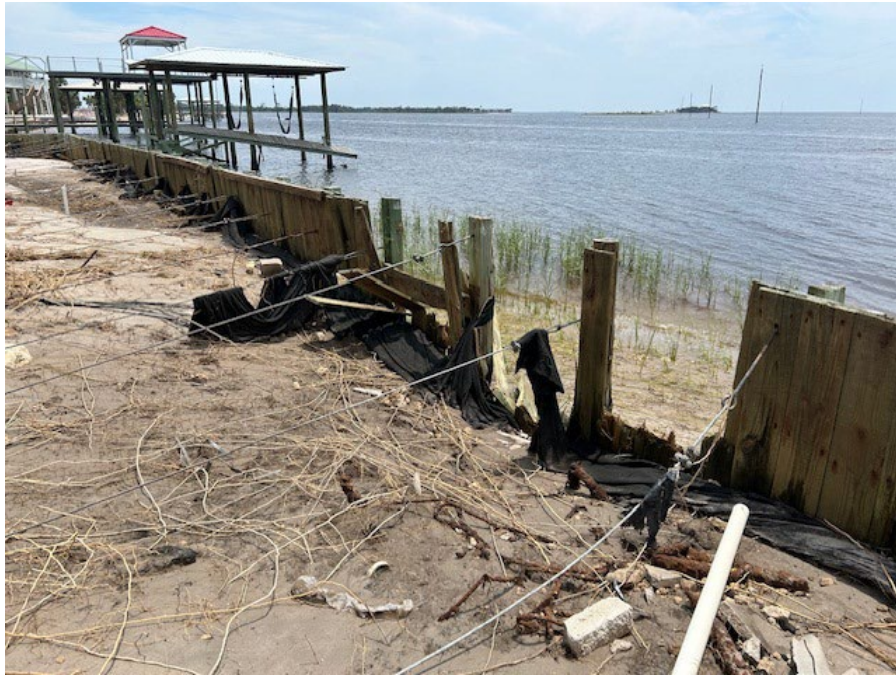
Figure 36. Damage to a timber wall at Horseshoe Beach by Debby.
