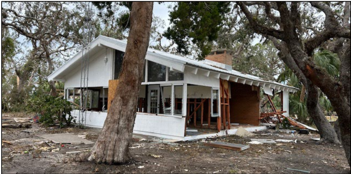
Figure 39. Grade level dwelling destroyed in Horseshoe Beach.
