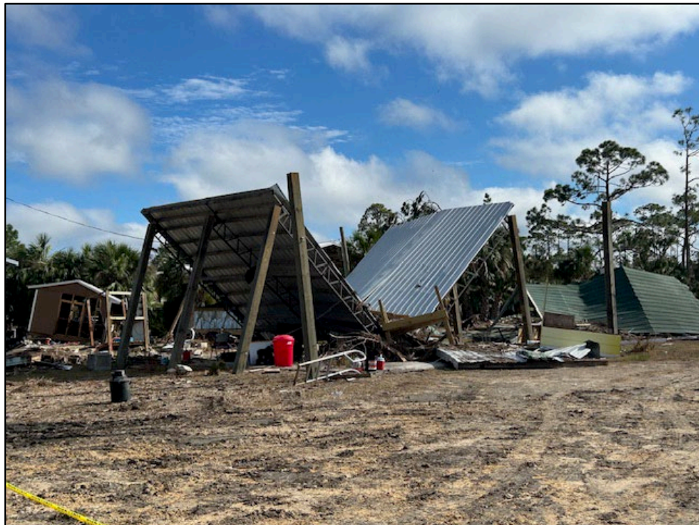
Figure 23. Recreation vehicle shelter destroyed on Cedar Island.
