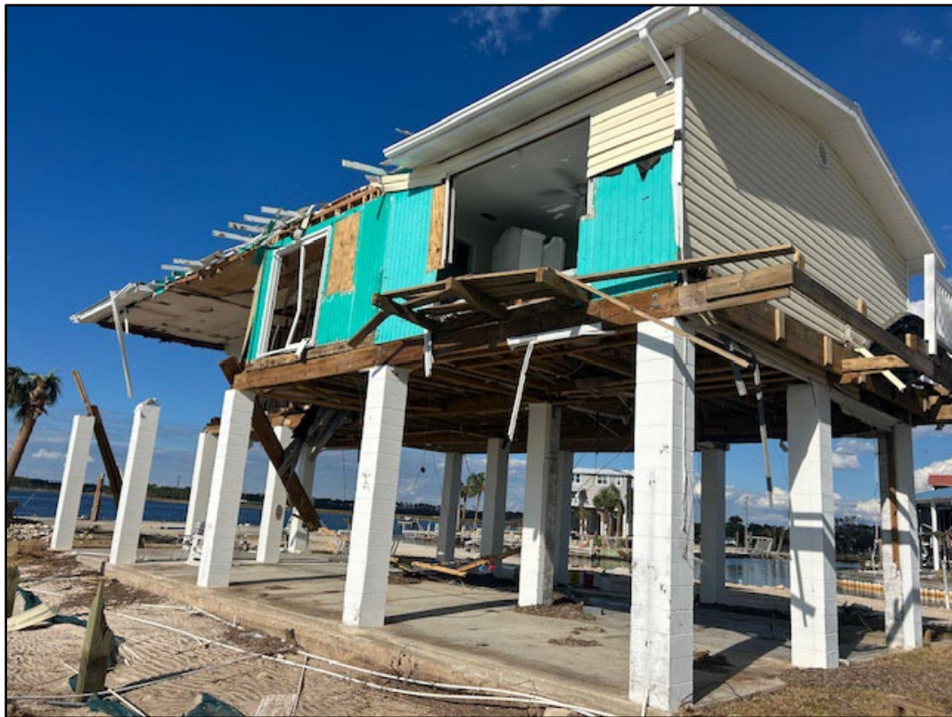
Figure 26. Three fourths of the houses on Dark Island were destroyed or sustained major structural damage.
