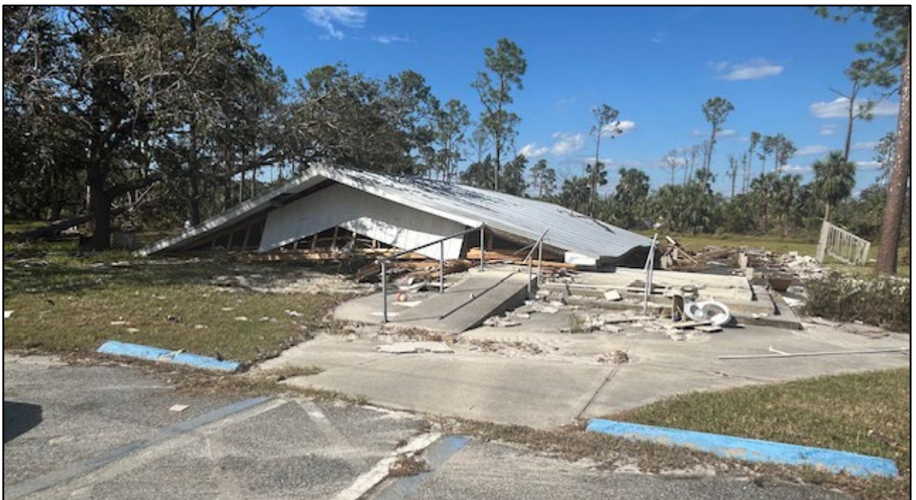
Figure 41. Grade level of a church building destroyed in Horseshoe Beach.
