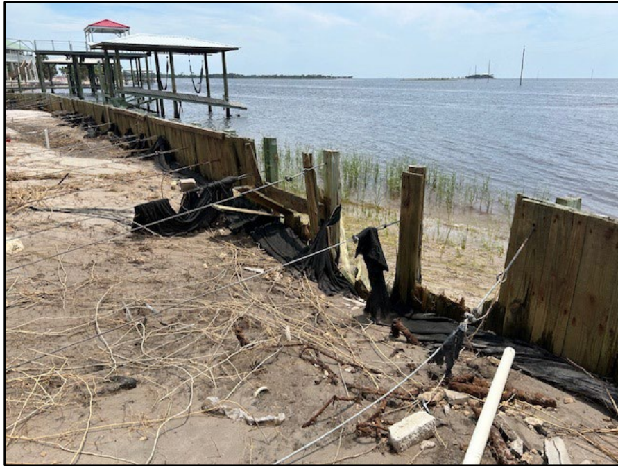
Figure 35. Damage to a timber wall at Horseshoe Beach by Debby.
