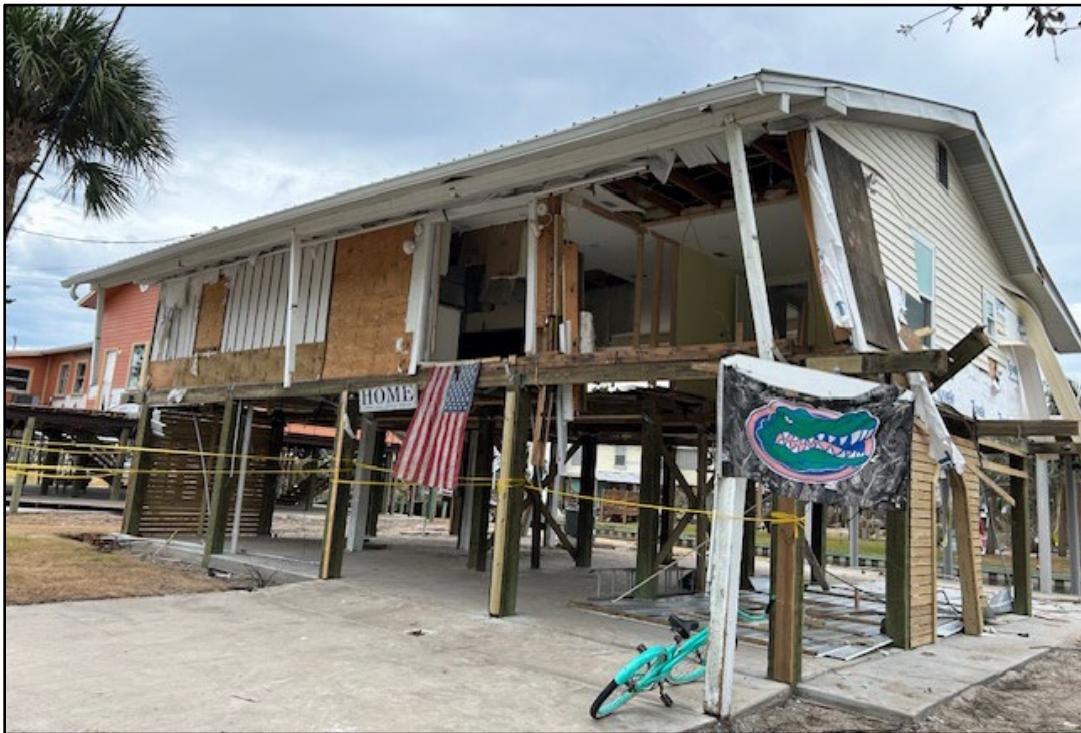
Figure 45. Pile supported dwelling damaged due to insufficient elevation.
