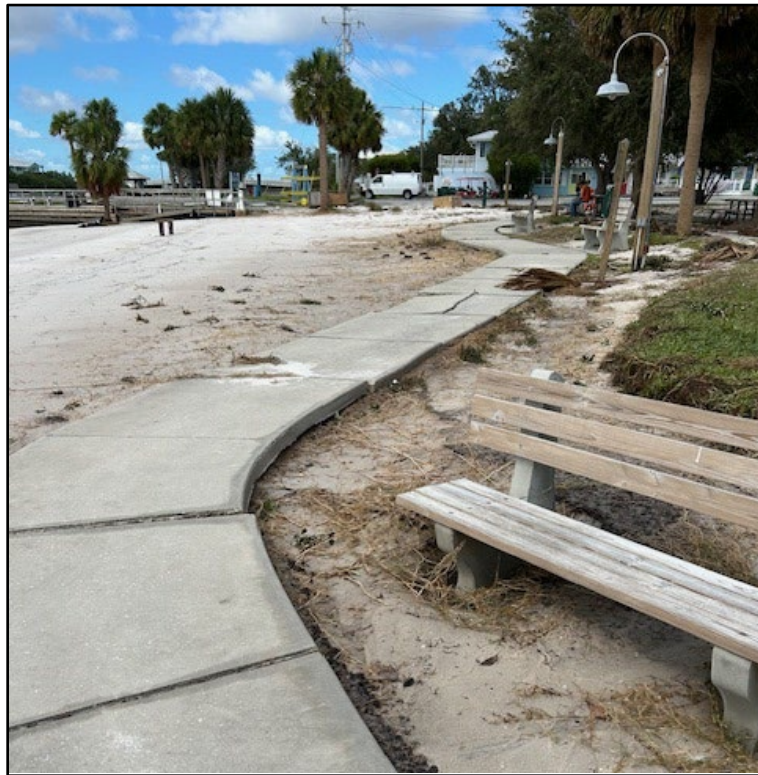
Figure 56. Scoured upland and damaged sidewalk at public beach, Cedar Key.
