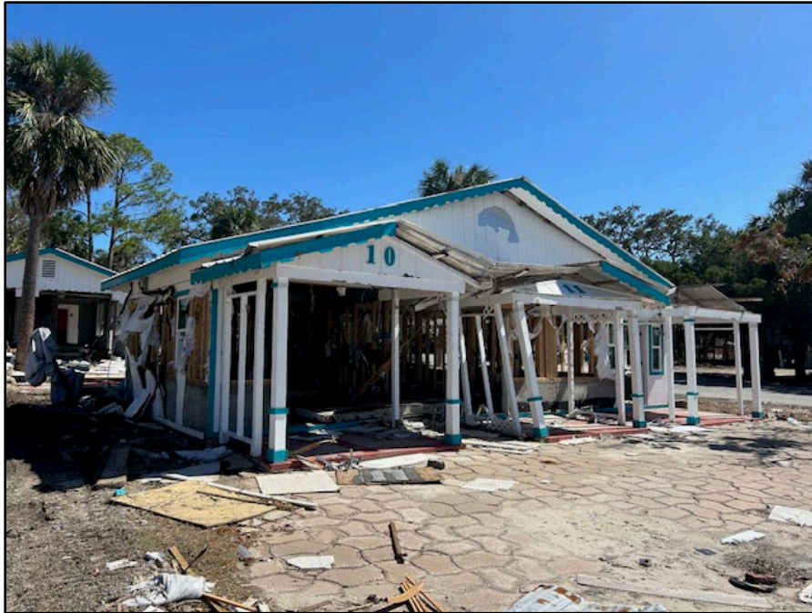
Figure 58. One of five destroyed motel buildings on G Street, Cedar Key.
