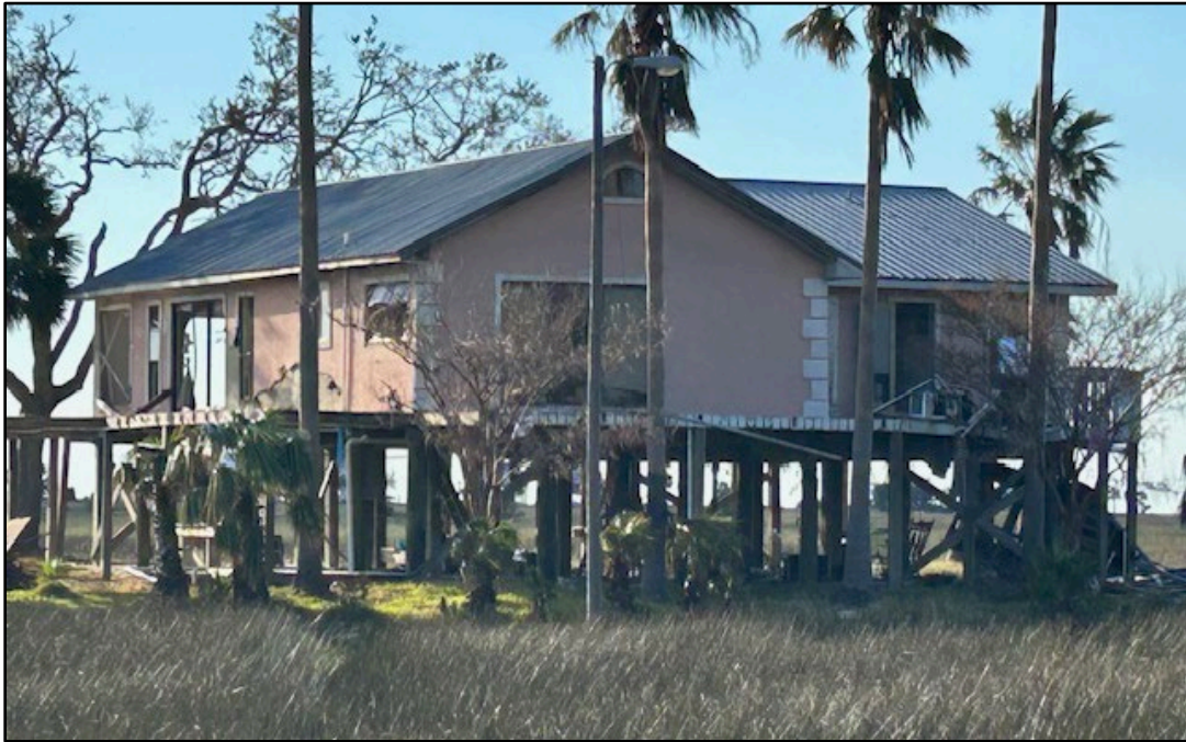
Figure 27. Damaged house on Bird Island.
