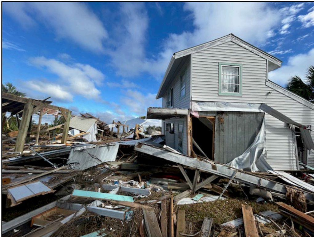
Figure 21. Catastrophic damage on Cedar Island.
