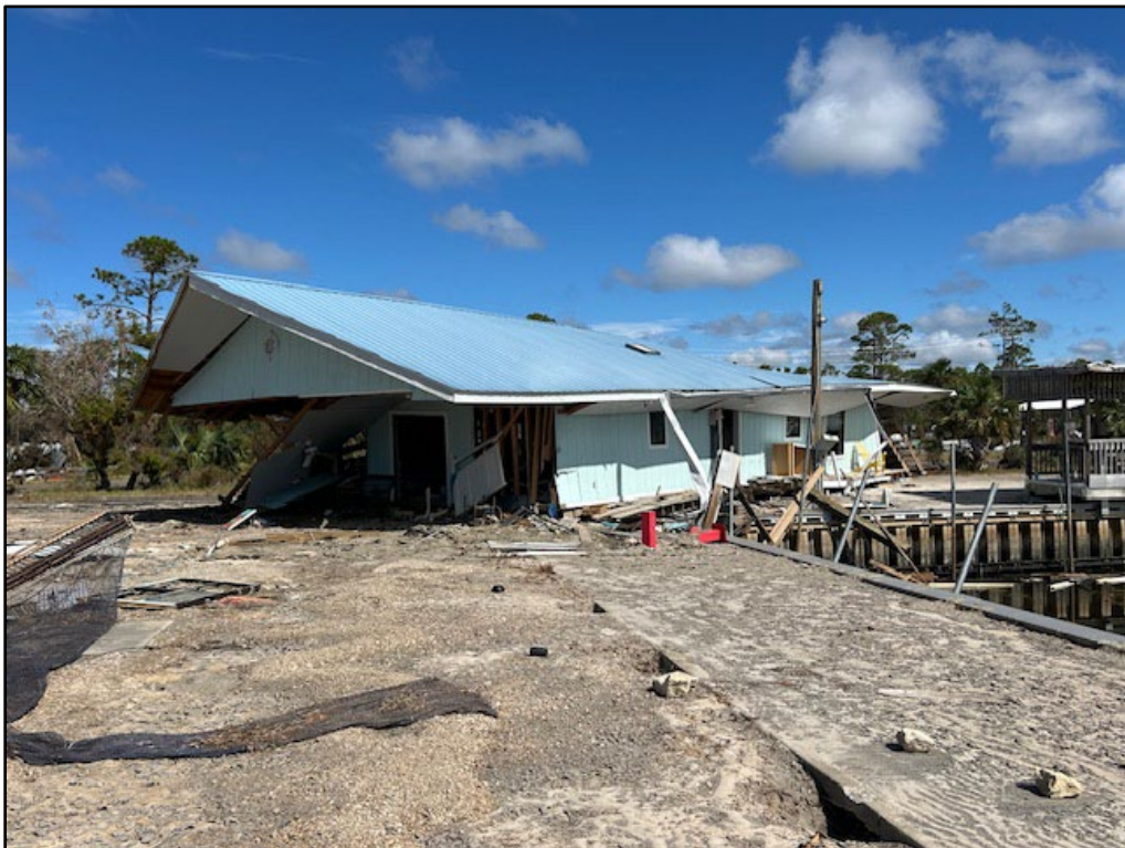
Figure 18. Keaton Beach dwelling on a road blocking access.
