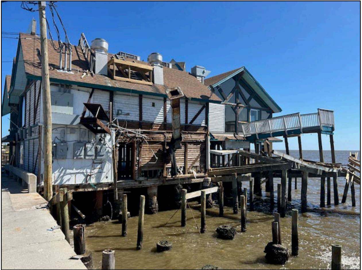
Figure 62. Commercial building damaged on Water Street, Cedar Key.
