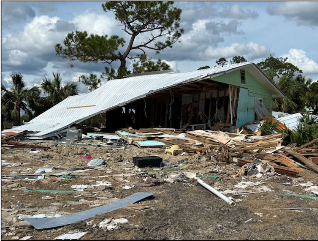
Figure 14. Dekle Beach dwelling destroyed.
