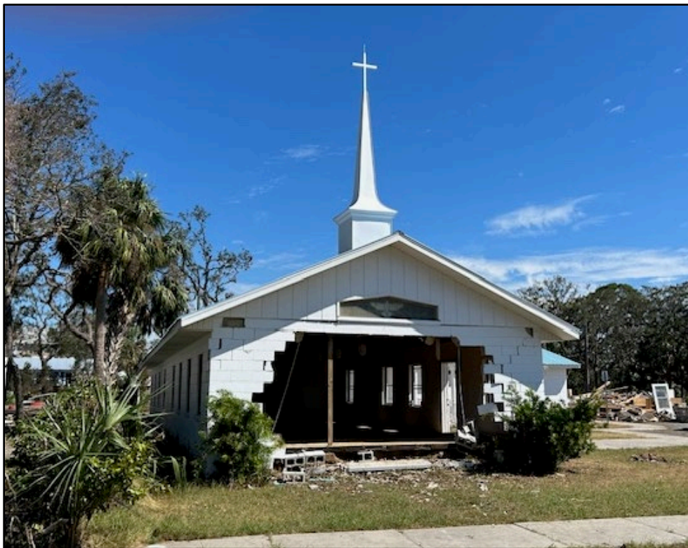
Figure 43. Grade level of a church destroyed in Horseshoe Beach.
