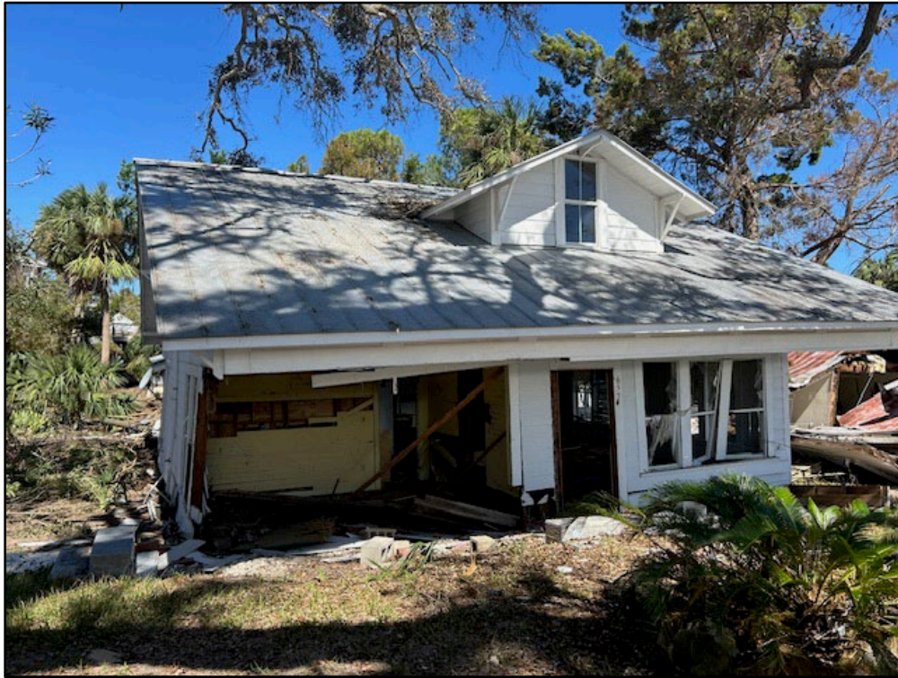
Figure 60. Single-family dwelling destroyed on 1st Street, Cedar Key.
