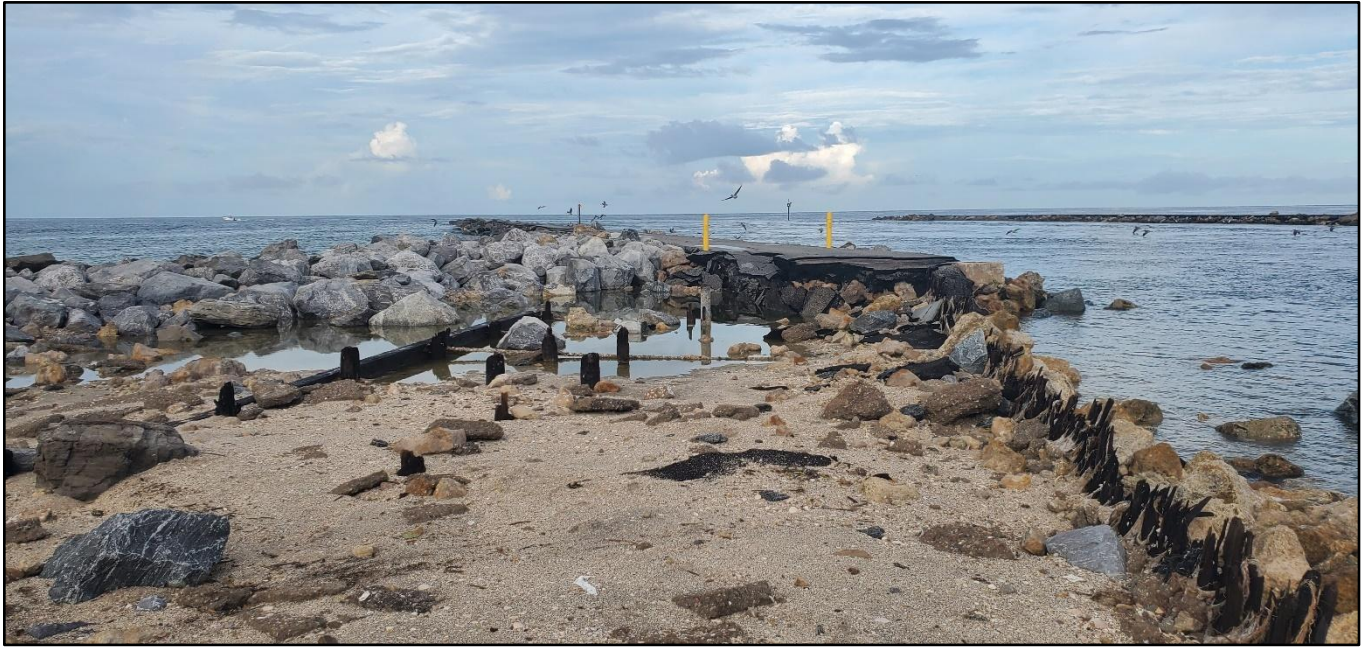
Figure 99. Major damage to Venice Inlet south jetty and bulkhead by Helene, R-115.
