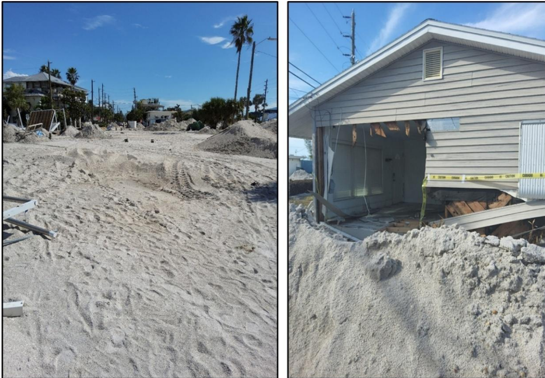
Figure 18. Overwash due to Helene’s storm surge on Treasure Island near R-137 (left) and R-139 (right).
