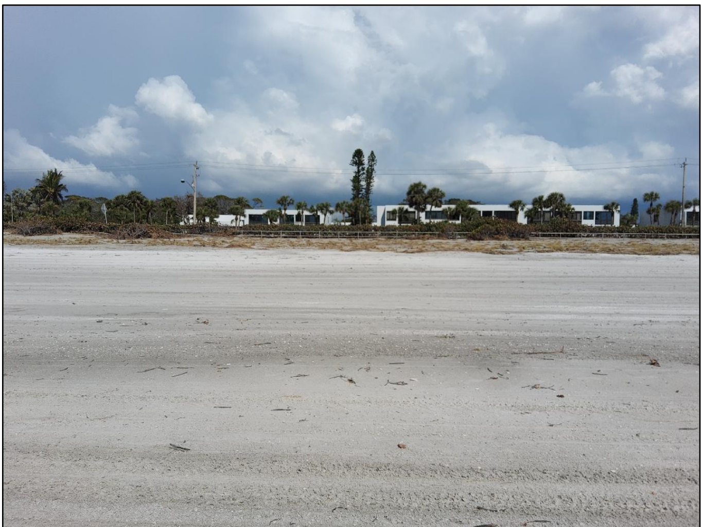
Figure 53. Major beach and dune erosion (condition IV) following Helene and Milton on Longboat Key (R-2 to R-3).
