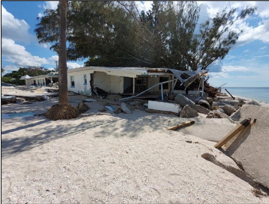
Figure 91. Multi-family dwelling destroyed on Casey Key near R-90.
