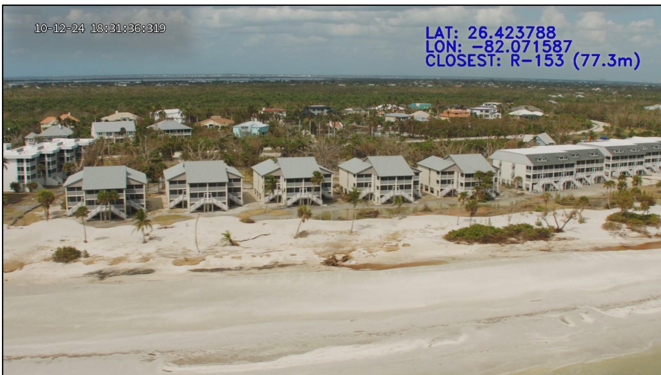
Figure 133. Major beach and dune erosion (condition IV) due to Helene and Milton on Sanibel Island near R-153.
