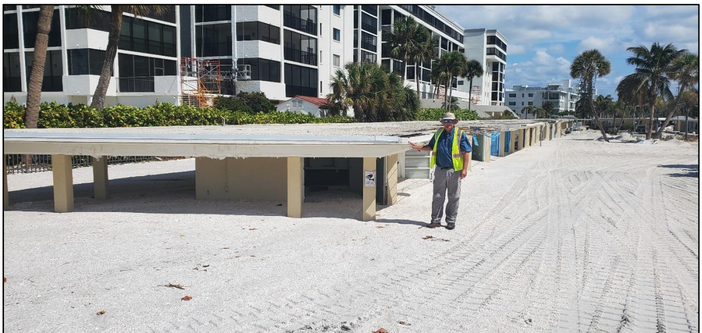
Figure 57. Major damage to a Lido Key hotel from Helene’s storm surge and overwash deposit of approximately three to four feet of beach sand near R-40.
