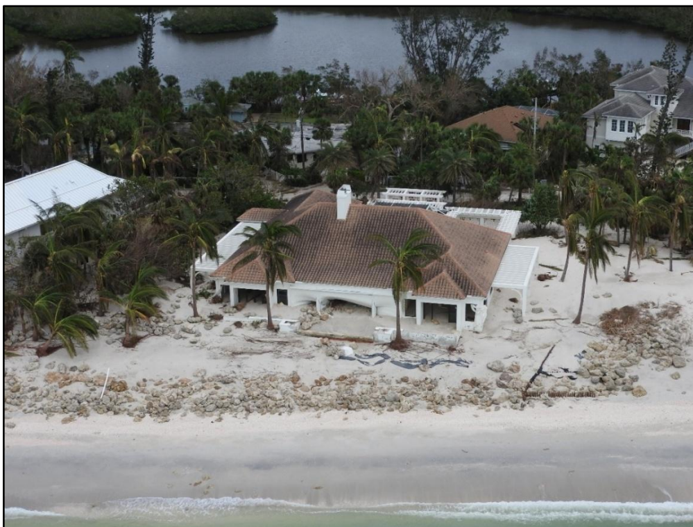
Figure 94. Single-family dwelling with major first floor damage by Milton on Casey Key, near R-95.
