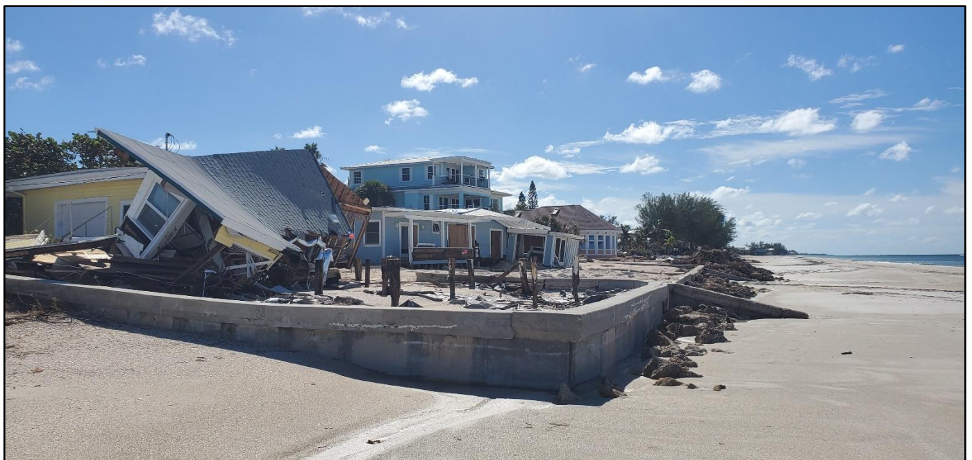
Figure 40. A single-family dwelling destroyed by Helene's storm surge on Anna Maria Island next to another home with major first floor damage near Avenue F near R-23.
