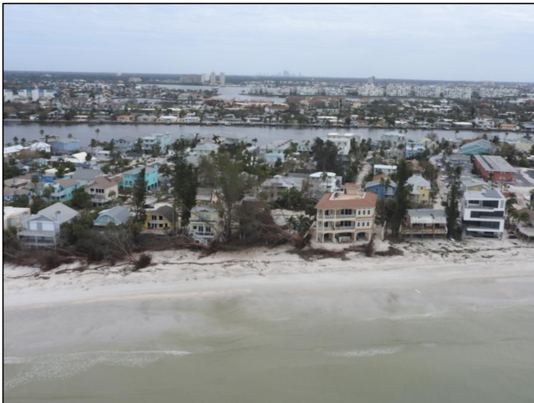
Figure 19. Major beach and dune erosion (condition IV) following Helene and Milton on Treasure Island (R-141).
