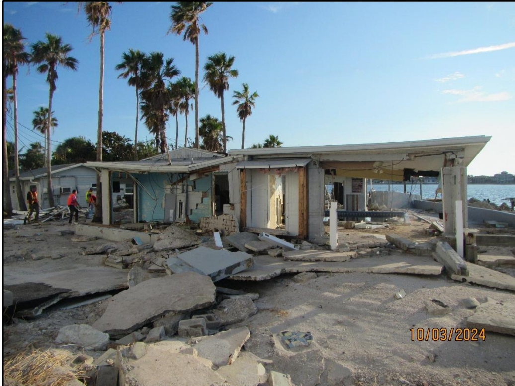
Figure 22. Damage of dwellings in St. Pete Beach due to Hurricane Helene near R-166.
