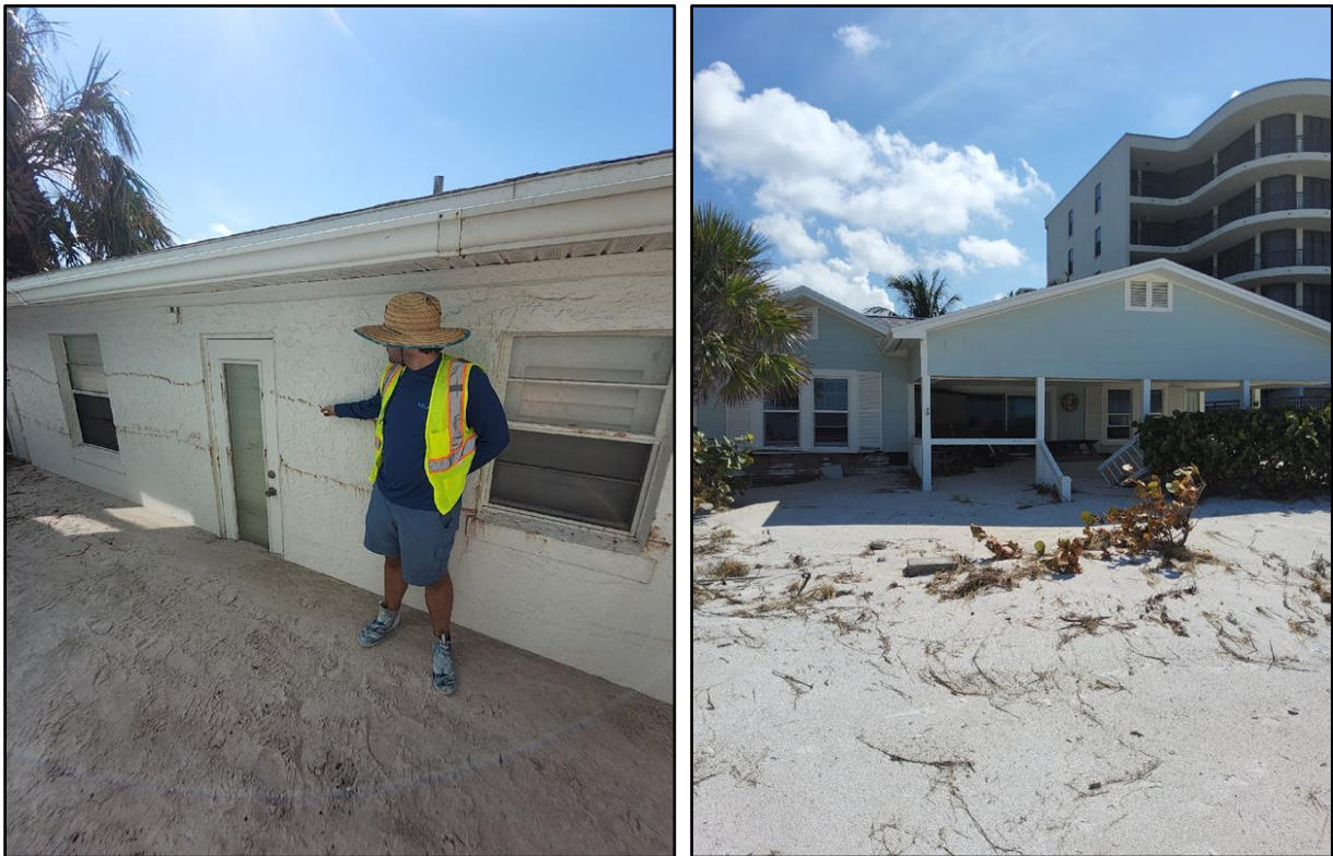
Figure 16. Indian Shores beach dwellings impacted by overwash sand from Helene’s storm surge at R-83 (left) and R-91 (right).
