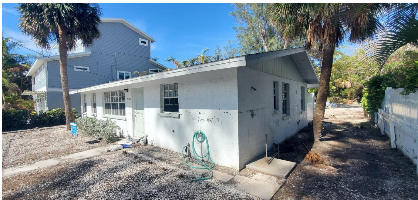
Figure 46. A single-family dwelling flooded by Helene’s storm surge on Anna Maria Island. Note the high water mark above the outdoor shower handle and the front window base.
