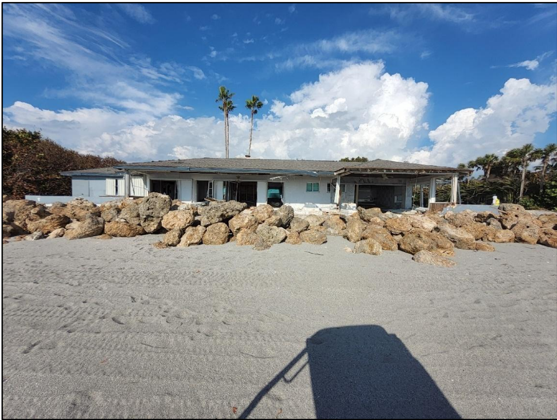
Figure 85. Major damage to rock revetment (level III) and to single-family dwelling on Siesta Key near R-67.
