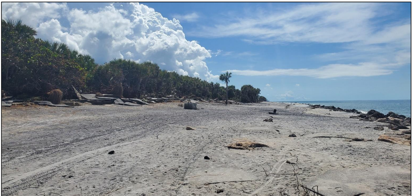
Figure 75. Major beach and dune erosion (condition IV) and major road damage at Caspesan Beach near R-136.
