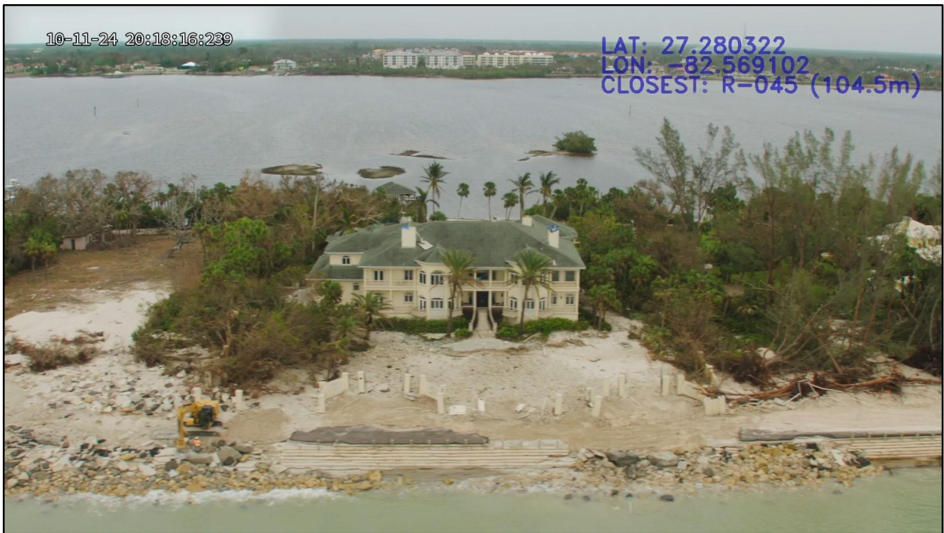
Figure 89. Major road and revetment damages from Helene’s storm surge on Casey Key near R-85.
