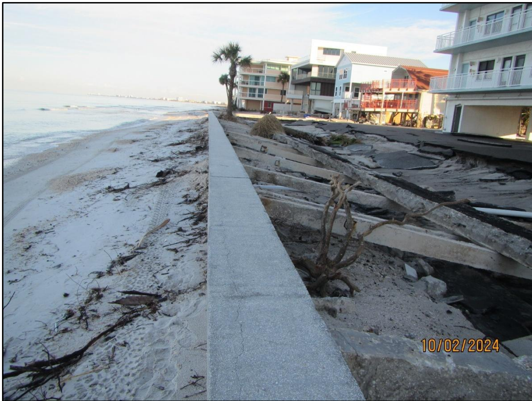
Figure 23. Seawall damage in Treasure Island/ Sunset Beach due to Hurricane Helene near R-139.
