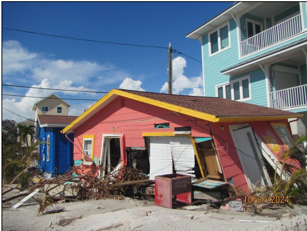
Figure 21. Damage to single family dwelling on Treasure Island due to Hurricane Helene near R-141.
