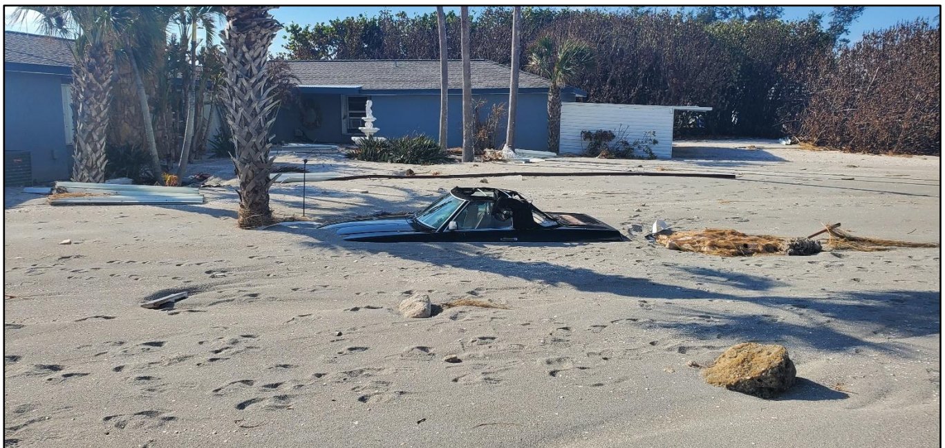
Figure 63. Storm surge damages to home and yard from Helene and Milton on Siesta Key near R-67. Note: Mercedes convertible buried in 3 to 4 feet of overwash sand.
