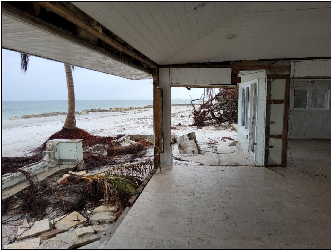
Figure 51. A single-family dwelling destroyed by Helene and major erosion (condition IV) on northern Longboat Key, near R-50.
