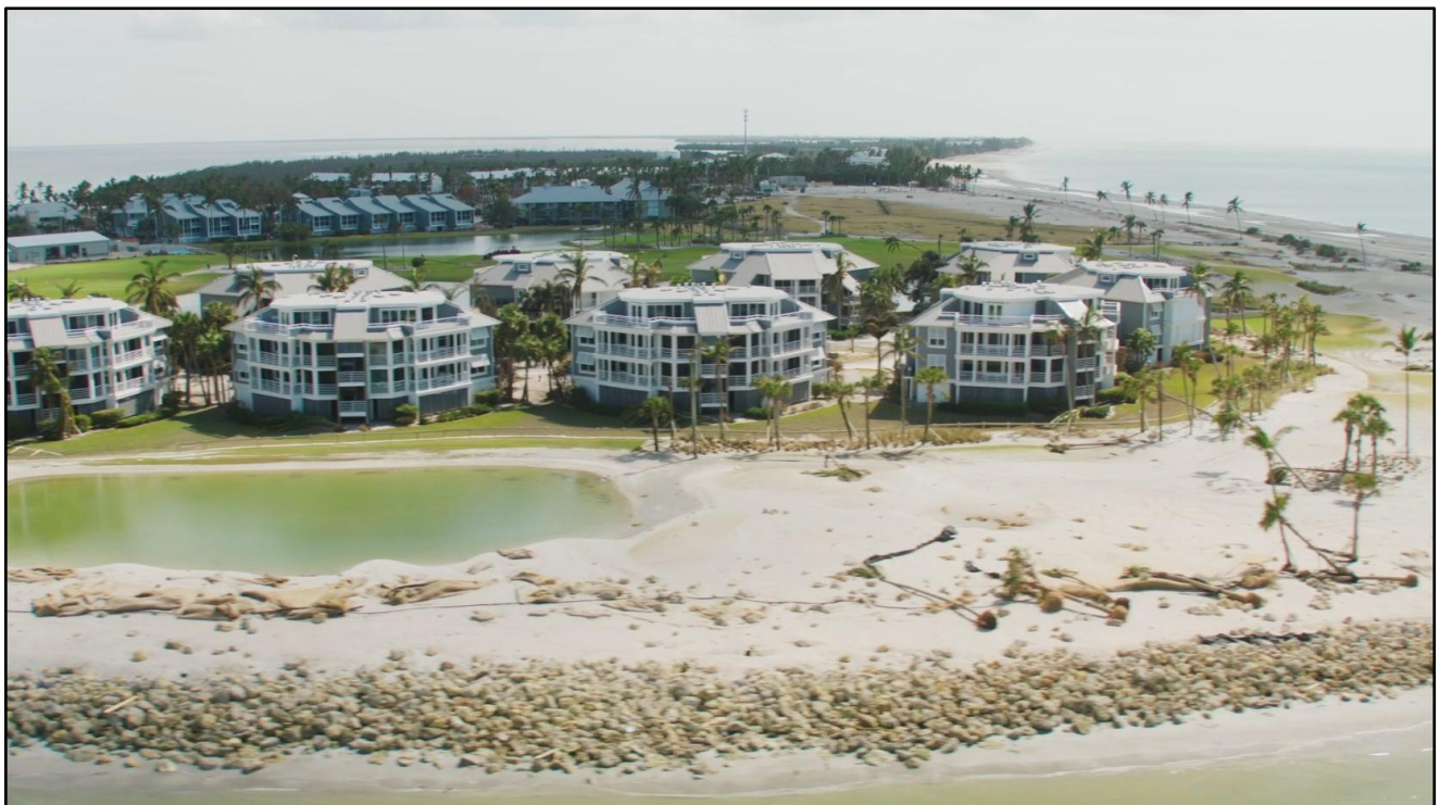
Figure 141. Rock revetment damage at South Seas Plantation at Redfish Pass on Captiva Island near R-84.
