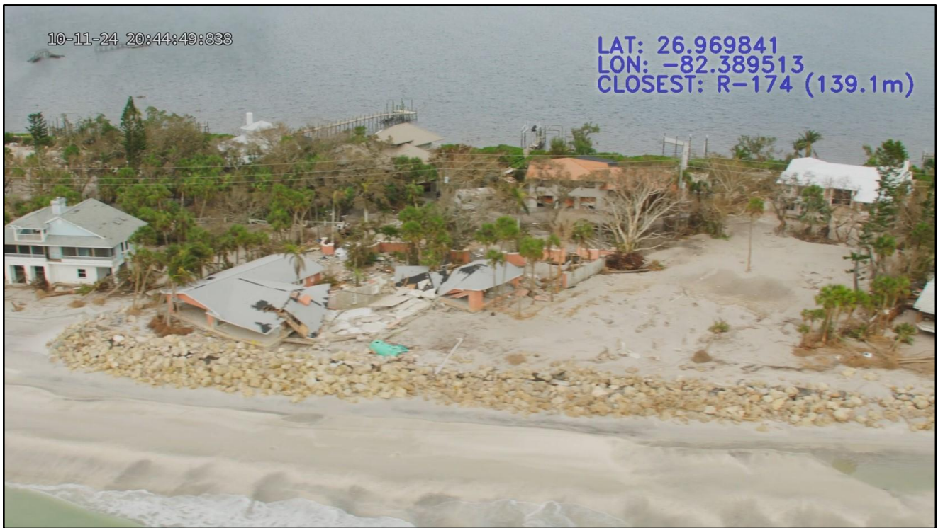
Figure 105. Single-family dwelling destroyed and major revetment damage by Milton on Manasota Key, R-173.
