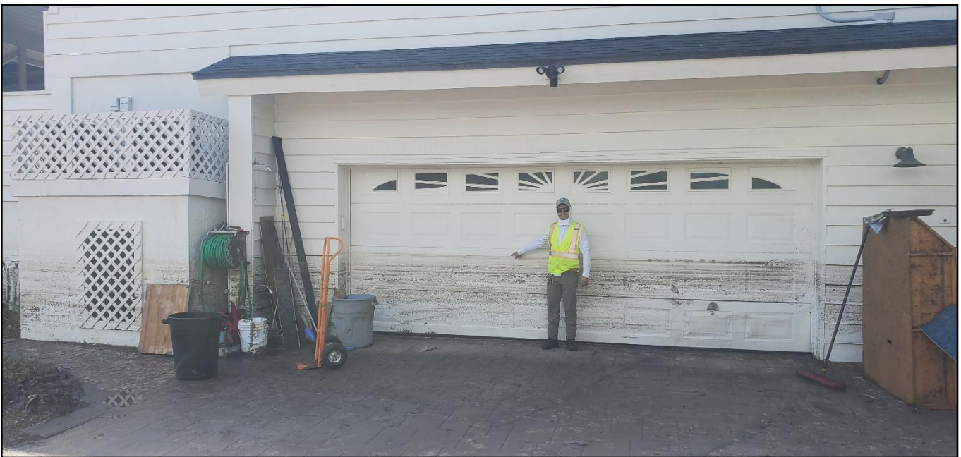
Figure 77. High water mark on garage door on Manasota Key (R-173).
