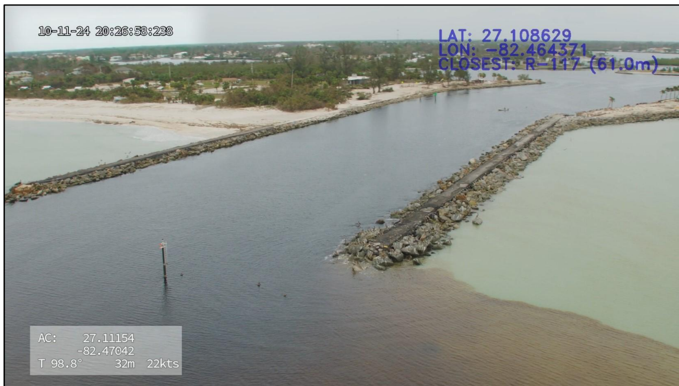
Figure 96. Major damage to the jetties of Venice Inlet by Helene and Milton.
