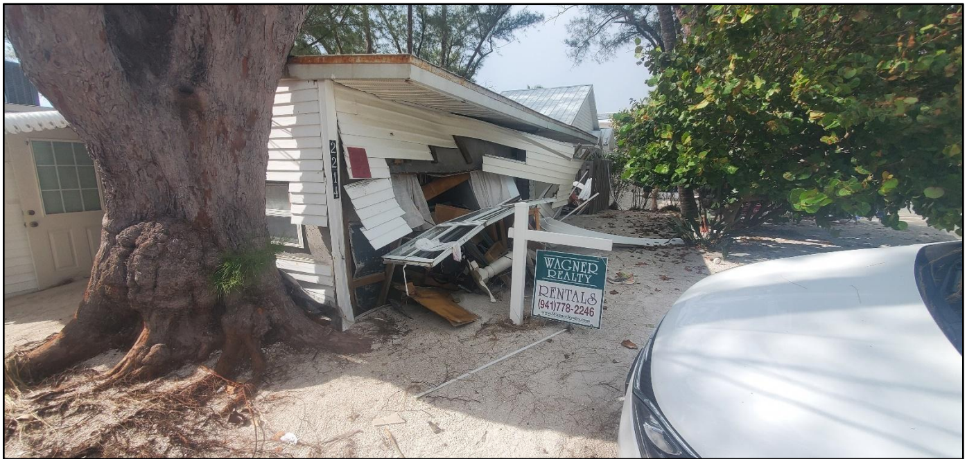
Figure 42. A single-family dwelling on Anna Maria Island with major first floor damage from Helene's storm surge near 23 rd Street North at R-28.
