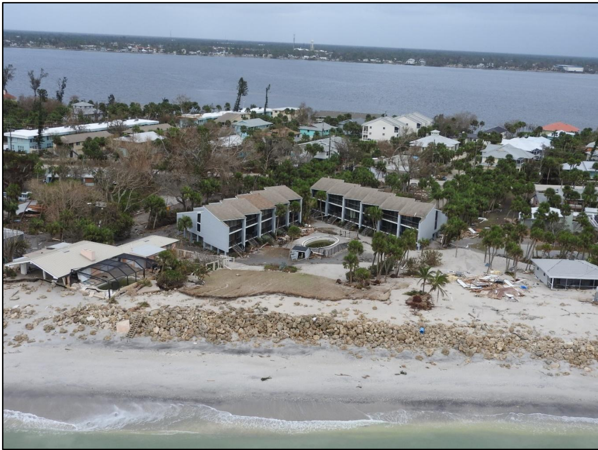
Figure 107. Major beach erosion and rock revetment damage following Milton at Englewood Beach near R-2.
