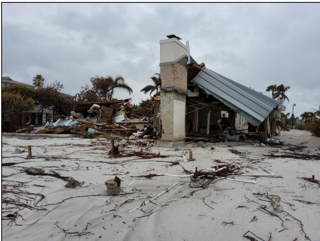
Figure 50. A single-family dwelling destroyed by Helene on northern Longboat Key near R-50.
