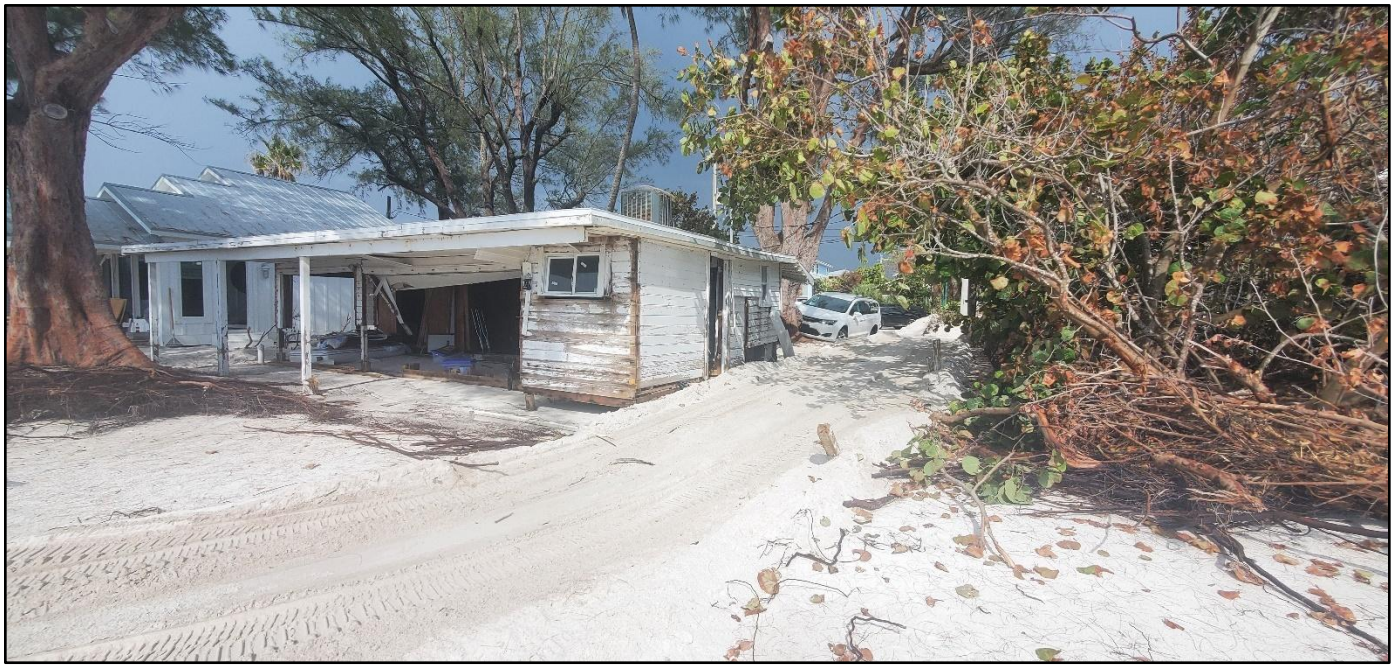
Figure 41. A gulf-fronting single-family dwelling on Anna Maria Island destroyed by Helene near 23 rd Street North at R-28.
