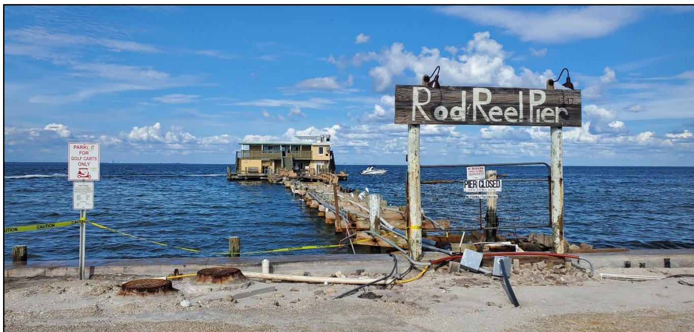
Figure 35. Major deck damage to the Rod and Reel Pier by Hurricane Helene at the northeast end of Anna Maria Island near R-1.
