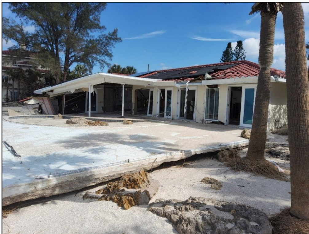
Figure 92. Single-family dwelling destroyed and a pool filled with sand by Helene on Casey Key near R-91.
