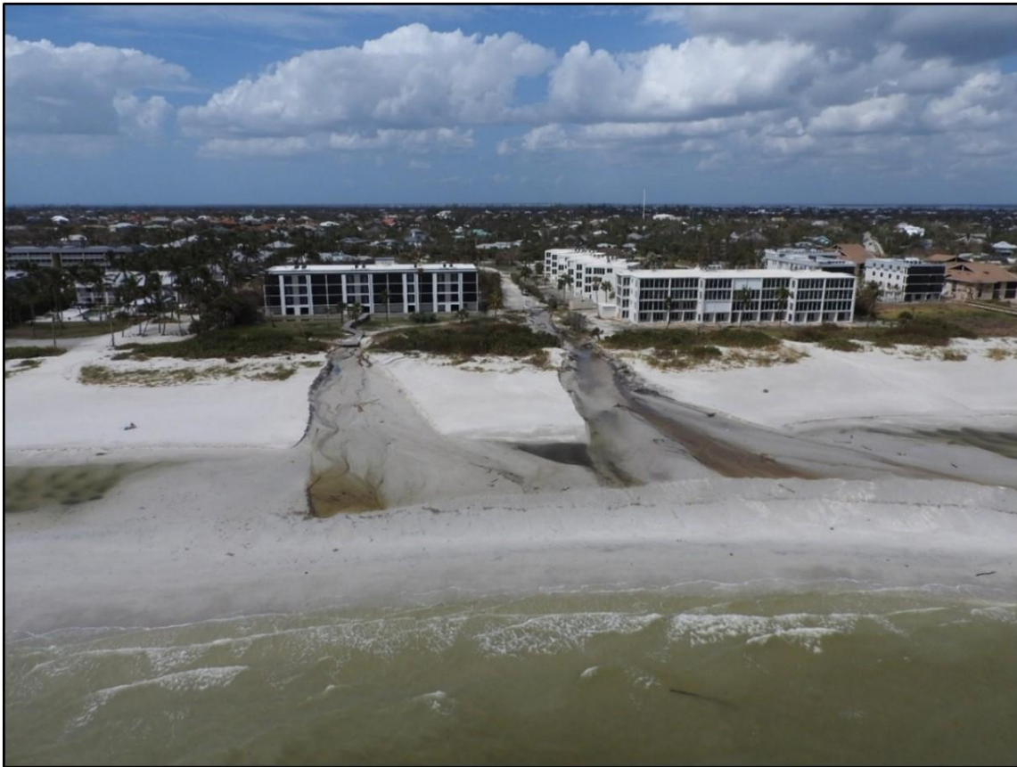
Figure 134. Storm surge discharge gullies following Milton on Sanibel Island near R-162.
