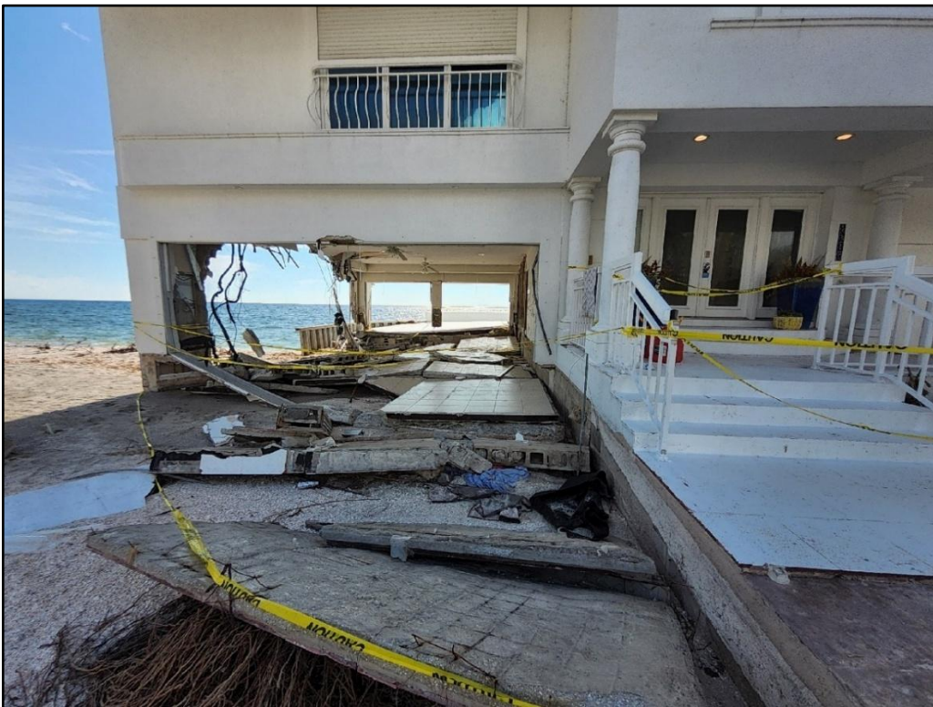
Figure 88. Major damage to single-family dwelling by Helene at Turtle Beach on Siesta Key near R-77.
