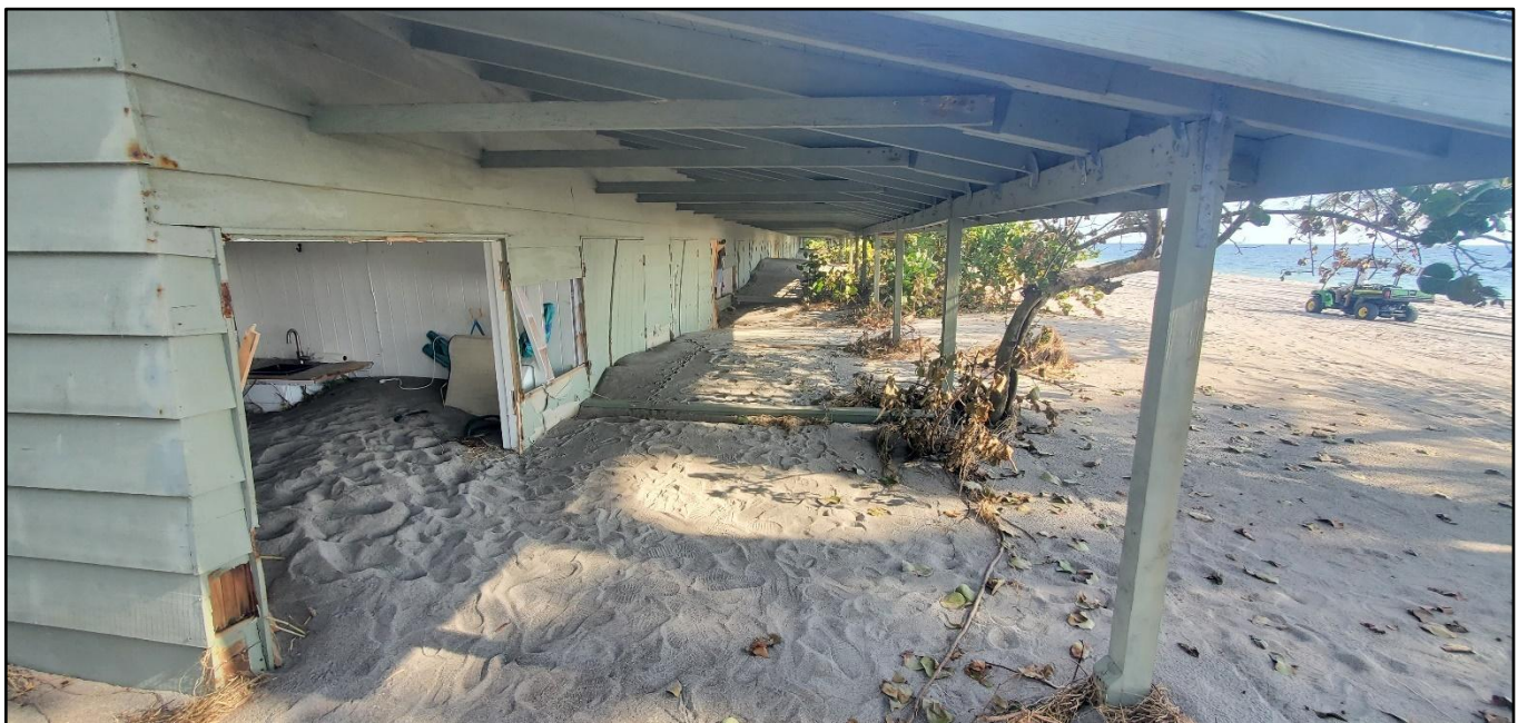
Figure 86. Damaged and sanded beach cabanas impacted by Helene’s storm surge at Turtle Beach on Siesta Key near R-71.
