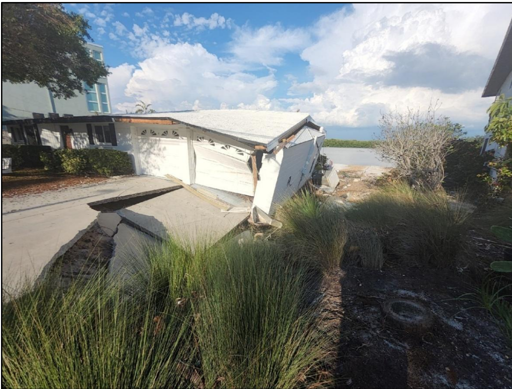
Figure 87. Dwelling destroyed by Helene at Turtle Beach on the bayside of Siesta Key near R-76.
