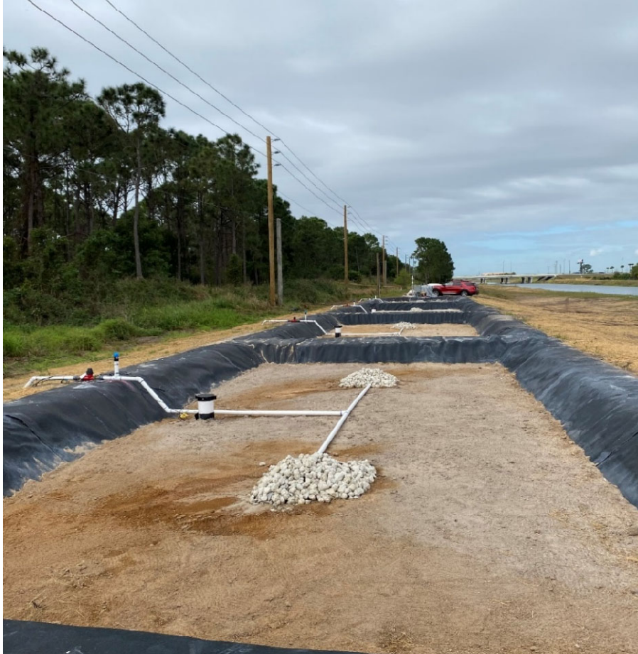
(b) Site condition after construction (new electric poles are shown in the background)
