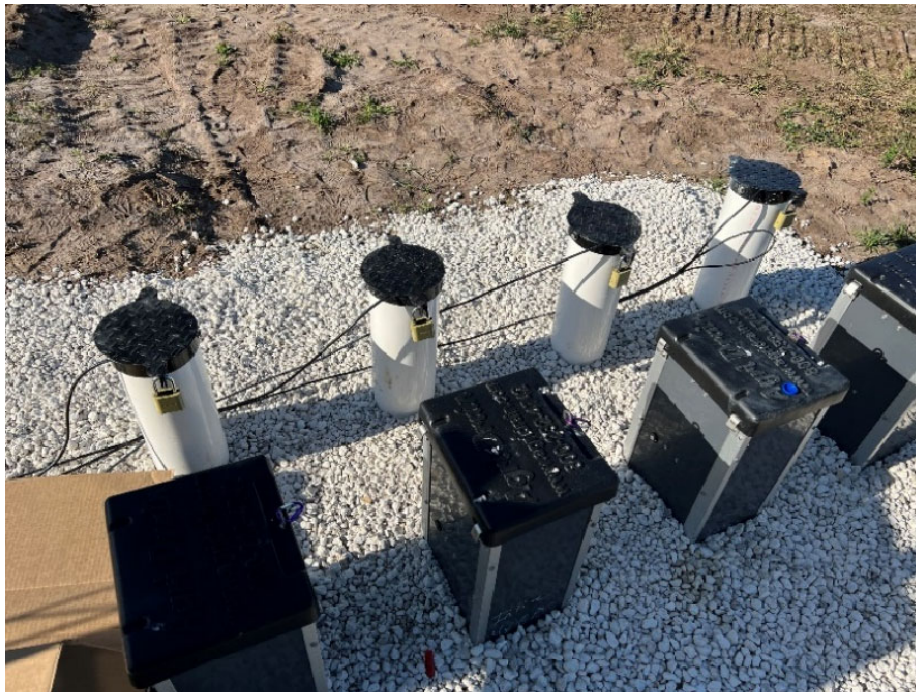
Figure 3-5: Water quality monitoring (circular enclosures) wells and drainage boxes (square boxes).
