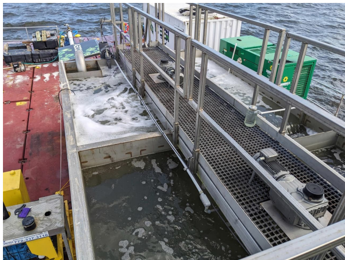
Oxygenated coagulation chamber (top compartment) with foamy surface and surface agitation from hydraulic mixing. Downstream flocculation chamber (bottom compartment).
