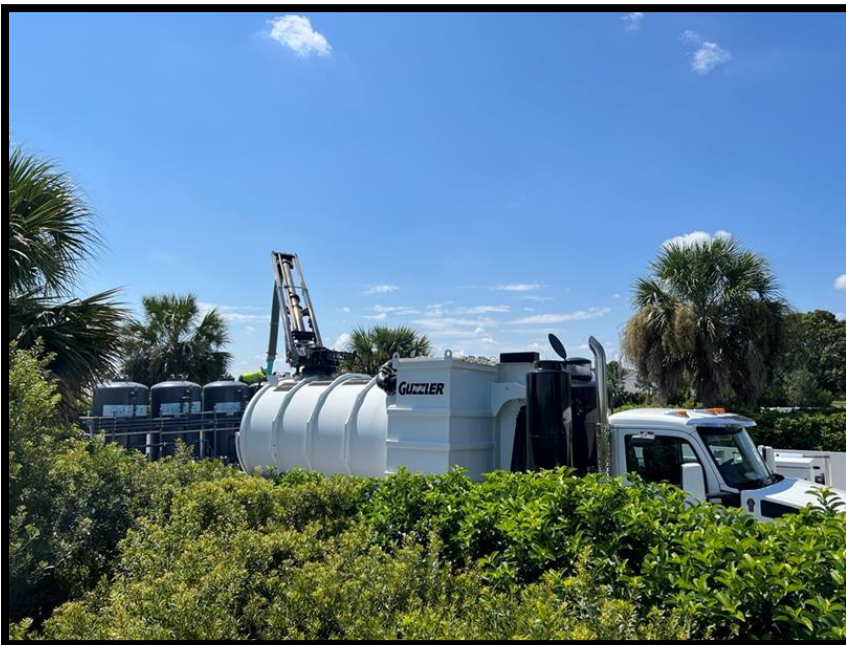
Figure 17. Media removal via vacuum truck (Task 4 – Operations).
