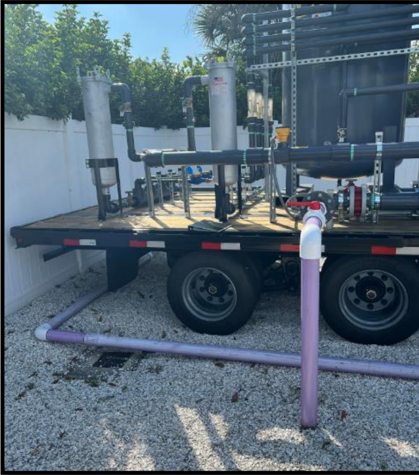
Figure 16. Inlet (vertical) and outlet (horizontal) pipes (Task 3 – Start up).
