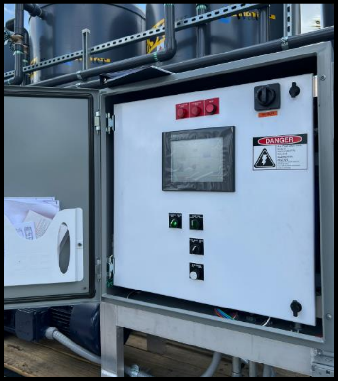
Figure 15. Image of control panel (Task 3 – Start up).
