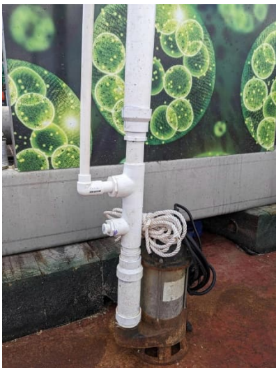
Modified sump pump for mixing and aeration with venturi air vent. Pump is secured to the harvester coagulation chamber sidewall.
