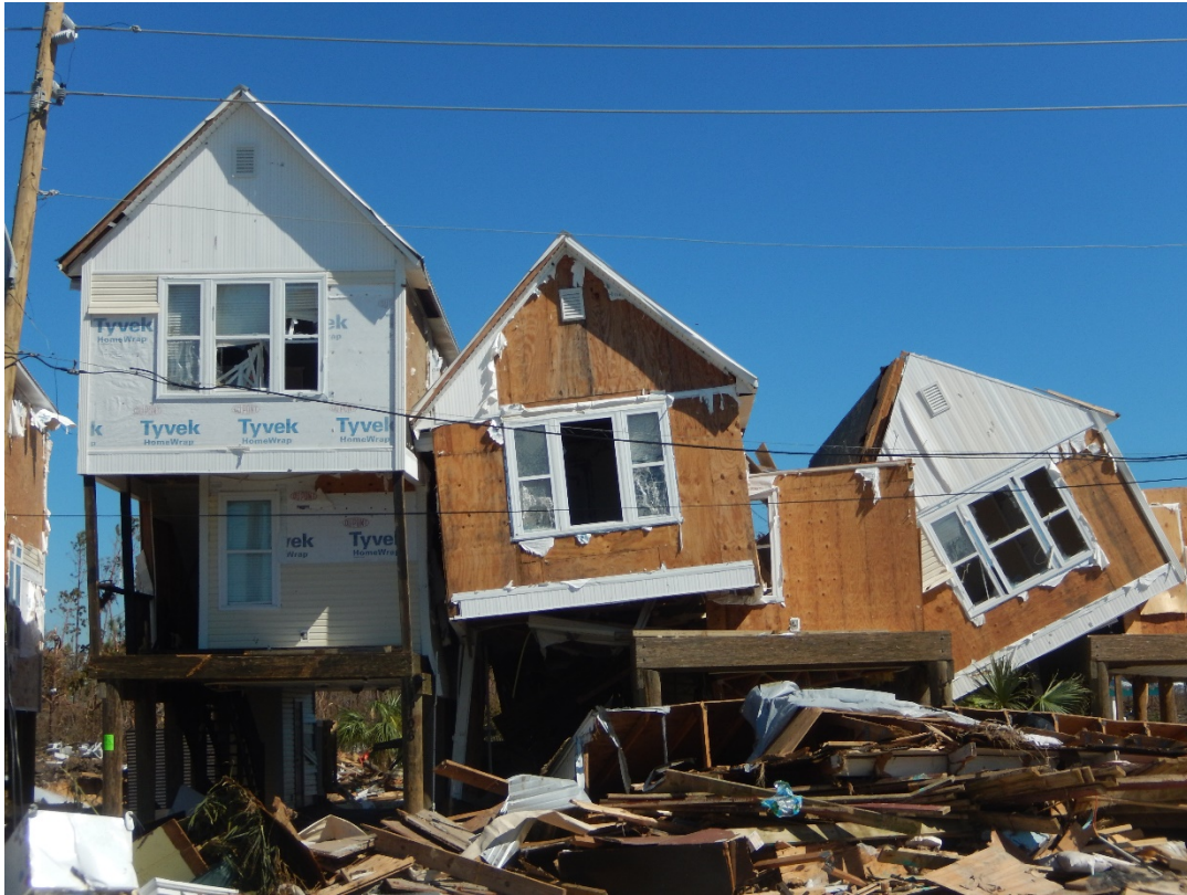
Figure 23. Beach dwellings north of U.S. 98 lifted off their foundations, R128.
