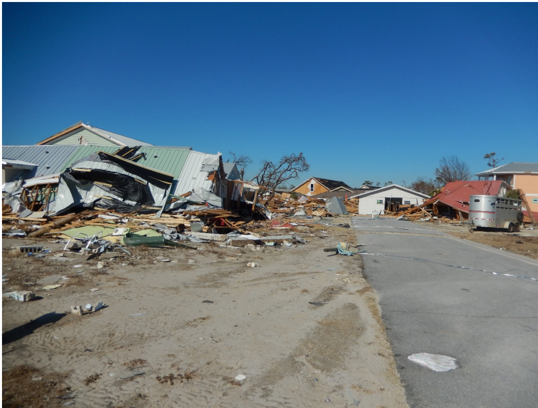
Figure 29. Buildings transported several hundred feet landward by the flood across U.S. 98 and deposited on 15 th Street, R130, Mexico Beach.
