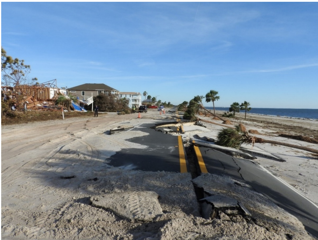
Figure 34. Segment of U.S. 98 destroyed near R139, Mexico Beach.
