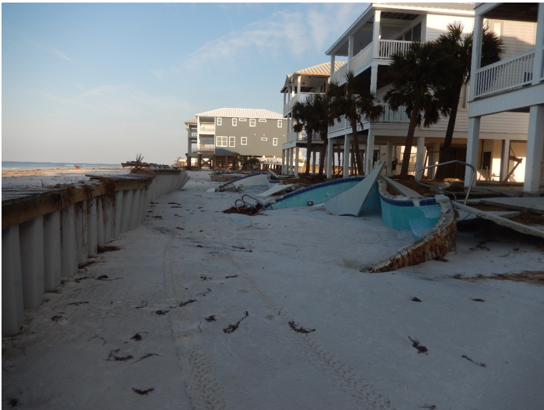
Figure 62. Major damage to bulkheads and swimming pools near R104.
