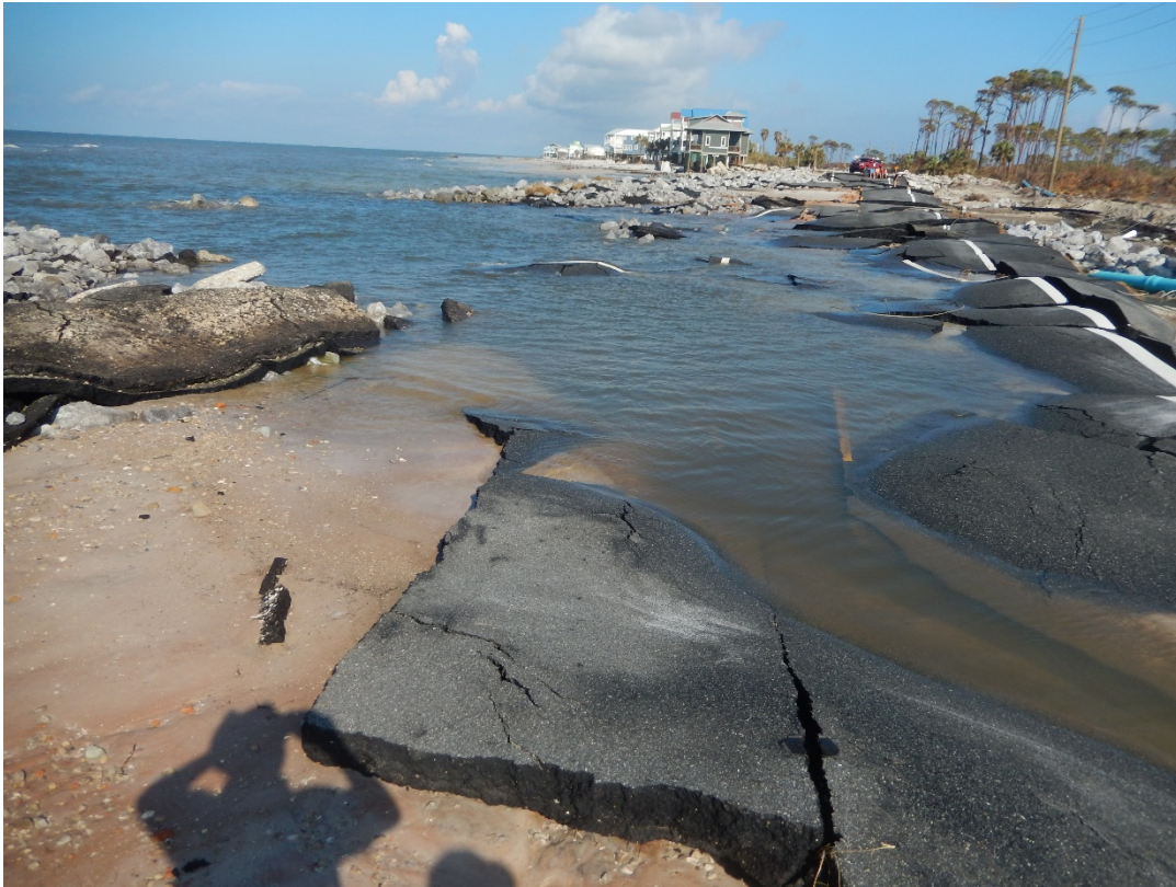
Figure 63. County Road 30E destroyed north of the Stump Hole revetment, R105.
