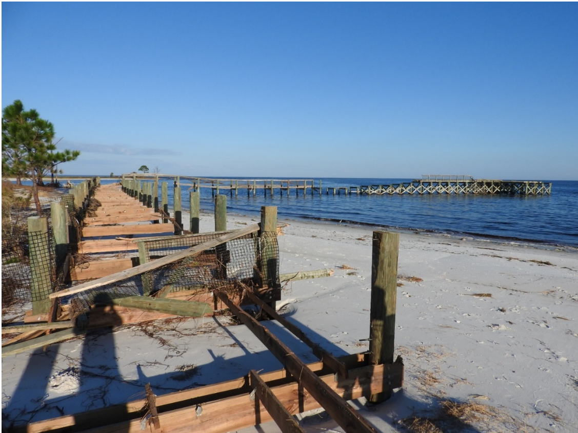
Figure 93. Fishing pier and access walkway damaged at Mashas Sands, V303.
