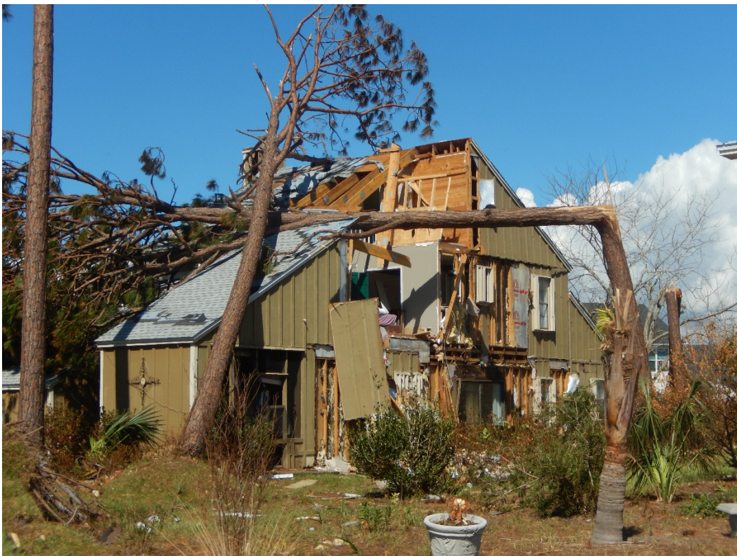
Figure 48. Major damage to dwelling due to high winds and fallen trees, Beacon Hill.
