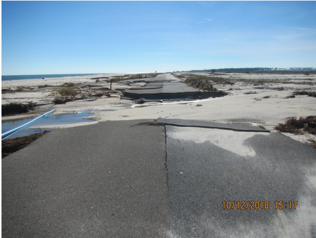
Figure 78. Dunes leveled and park road destroyed at R114, St. George Island.
