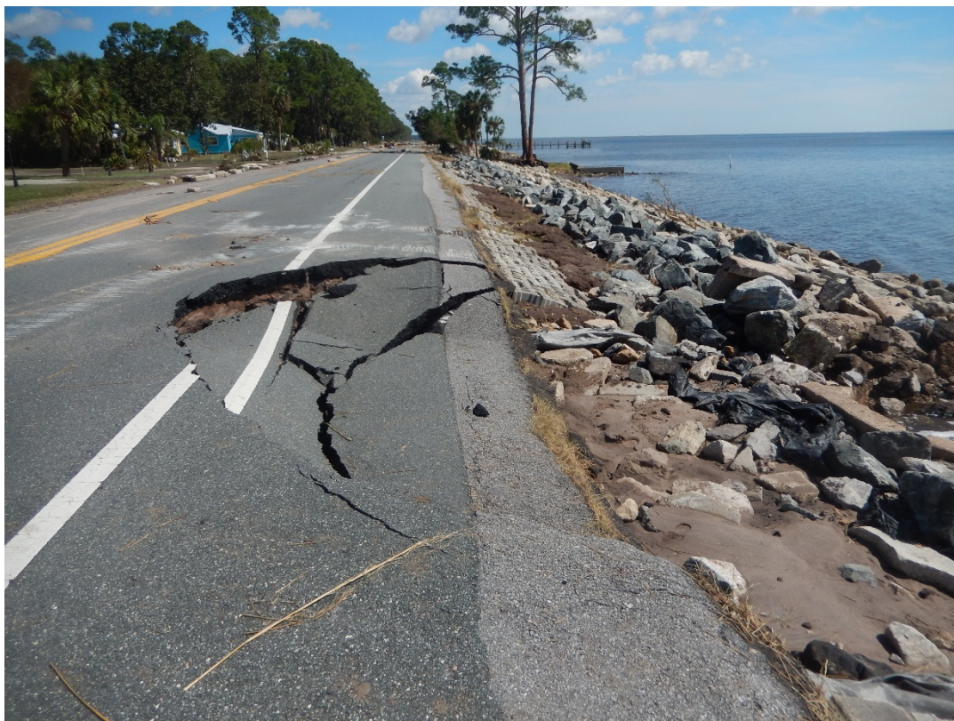
Figure 79. U.S. Highway 98 damaged near Eastpoint.
