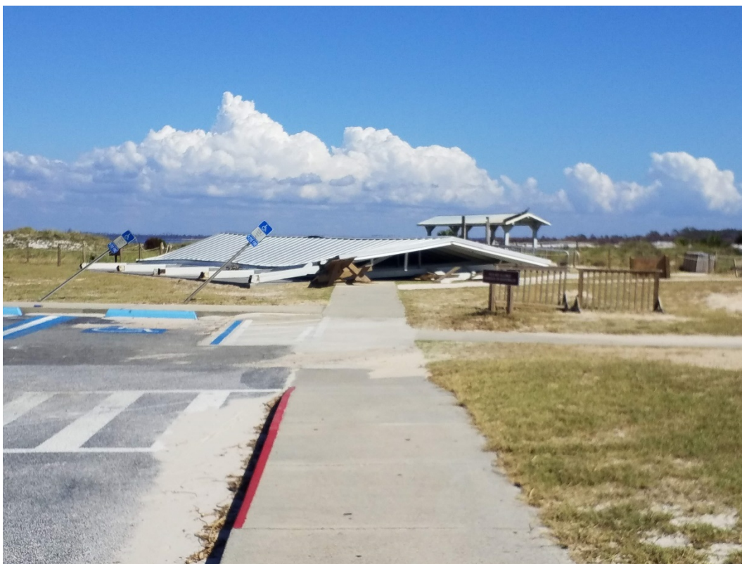
Figure 17. Collapsed pavilion near R97, St. Andrews State Park.
