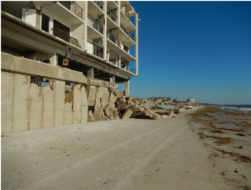
Figure 37. Over 700 feet of reinforced concrete seawall destroyed at R135.
