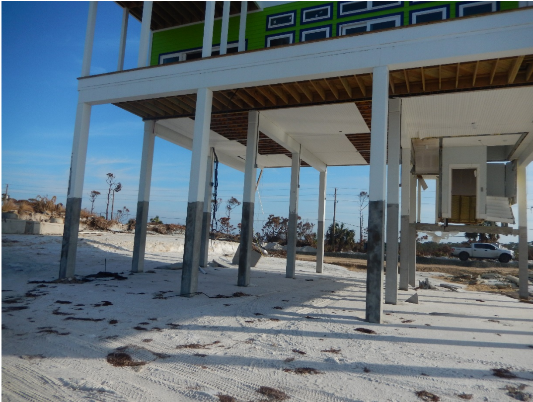
Figure 61. Over six feet of vertical loss of grade beneath structure near R104.
