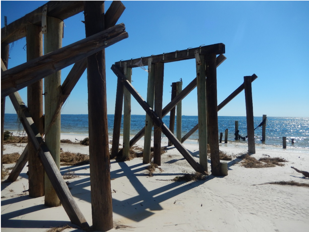
Figure 25. Mexico Beach pier destroyed near R129.
