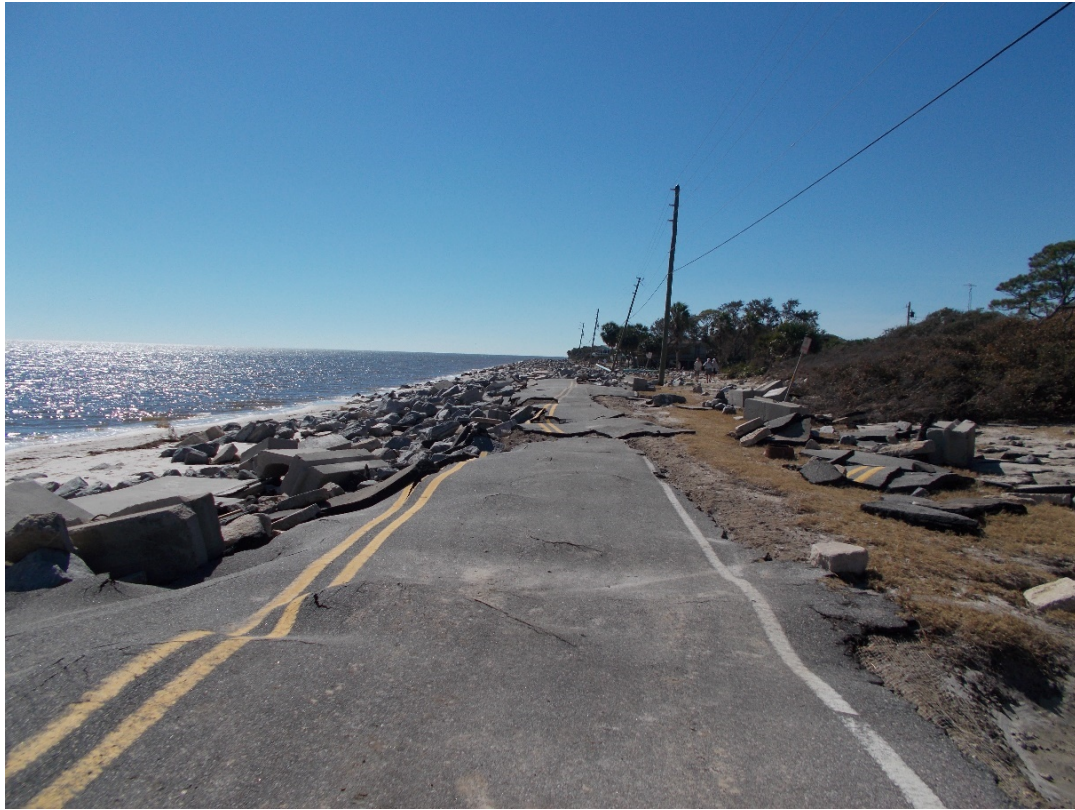
Figure 88. 3,000 feet of road and revetment destroyed between R211-R214, Southwest Cape.
