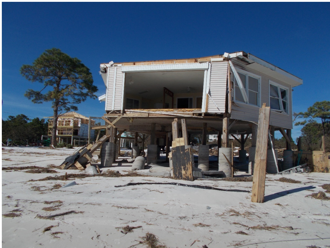
Figure 89. Dwelling destroyed near R210, Southwest Cape.
