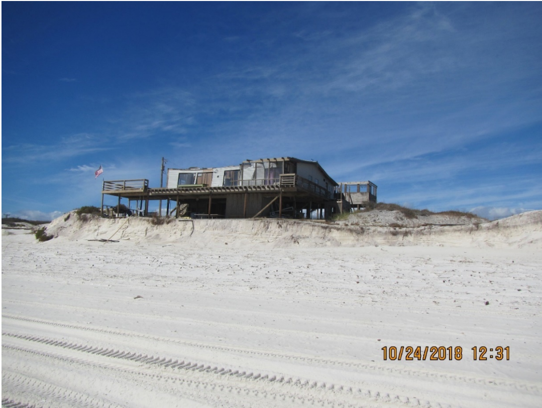
Figure 85. Dwelling destroyed near R178, Dog Island.
