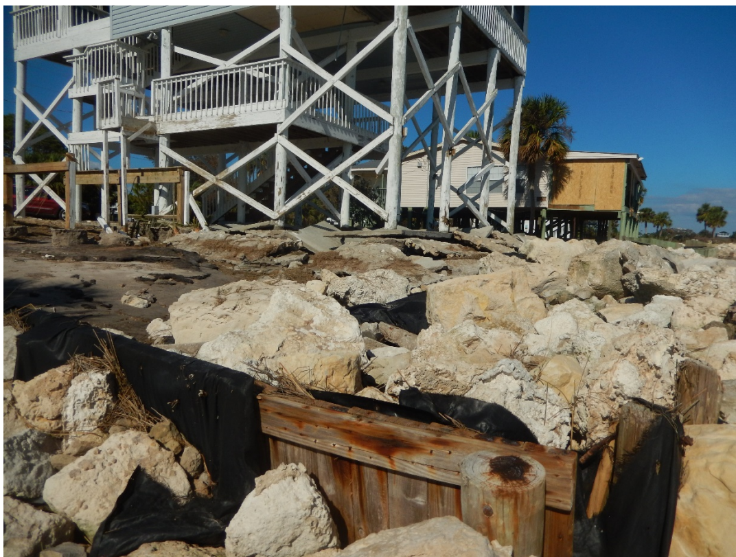
Figure 97. Rock revetment damaged and dwelling with parking slab and bracing damage at Shell Point, V361.
