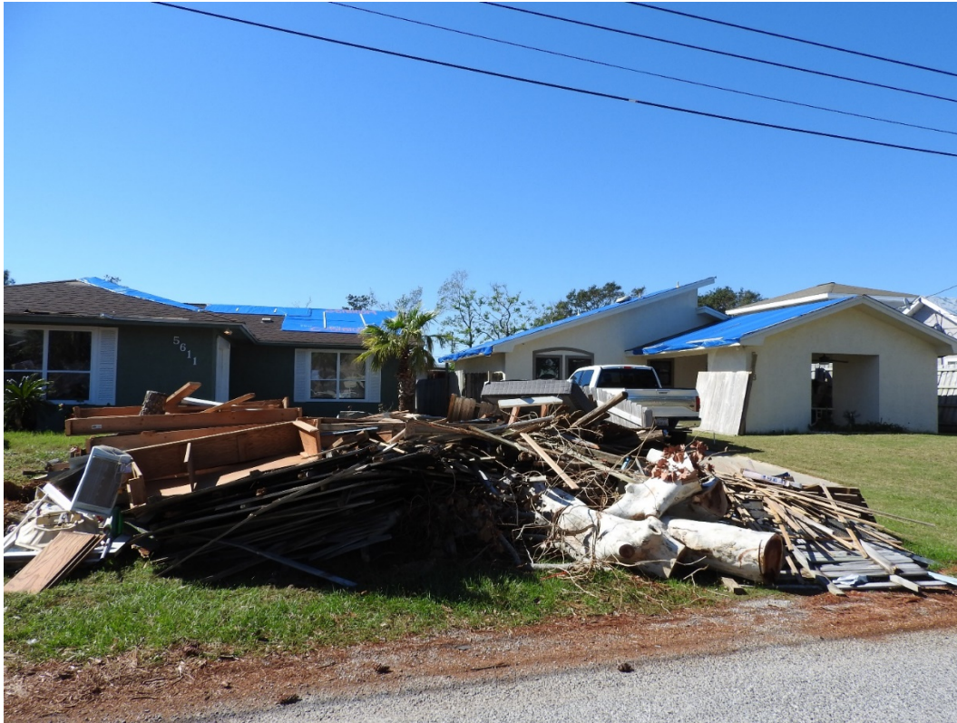
Figure 16. Roof damage on a single-family dwelling near R86, Panama City Beach.
