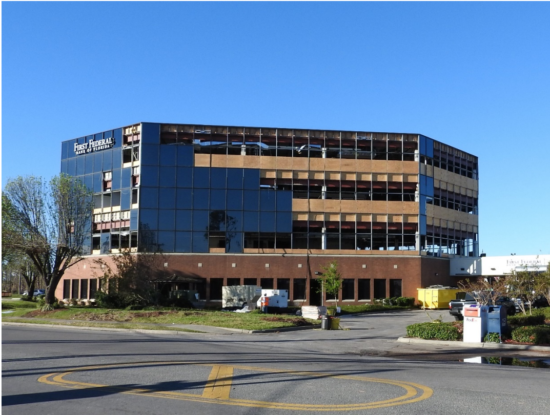
Figure 10. Bank with severe wind damage on 23rd Street, Panama City.
