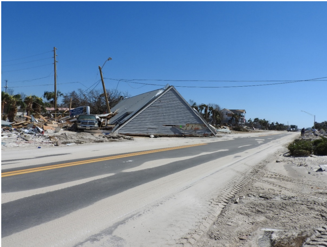
Figure 33. Roof of dwelling transported across U.S. 98 by the storm surge near R138.
