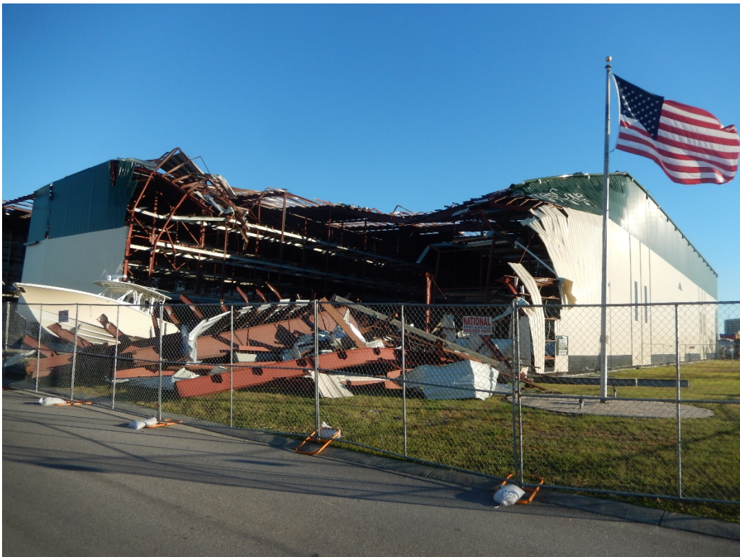
Figure 11. Dry storage marina with wind damage on Thomas Drive, Panama City Beach.
