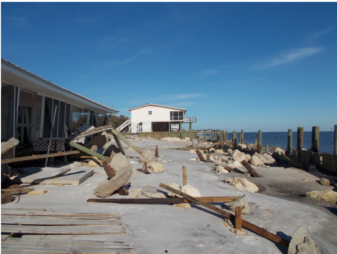
Figure 91. Dwelling and bulkhead damaged near R214.5, Southwest Cape.
