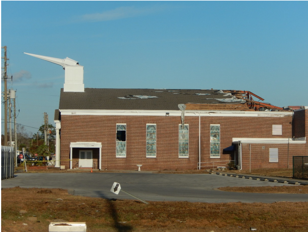
Figure 51. First Baptist Church with major wind damage, Port St. Joe.
