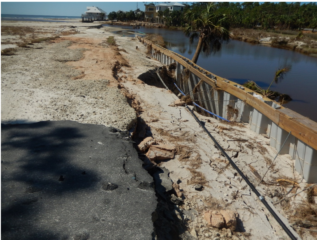
Figure 68. Bulkhead on Money Bayou damaged, R141.
