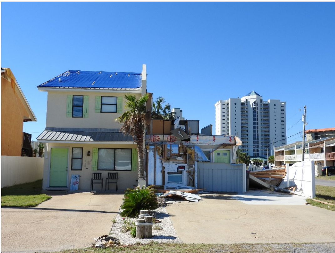
Figure 15. Roof damage and destroyed dwelling near R82, Panama City Beach.
