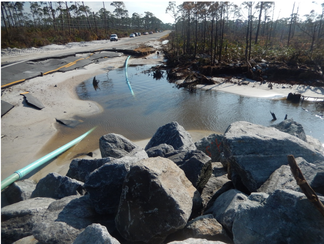
Figure 64. County Road 30E destroyed south of the Stump Hole revetment, R107.
