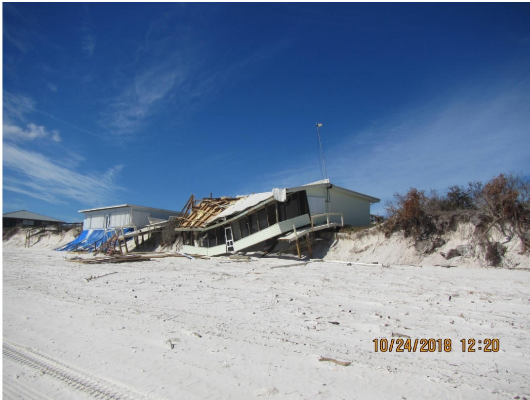
Figure 86. Dwelling destroyed near R179, Dog Island.
