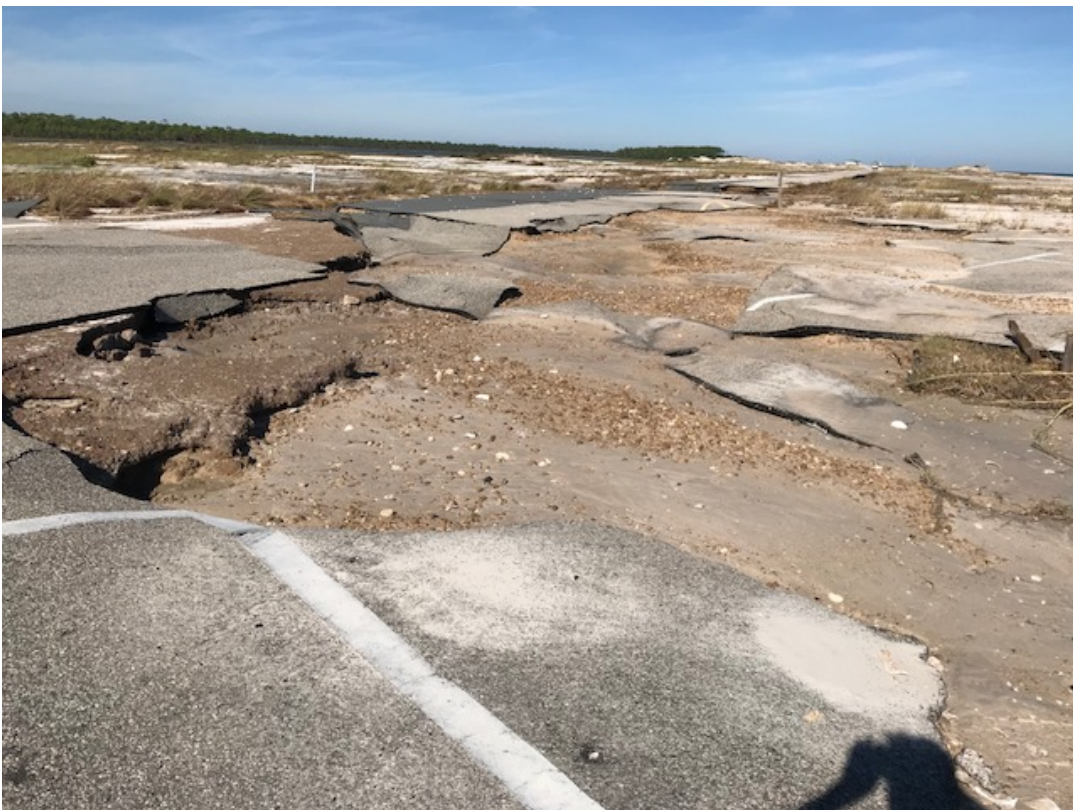
Figure 77. State park road destroyed near R108, St. George Island.
