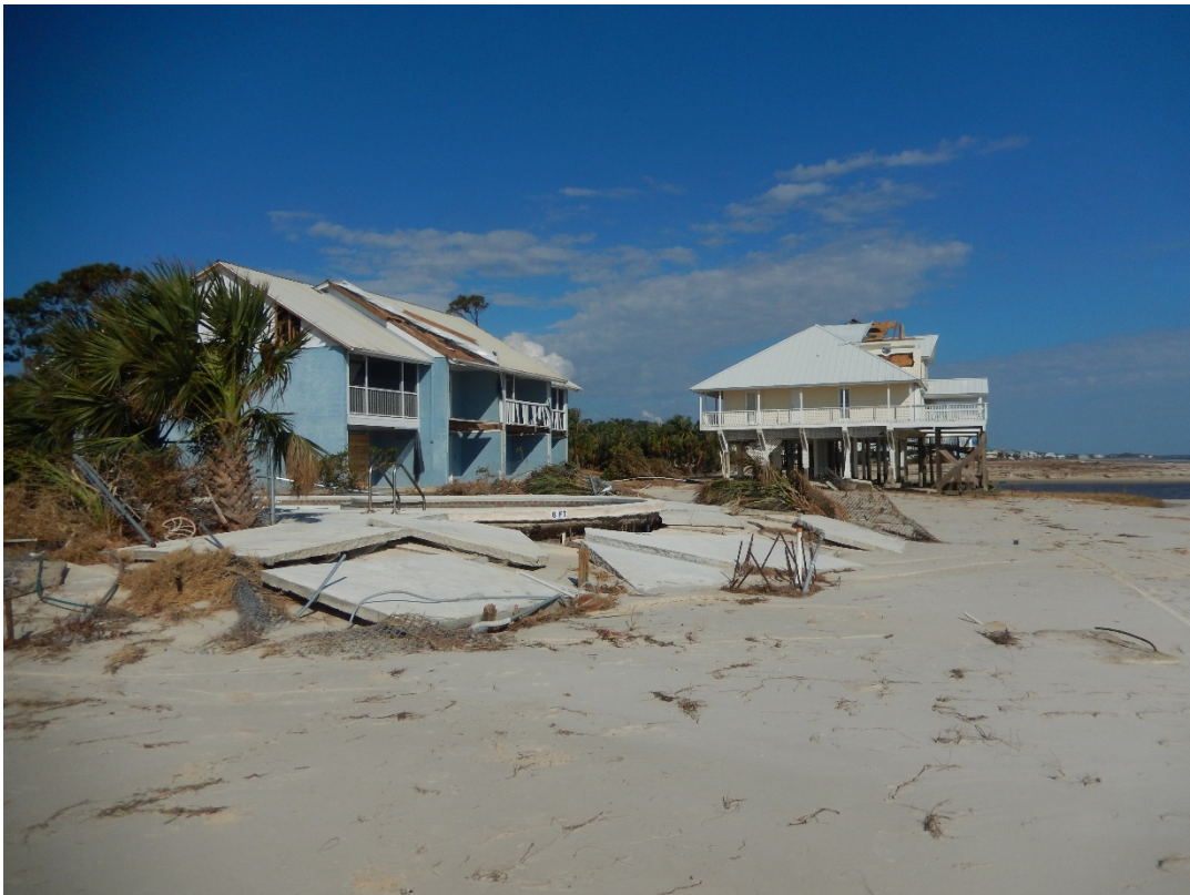
Figure 66. Storm surge damages at Money Bayou, R140.
