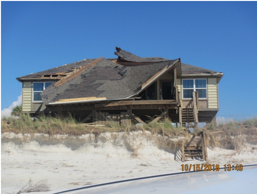
Figure 57. Major roof damage due to high winds near R85, St. Joseph Peninsula.
