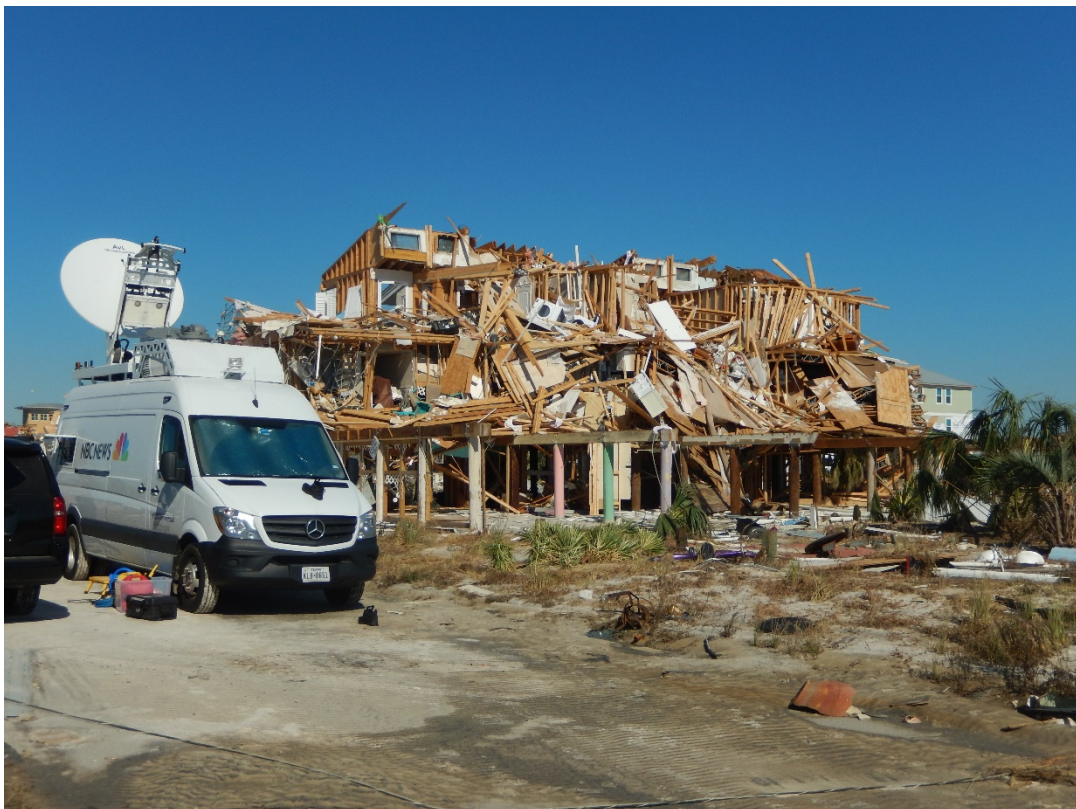
Figure 28. Pile-supported multifamily dwelling destroyed near R129, Mexico Beach.
