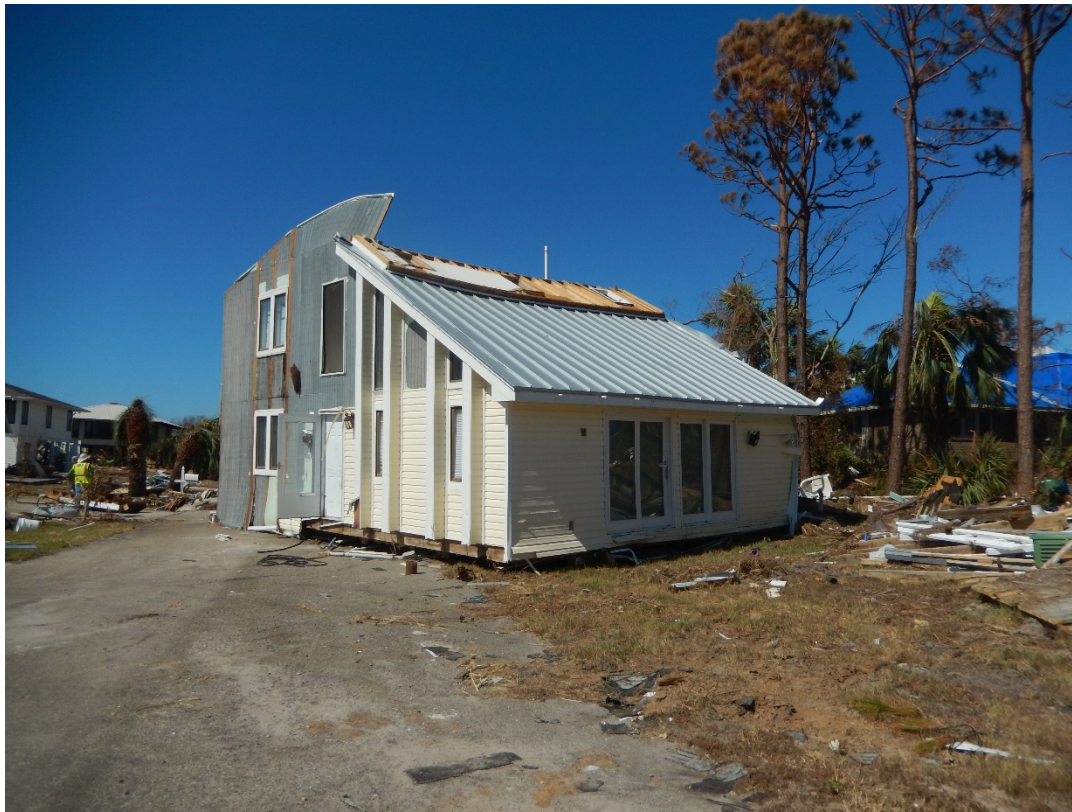
Figure 44. Dwelling transported by storm surge onto Trade Winds Dr. near R6, Beacon Hill.
