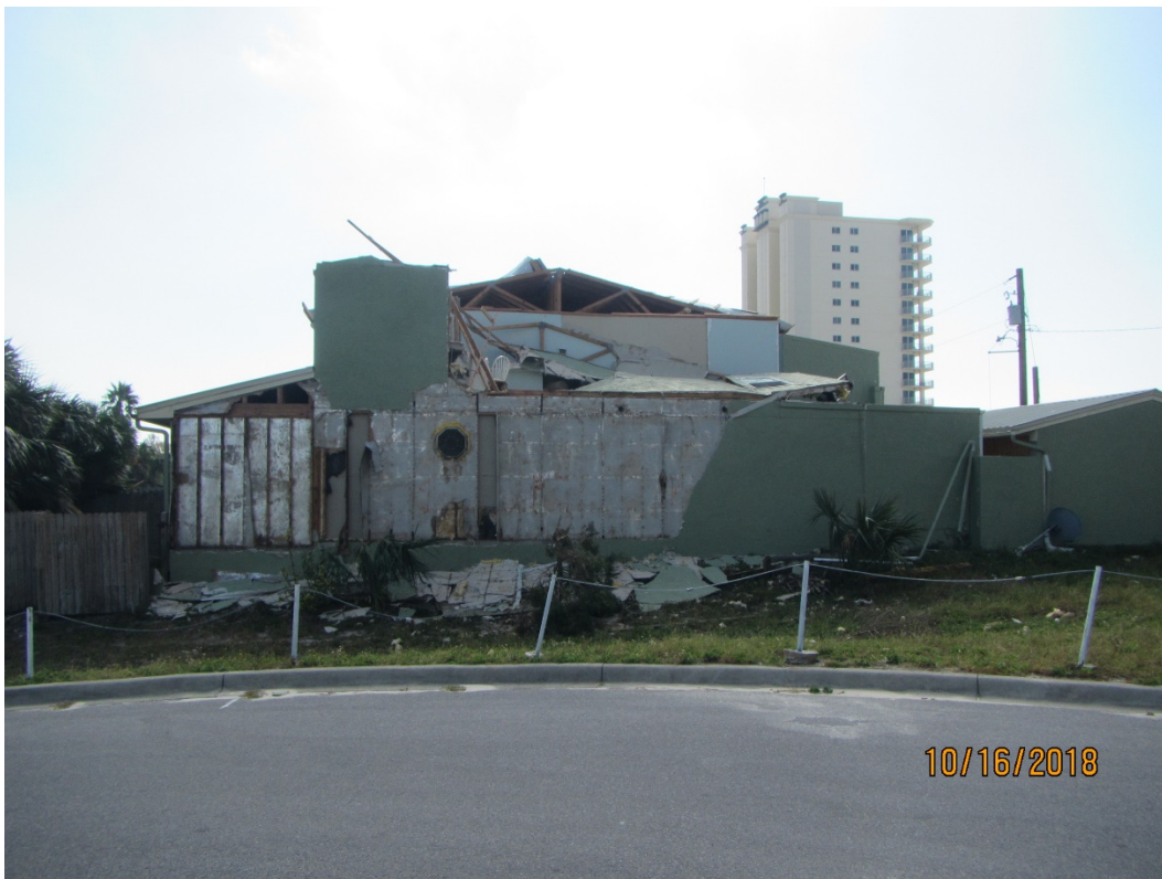
Figure 13. Wind damages on a multifamily dwelling near R73, Panama City Beach.
