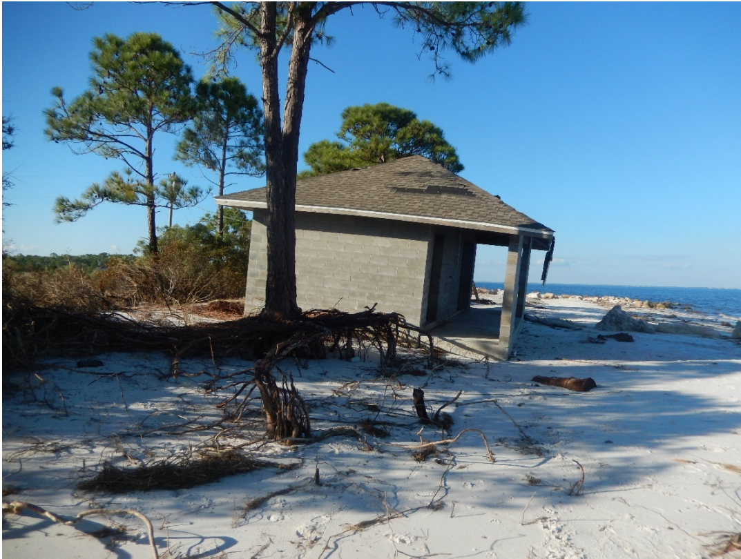
Figure 94. Bathhouse destroyed at Mashers Sands, V314.
