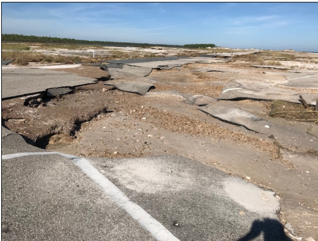
Figure 90. State park road destroyed near R108, St. George Island.
