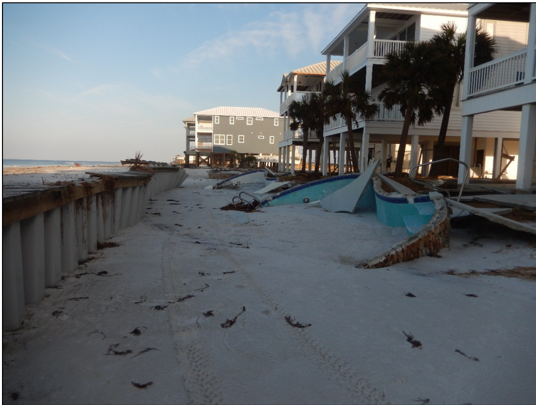
Figure 73. Major damage to bulkheads and swimming pools near R104.
