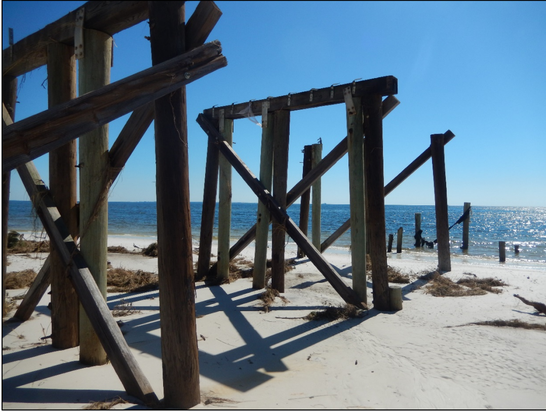
Figure 30. Mexico Beach pier destroyed near R129.
