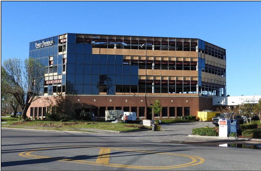
Figure 15. Bank with severe wind damage on 23rd Street, Panama City.
