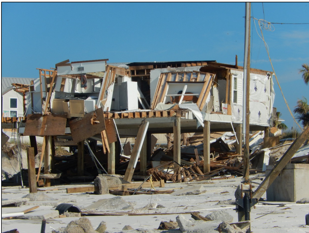
Figure 70. Pile-supported dwelling destroyed near R97.5, St. Joseph Peninsula.
