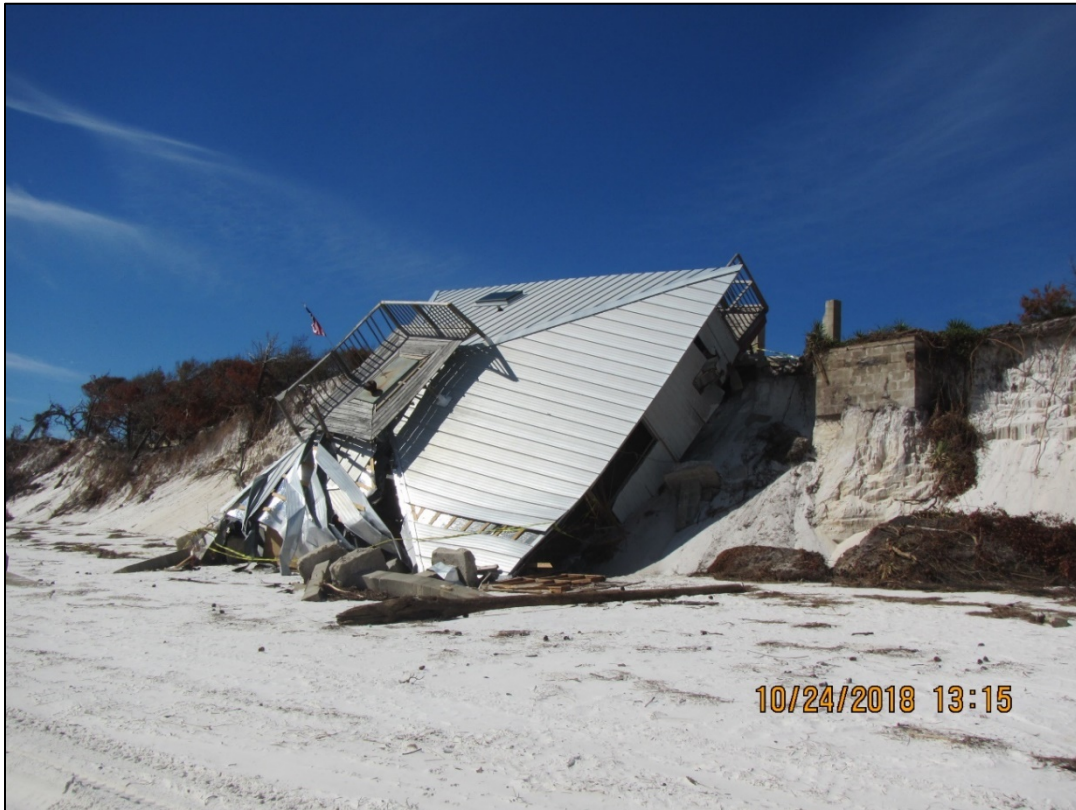
Figure 93. Dwelling destroyed near R173, Dog Island.
