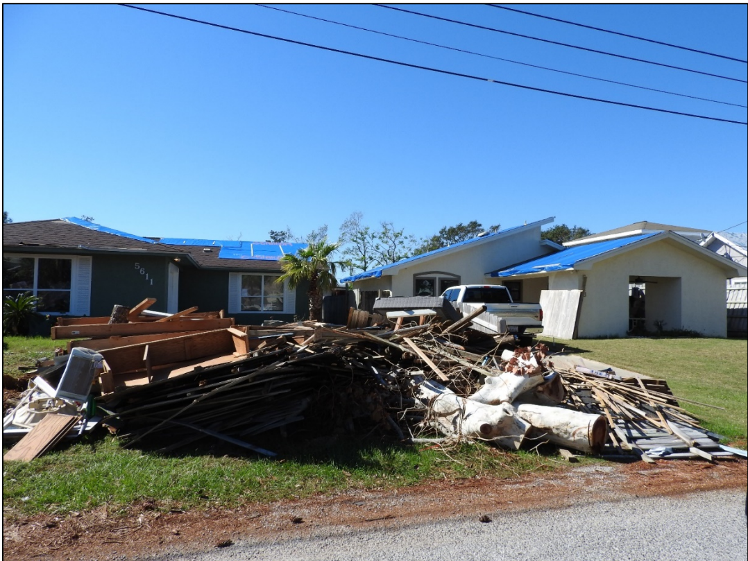
Figure 20. Roof damage on a single-family dwelling near R86, Panama City Beach.
