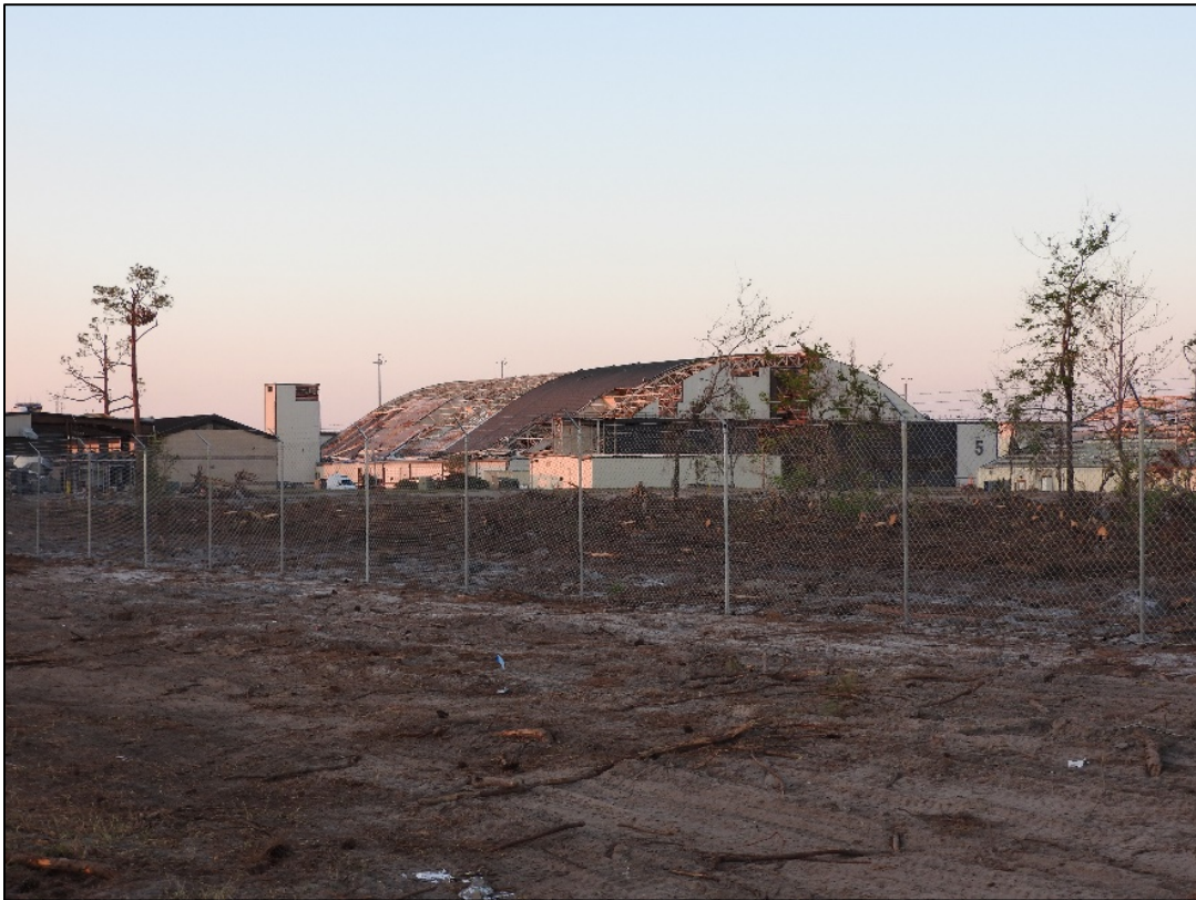
Figure 22. Tyndall Air Force Base, aircraft hangar damage.
