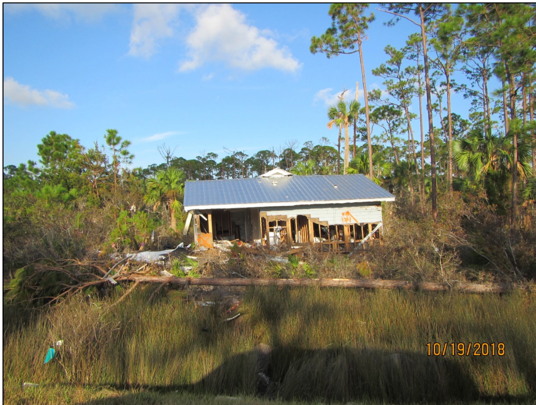
Figure 67. Destroyed dwelling transported across S.R.30A by the storm surge, St. Joseph Bay.
