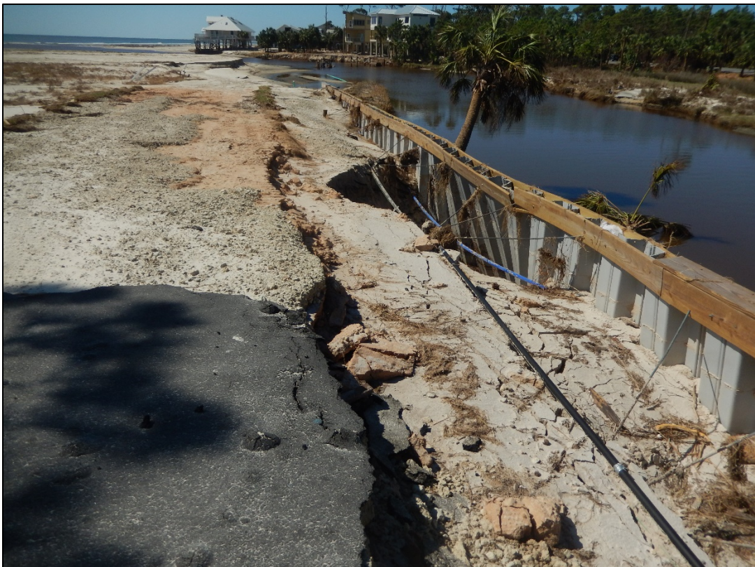
Figure 78. Bulkhead on Money Bayou damaged, R141.
