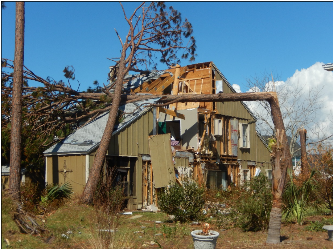
Figure 62. Major damage to dwelling due to high winds and fallen trees, Beacon Hill.
