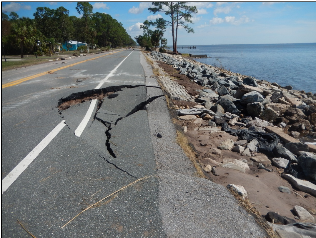
Figure 92. U.S. Highway 98 damaged near Eastpoint.
