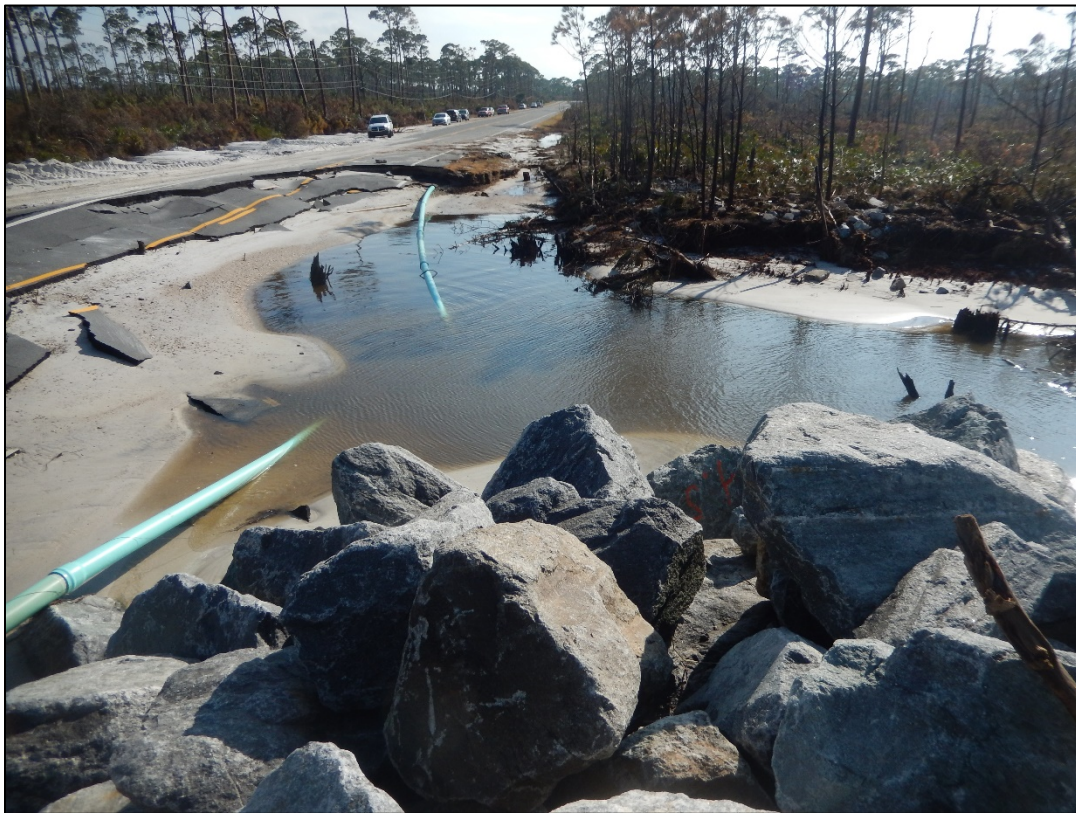
Figure 75. County Road 30E destroyed south of the Stump Hole boulder mound, R107.
