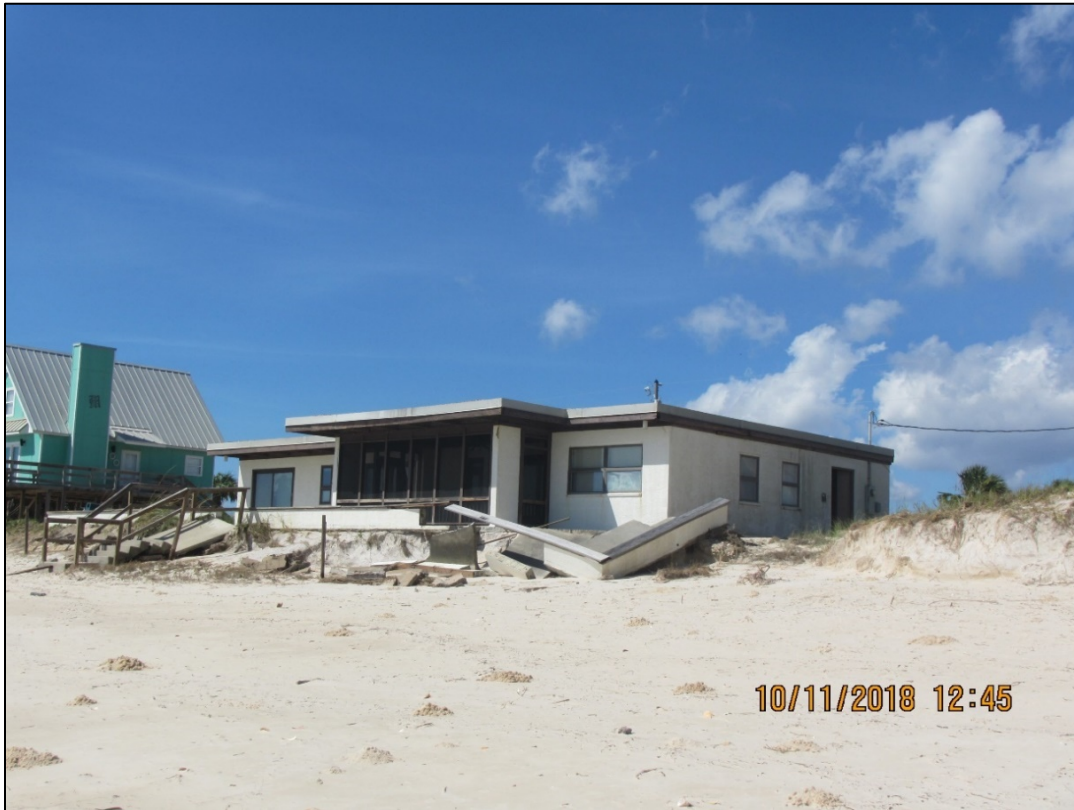
Figure 89. Dwelling damaged near R78, St. George Island.
