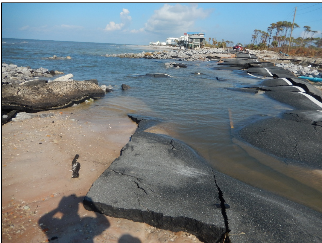
Figure 74. County Road 30E destroyed north of the Stump Hole boulder mound, R105.
