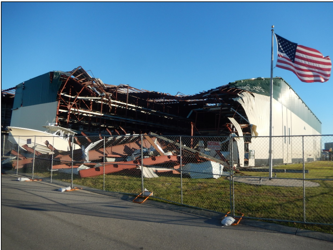
Figure 16. Dry storage marina with wind damage on Thomas Drive, Panama City Beach.
