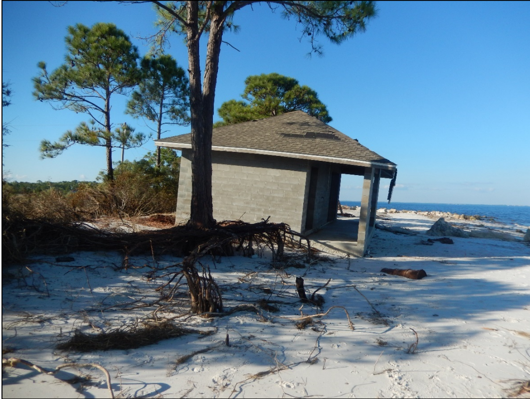
Figure 105. Bathhouse destroyed at Mashas Sands, V314.
