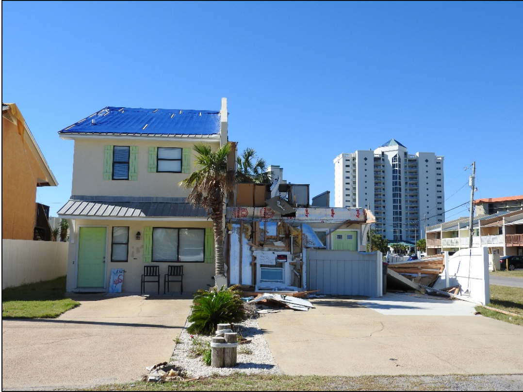
Figure 19. Roof damage and destroyed dwelling near R82, Panama City Beach.
