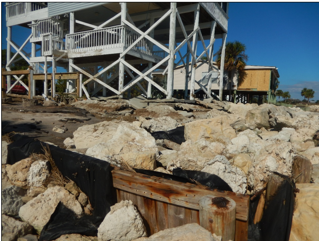
Figure 108. Rock revetment damaged and dwelling with parking slab and bracing damage at Shell Point, V361.
