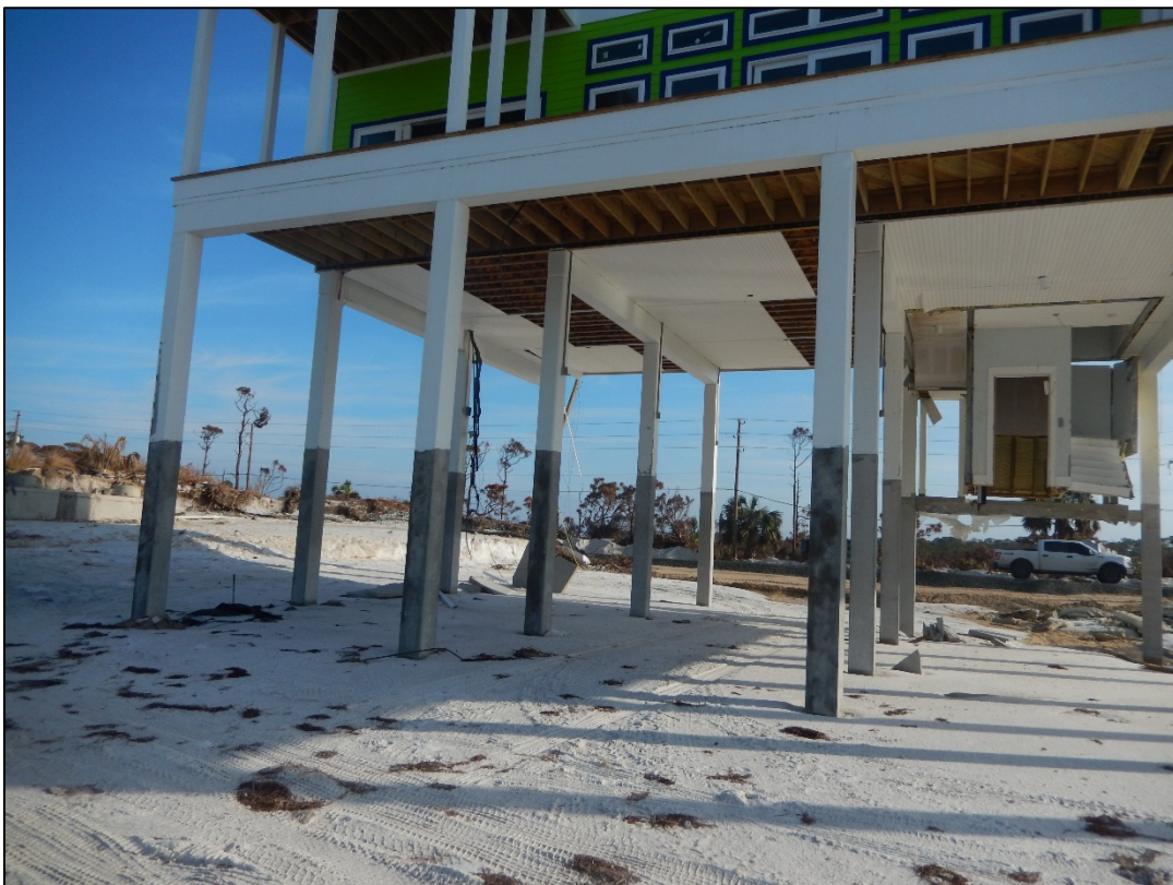
Figure 72. Over six feet of vertical loss of grade beneath structure near R104.
