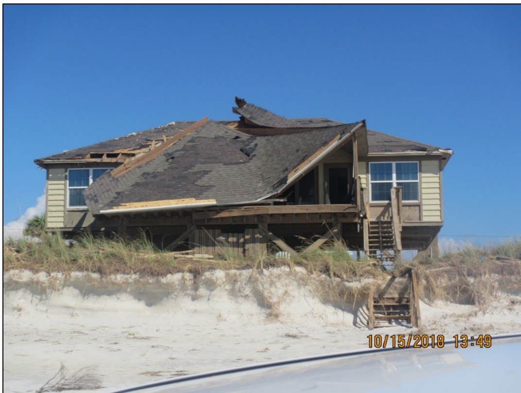
Figure 68. Major roof damage due to high winds near R85, St. Joseph Peninsula.
