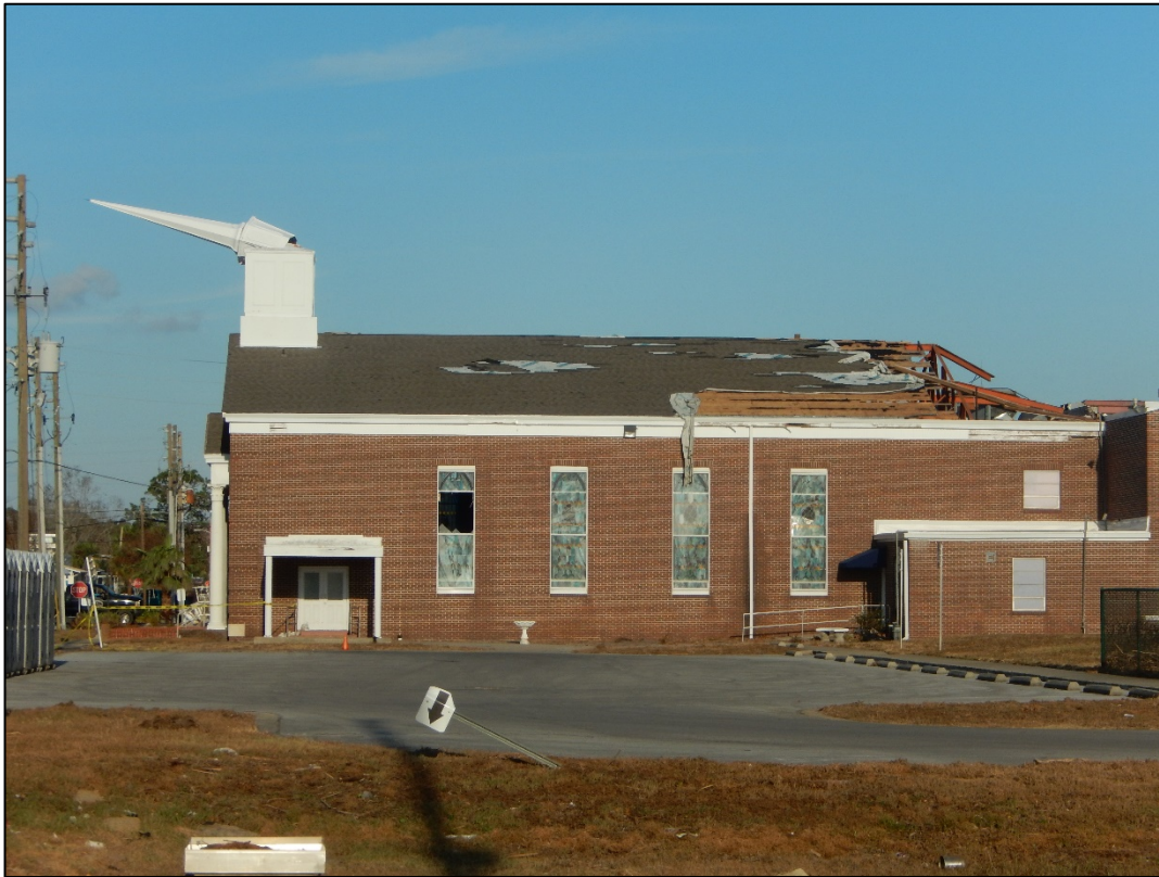
Figure 65. First Baptist Church with major wind damage, Port St. Joe.
