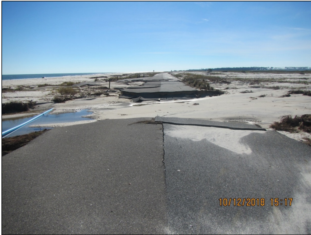
Figure 91. Dunes leveled and park road destroyed at R114, St. George Island.
