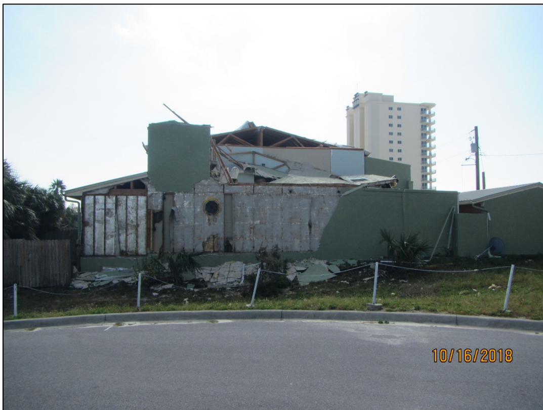
Figure 18. Wind damages on a multifamily dwelling near R73, Panama City Beach.
