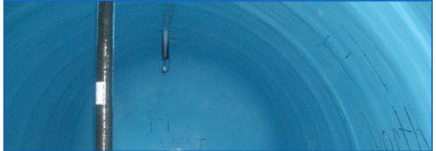
Ball Float or Vent Flow Restrictor; Installed
