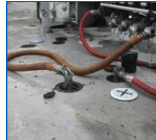
Fuel Truck Fueling UST
