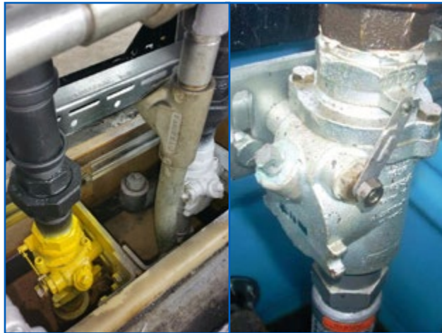
Shear Valves Secured to Brackets
