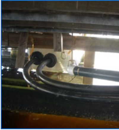
DW-semi-rigid Pipe Over Water
