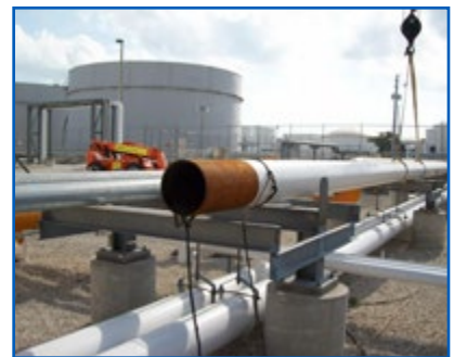
Bulk Product Piping
