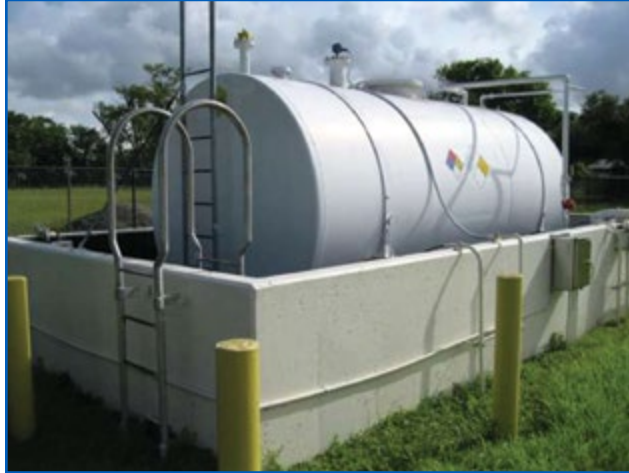
Horizontal SW-AST within Secondary Containment
