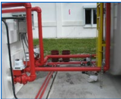
Piping for Shop Fabricated AST
