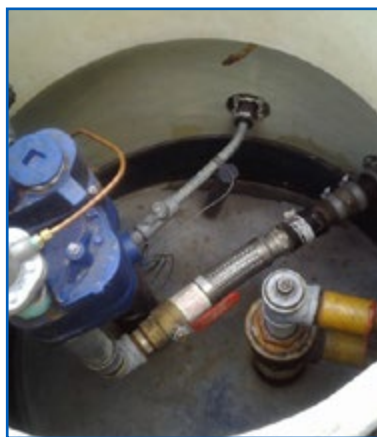
Flex Pipe Fitting in Pump/Piping Sump
