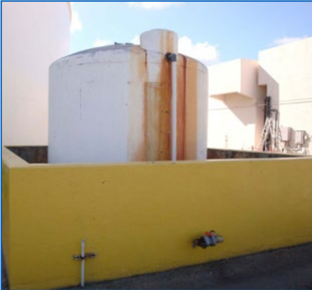
Check Drain Valves for Leaks. Ensure they are Locked when Not in Use
