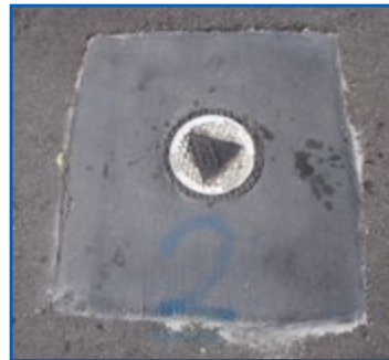
Installed MW with Color-coded Cover
