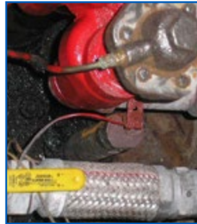
Sensor Float in Pump Sump
