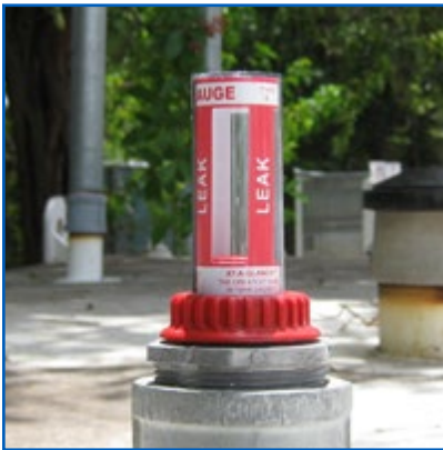
AST Float Gauge Installed
