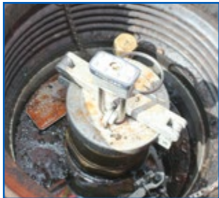
Fill Pipe with Fill Cap Secured
