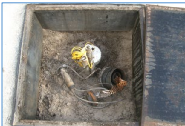
Old Discriminating Electronic Probe Pulled Out of Well, Pending Replacement
