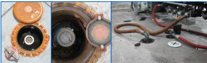
Stage I Vapor Recovery Color-coded Sump
