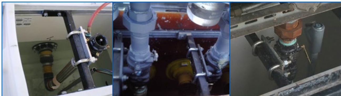
Various Shear Valves Installed at Correct Height. Note Valve Anchoring to Dispenser Box
