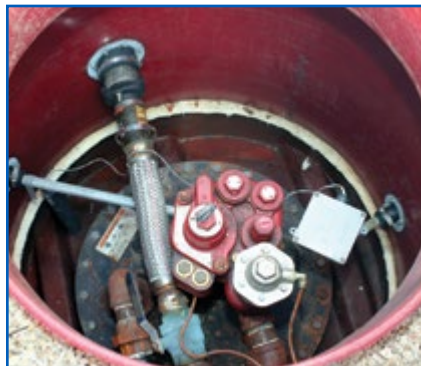
Piping, Pump and LLD inside Sump
