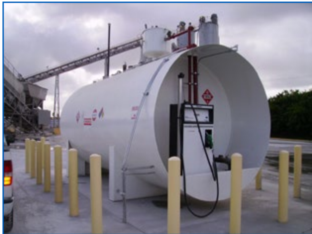
DW-AST with Dispenser within Containment
