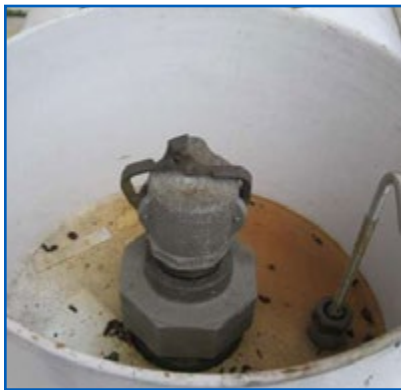
AST Spill Containment on Tank Top
