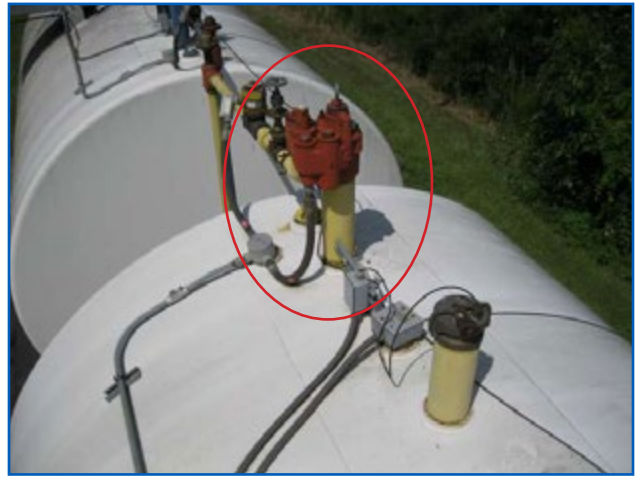
AST with STP connection on top of the Tank
