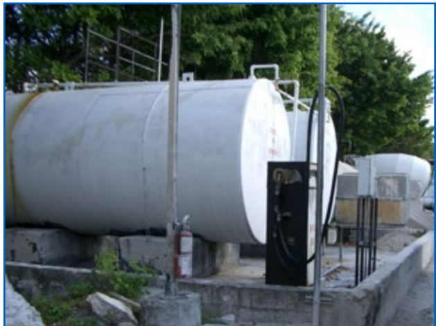
SW-AST with Dispenser within Secondary Containment
