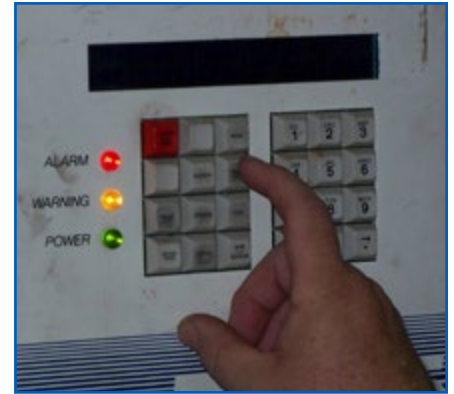
Installed Audio/Visual/Print Console
