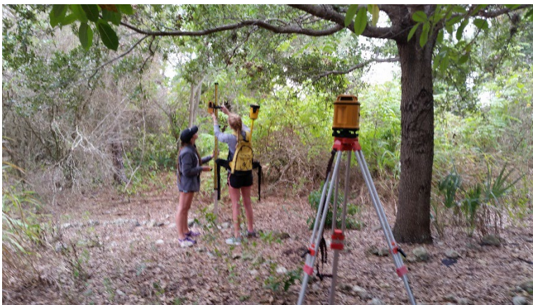
Mapping elevations of islands can give insights into appropriate vegetation for restoration work
