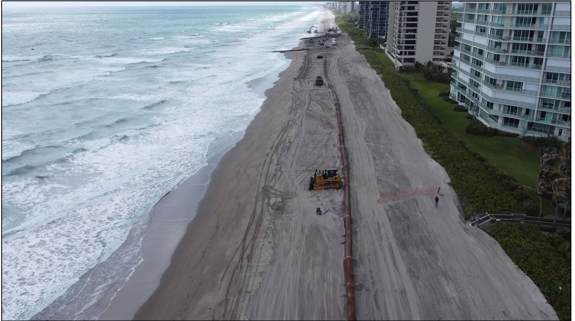
The federal (USACE) St. Lucie County Coastal Storm Risk Management Project being constructed near R-99, in April 2022. Photo courtesy of Joshua Revord P.E., with St. Lucie County. See additional construction photos of beach nourishment projects.
