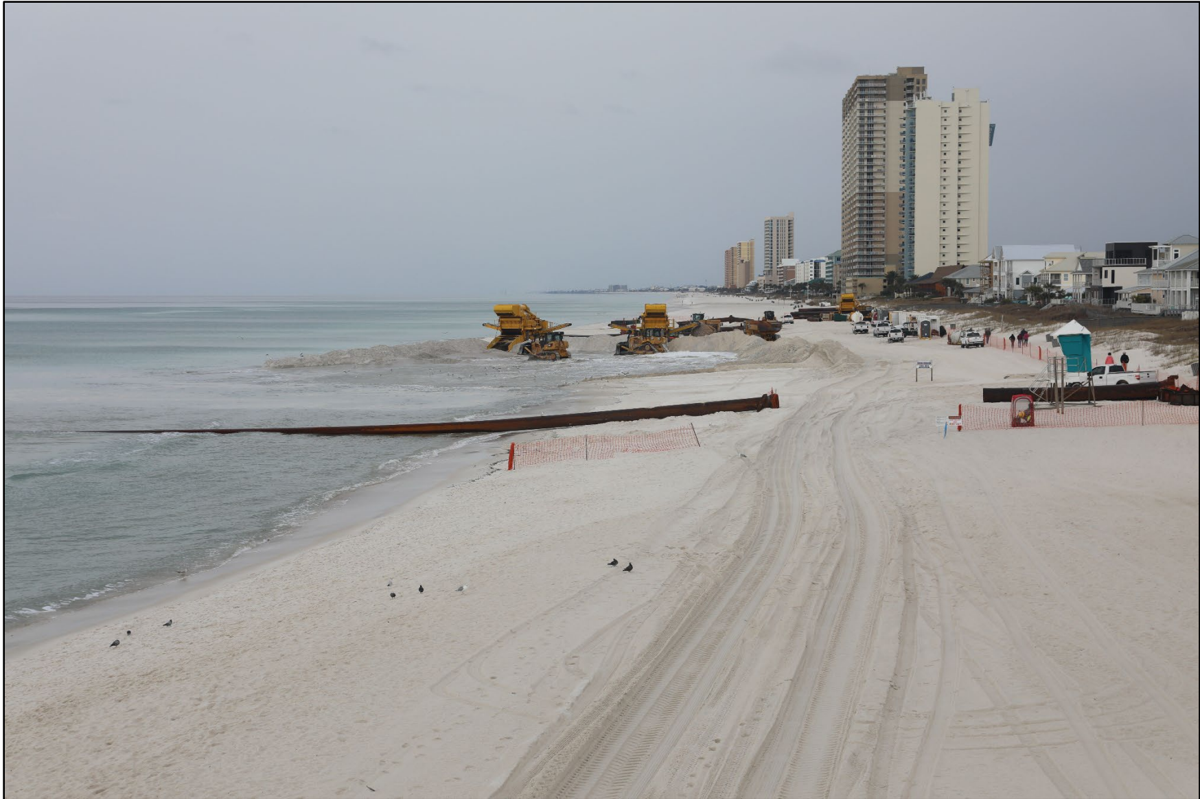
Panama City Beaches Shore Protection Project under construction (near R39) in February 2022. Photo courtesy of Lisa Armbruster with Bay County. See additional construction photos of beach nourishment projects.
