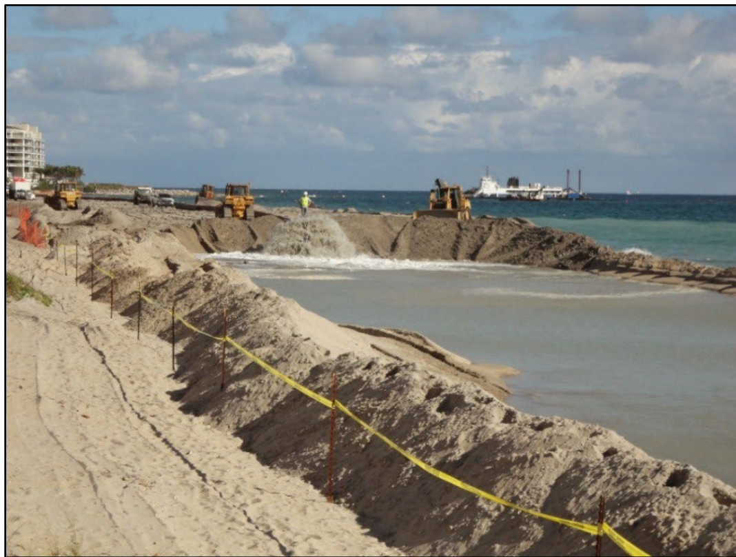
Figure 14. South Boca Raton beach nourishment project (2013) using sand from offshore sources. Photo courtesy of Peter Seidle, P.E.
