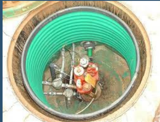
Secondary Containment Devices
