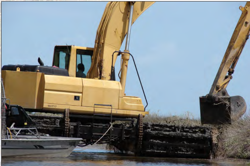
Top: An amphibious excavator with a 60 foot backhoe extension, excavated dredge material along the banks of a perimeter ditch around Rosetta Island. Bottom: Close up view of an amphibious excavator excavating dredge material at Rosetta Island.
