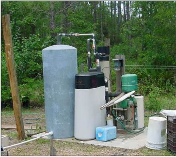
Figure 43. Private well with tank, softener, and filter.
