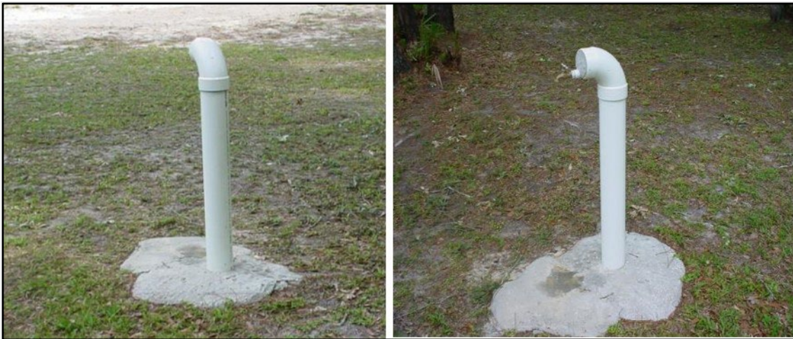
Figure 38. Is this a well? No, it is a faucet connected to a municipal water supply at a county park.
