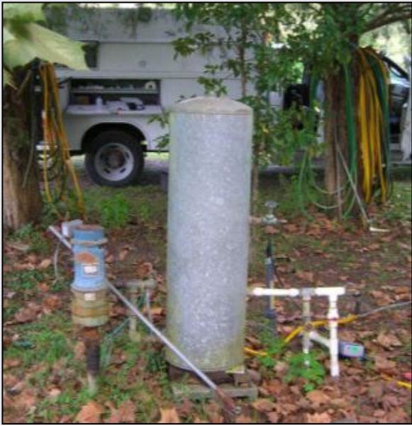
Figure 42. Private well with tank, but no softener or filter.
