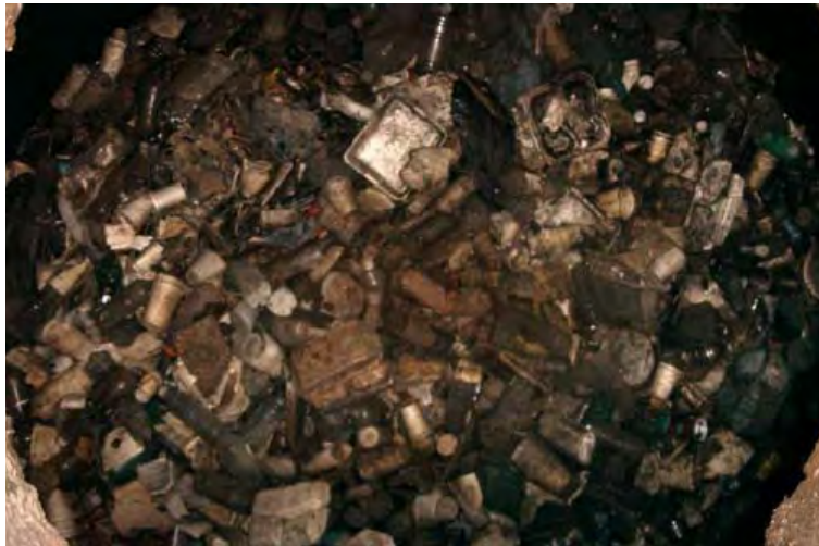
Figure 5.1 Debris within Storm Drain System in Wagner Creek (MH 276)
