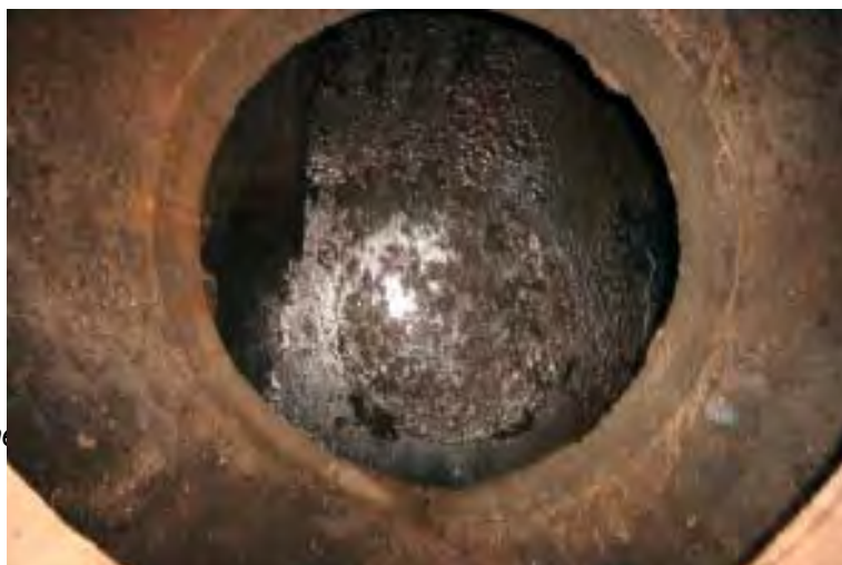
Figure 5.2 Stagnant Water With Biological Matter Accumulation in the Storm Drain System in Wagner Creek (MH 229)
